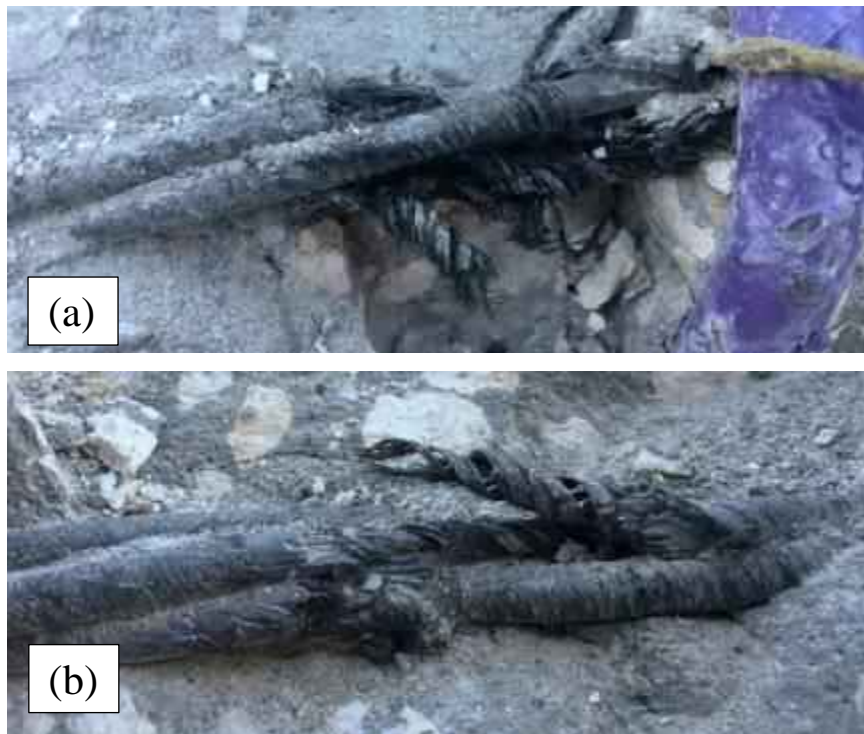
Figure 6.21: A close up view of the strand rupture after 3 months exposure (a) top beam (b) bottom beam.
