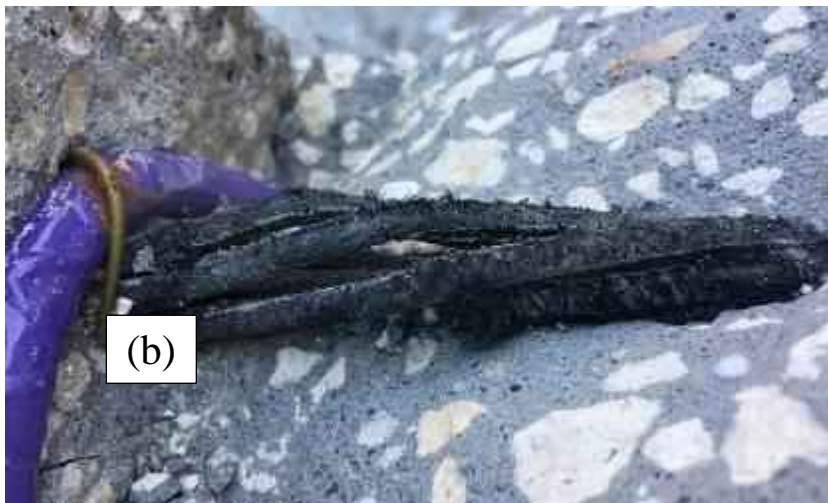
Figure 6.29: A close up view of the strand rupture after 12 months exposure (a) top beam (b) bottom beam
