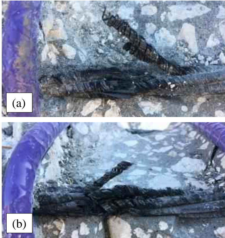
Figure 6.32: A close up view of the strand rupture after 18 months exposure (a) top beam (b) bottom beam.
