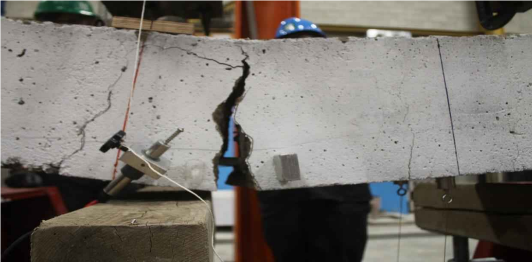
Figure 4.52: Flexural tension failure mode observed in all of the control and conditioned specimens
