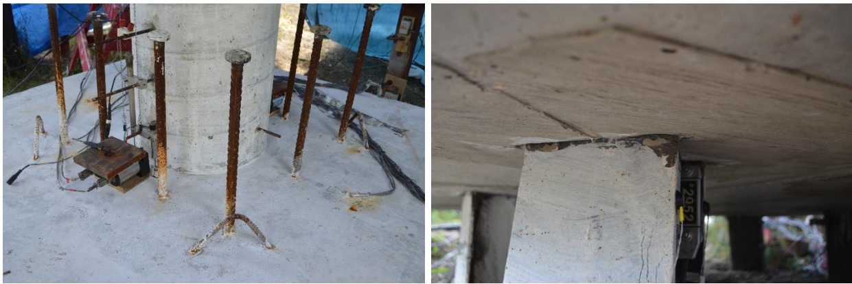
Figure 5.44. No damage on column connection (left) and pile connection at the end of Phase I, (right)
