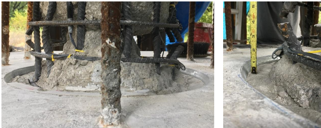
Figure 5.46. Spalling of grout closure pour at the end of Phase II
