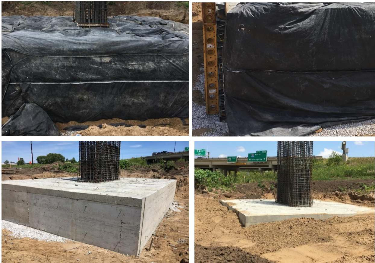
Figure 5.17. Insulation and formwork removal stage: Day 0 Insulation blanket (top left), Day 5. Formwork removed from three sides (top right), Day 10 Exposed concrete surface (bottom left), and Day 12 Footing backfilled with soil (bottom right)
