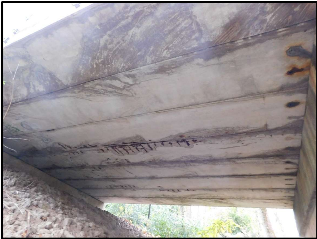
Figure 4.30 Spalling and exposed stirrups on east span.
