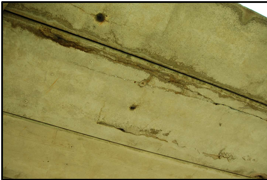
Figure 4.38 Longitudinal cracking in bottom flange near shear key (Rock Creek).
