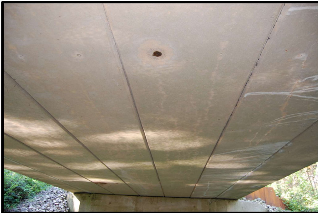
Figure 4.42 Rust staining around drain holes (Pond Creek).
