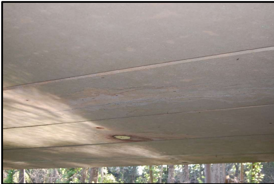
Figure 4.5 Longitudinal crack in middle beam.
