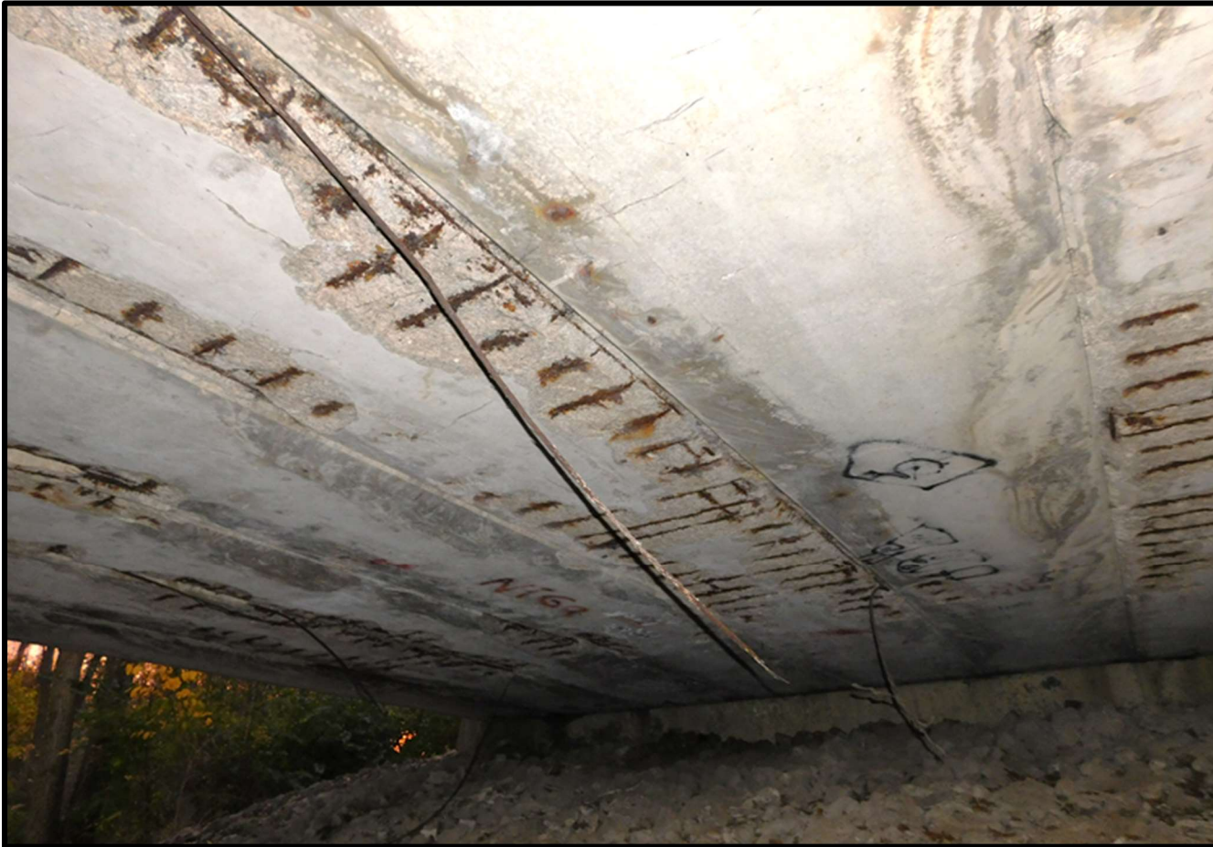
Figure 4.41 Fractured prestressing strands and corroding shear reinforcement (Main Street).
