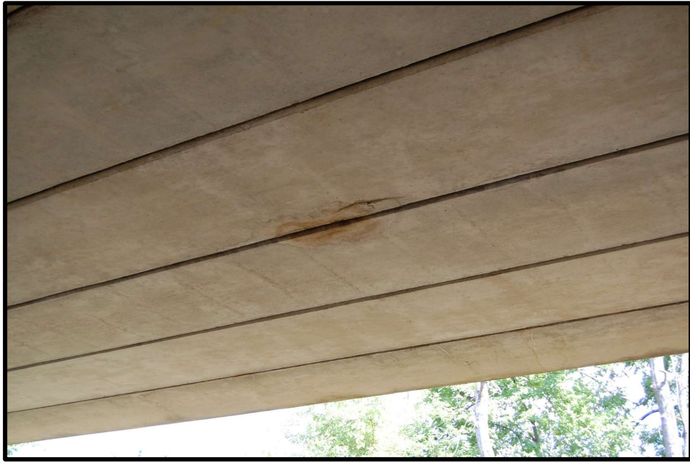
Figure 4.15 Staining near bottom of longitudinal joint.
