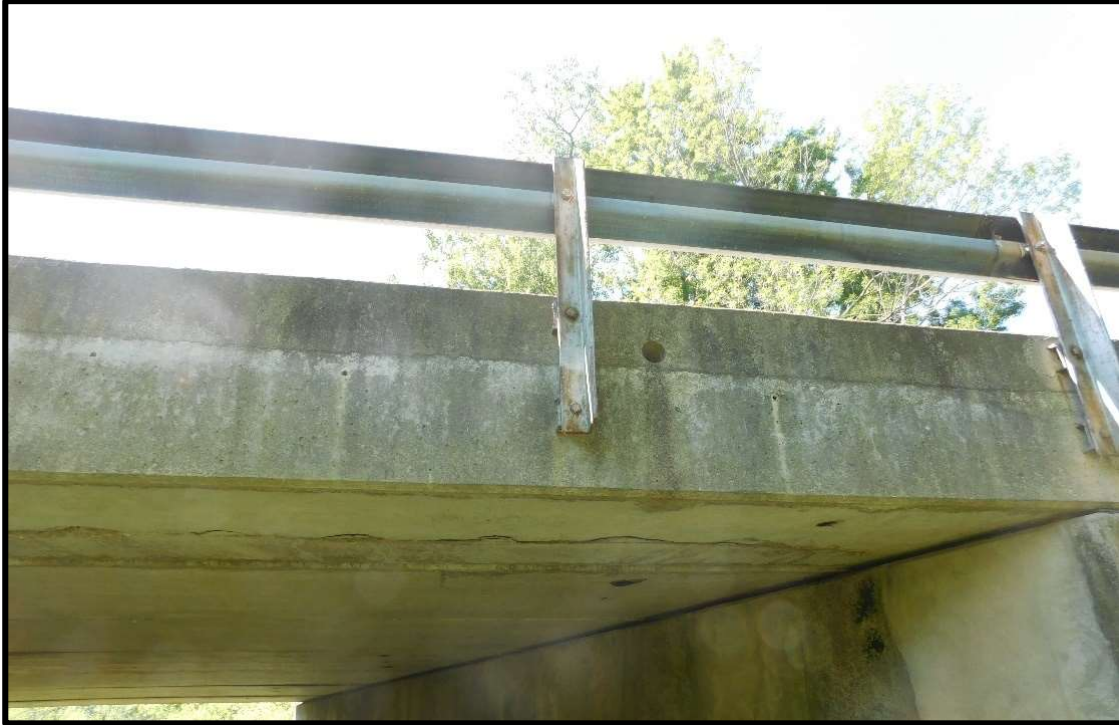
Figure 4.45 Curb cutout and efflorescence on exterior beam (Rock Creek).
