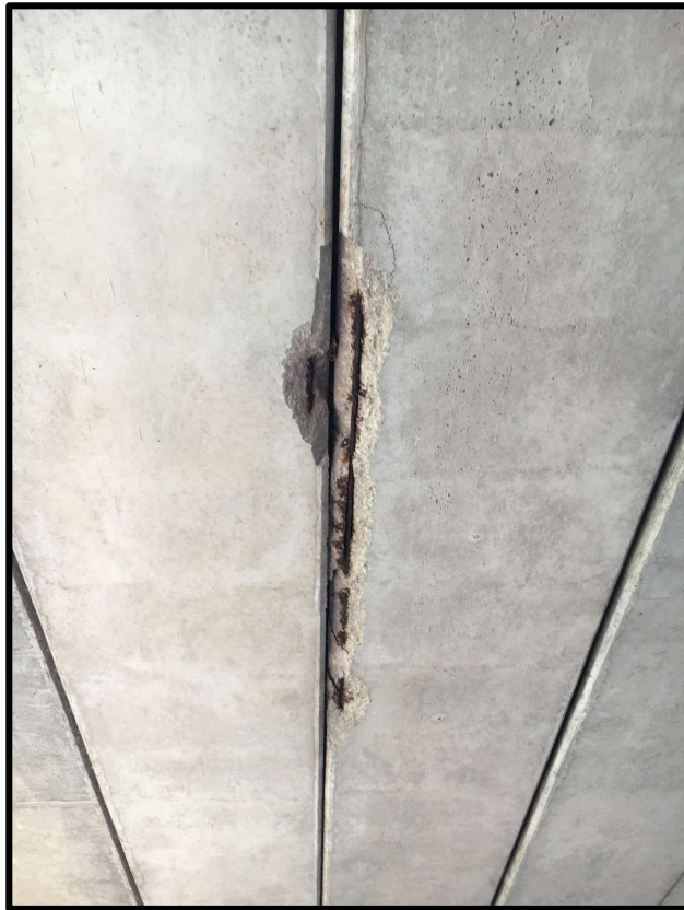
Figure 4.14 Region of spalling with two exposed strands.
