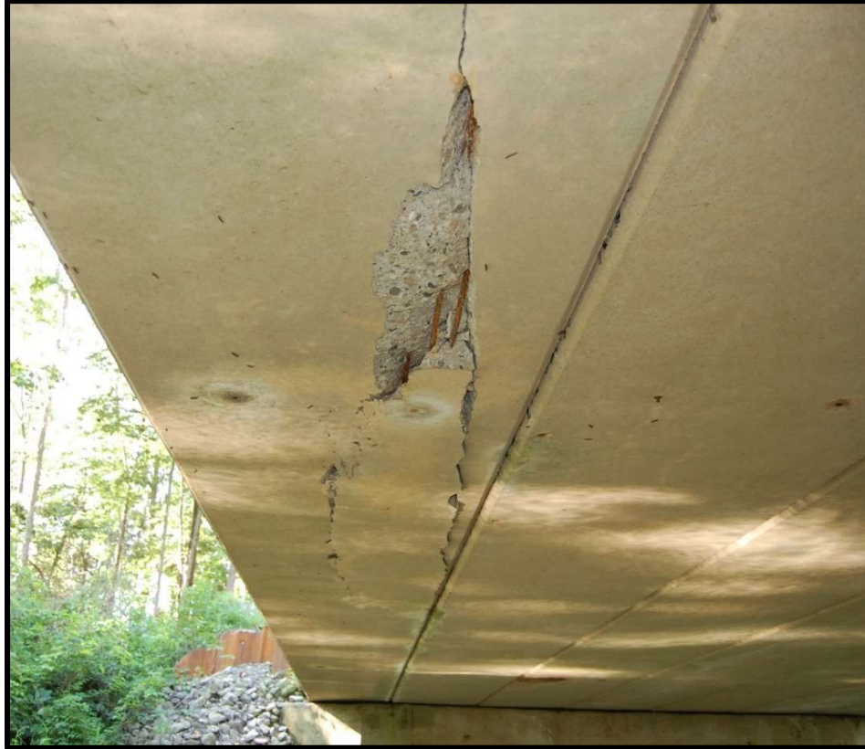
Figure 4.4 Cracking, spalling, and exposed strands in exterior beam on east end.
