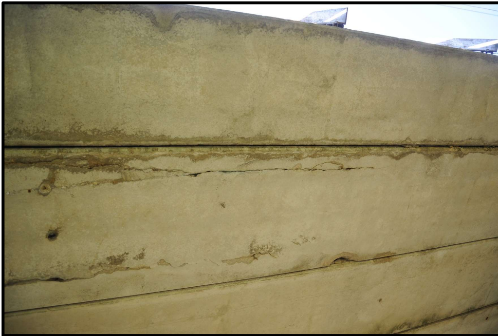
Figure 4.11 Longitudinal crack, spalling, and efflorescence in bottom flange in middle span.
