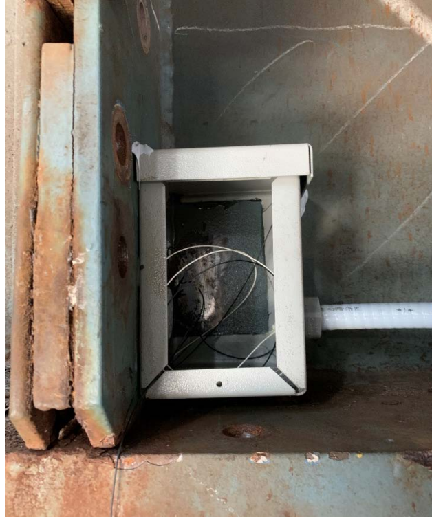
Figure 22 Sample of ruggedized and protected FBG sensor protected by NEMA enclosure box
