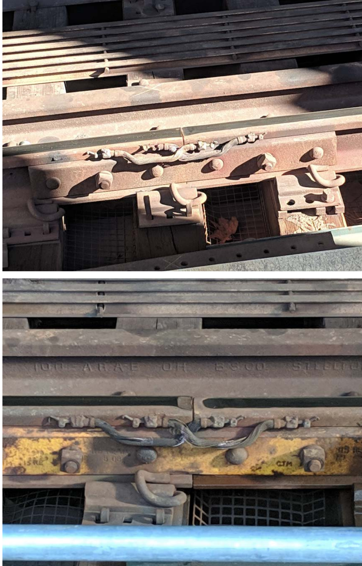
Figure 7 Problematic rail splicing joints
