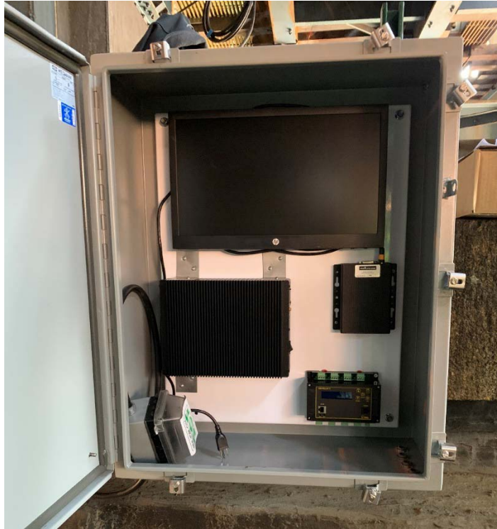
Figure 20 NEMA enclosure housing the DAQ, processor, and communication systems
