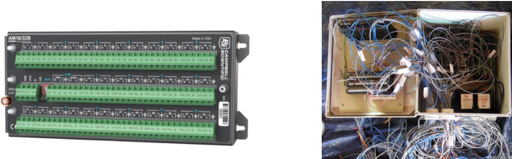
Figure 5 - Data acquisition system used for data collection
