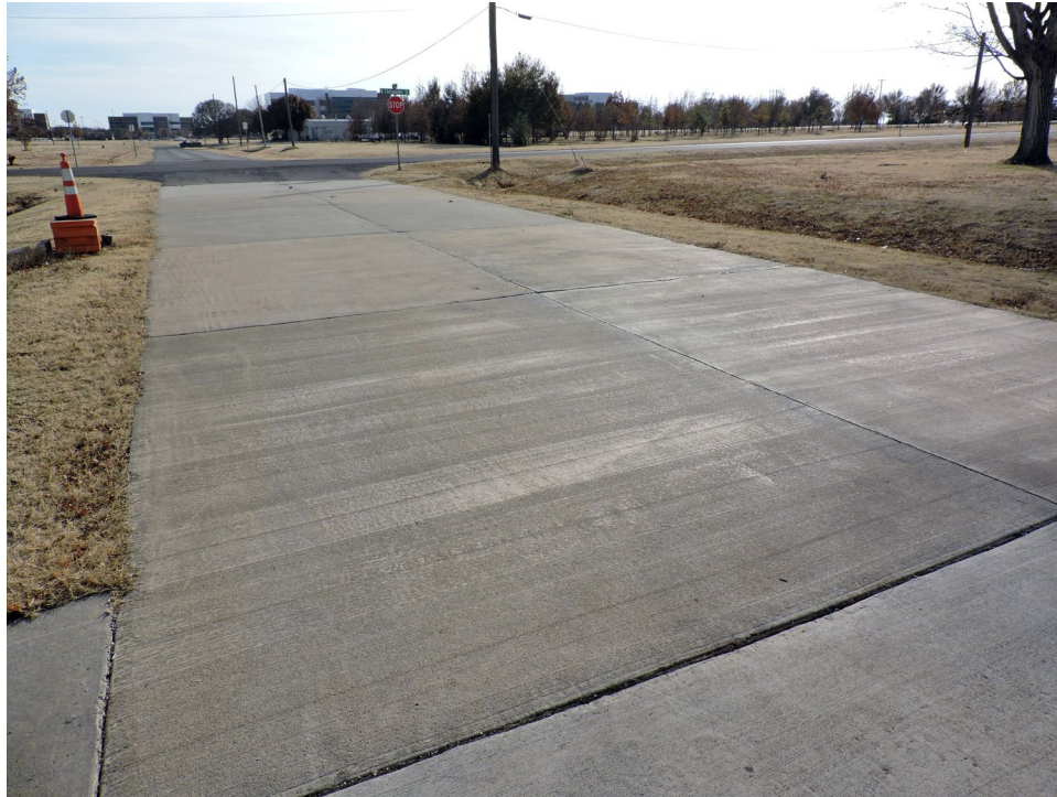
Figure 10-15. Condition of Panels 5 Through 8 After Two Years in Service
