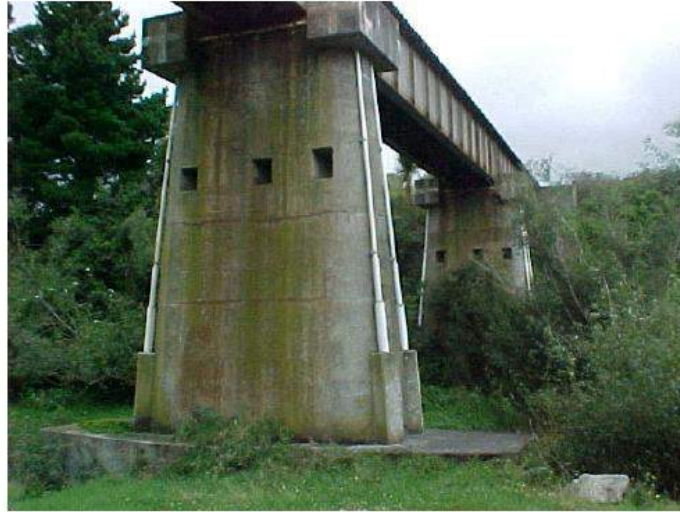
Figure 2.14 External Prestressing Retrofit at a URC Railroad Bridge Pier in New Zealand (Walsh 2002)
