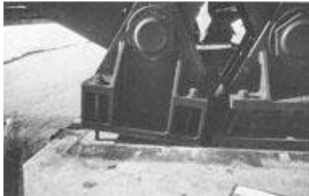
Figure 2.10 Anchorage Failure at the Bearing of a URC Pier of Bridge 14.5 after the 1964 Alaska Earthquake (McCulloch and Bonilla 1970)
