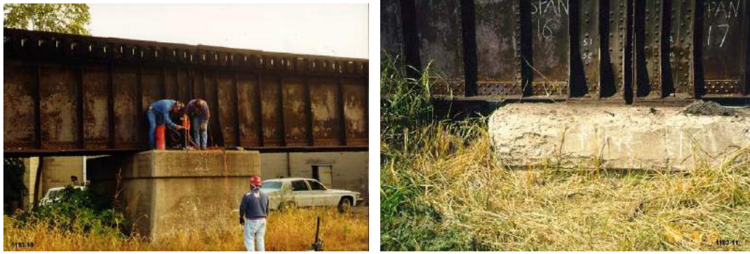
Figure 3.6 Typical Pier Condition in the Cincinnati Bridge (Uppal et al. 2000)
