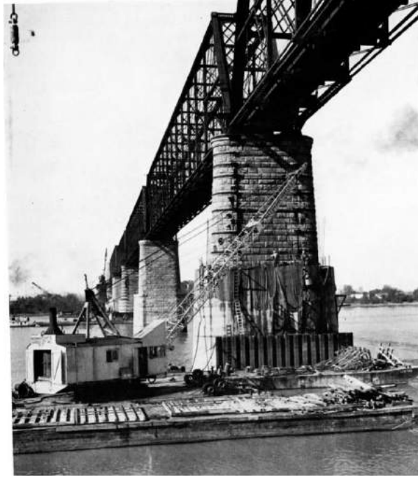
Figure 2.13 Construction of the RC Jacket Retrofitting at a URM Pier of the Illinois Central Railroad Cairo Bridge over the Ohio River (Modjeski and Masters 1953)
