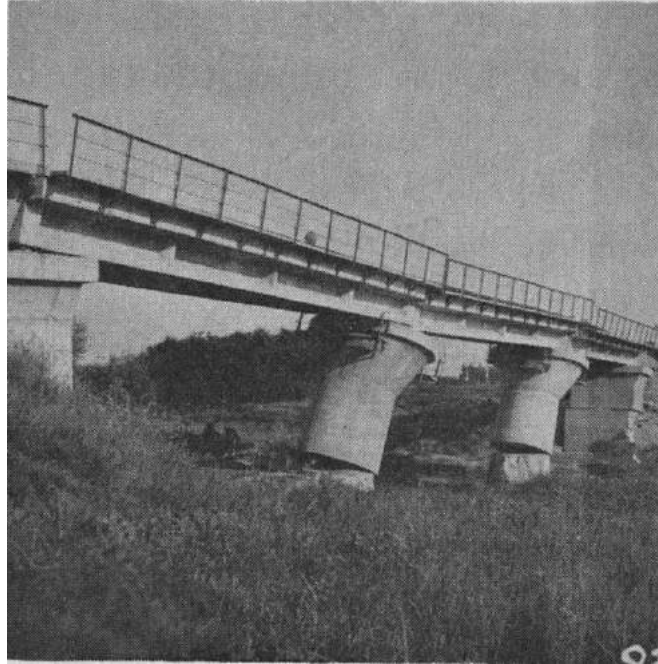
Figure 2.8 Tilting of Upper Partition of URC Piers of Dou River Railway Bridge after the 1976 Tangshan Earthquake (Chen 1978)
