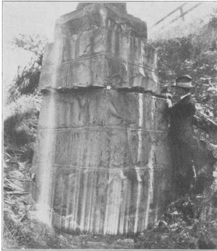
Figure 2.6 Cracking Damage of a URM Pier of Dos Pueblos Viaduct after the 1925 Santa Barbara Earthquake (Kirkbride 1927)
