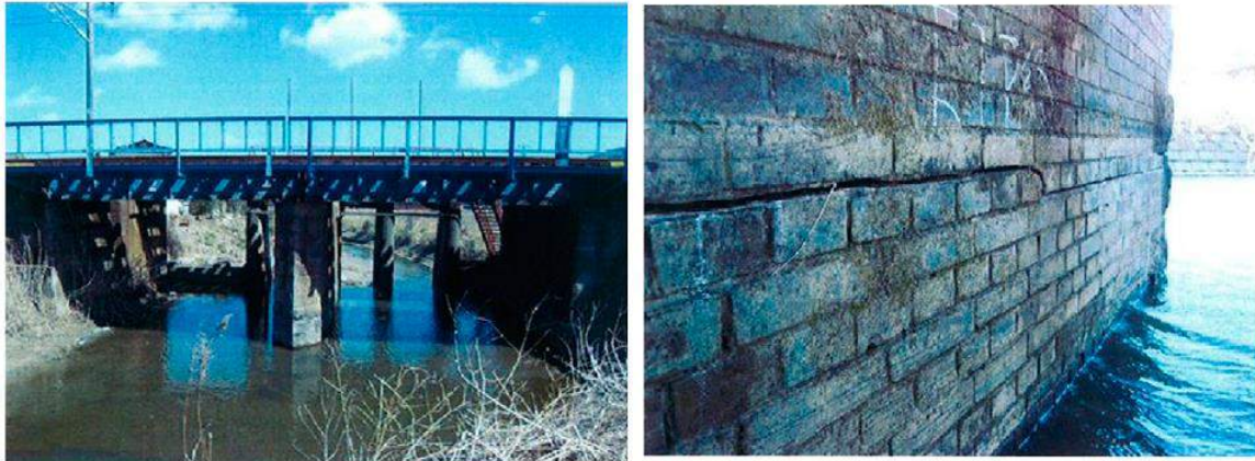
Figure 2.2 Damaged Railroad Bridge and the Crack at the Pier (Abé and Shimamura 2014)
