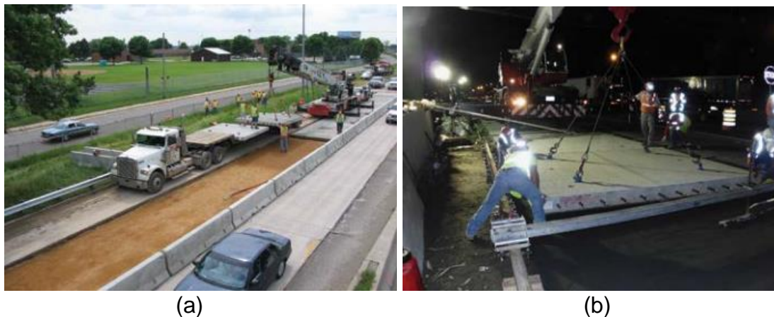
Figure 2: (a) Single lane repair using an existing lane and the shoulder, and (b) single lane closure and placement of slabs using crane (SHRP-2, 2015)
