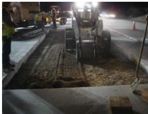
Figure 8: A skid-steer mounted milling head used to trim a cement treated base (NCPA, 2017)
