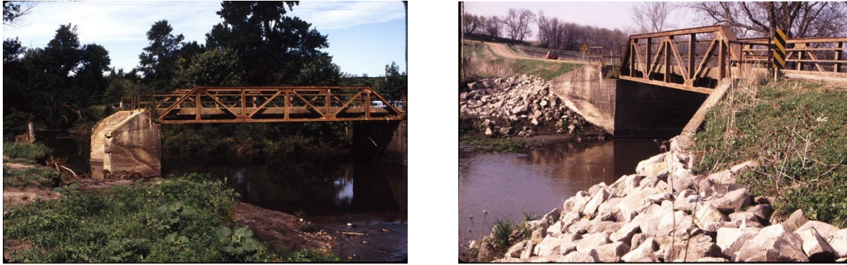
Figure 1.1 Effect of flood on erosion at a small bridge situated in Squaw Creek, close to Ames (Iowa). The left picture shows that all the erodible material behind the toe of the wing-wall abutment was washed by the flood. The right picture shows the bridge after the abutments were reconstructed and riprap stone was placed on the floodplain around the abutments
