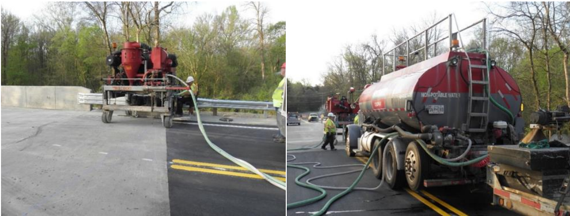
Figure 5: Grooving Machine (left) and Grooving Machine Water Storage Tank (right)
