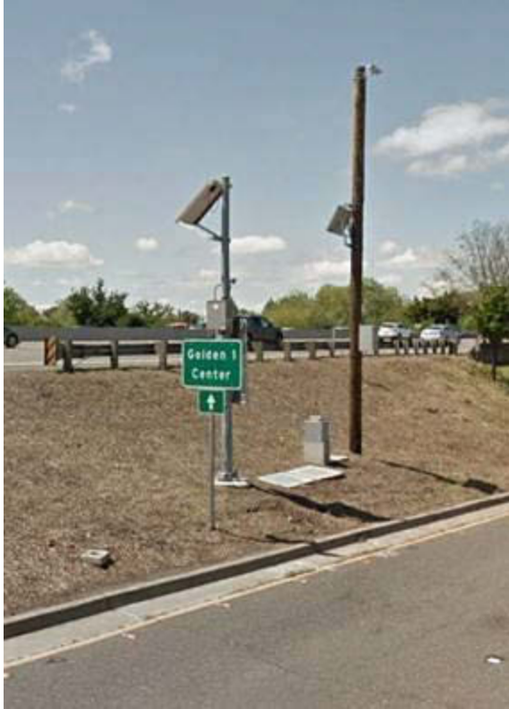
Figure 4.41: TAPCO radar sensor blocked by informational sign for the 16 th Street exit ramp system. The AHMCT VBSM can be seen behind the TAPCO system.
