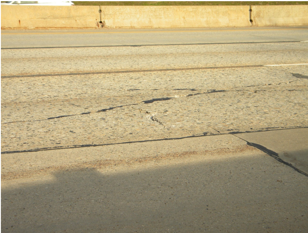
Figure 4. Shattered slabs with longitudinal and transverse cracking on I-215.
