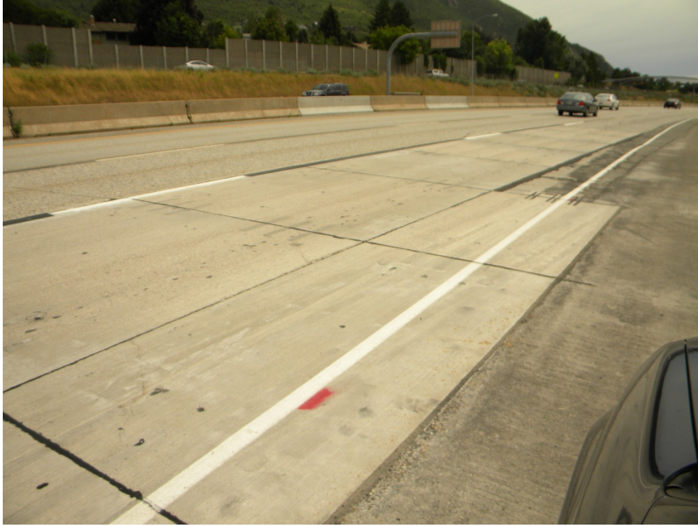
Figure 32. Placed panels and project open to traffic before diamond grinding for ride quality.
