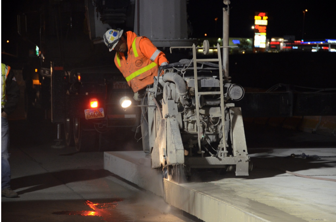
Figure 24. Cutting panels to 1- to 1.5-in taper to account for horizontal curvature of existing roadway.
