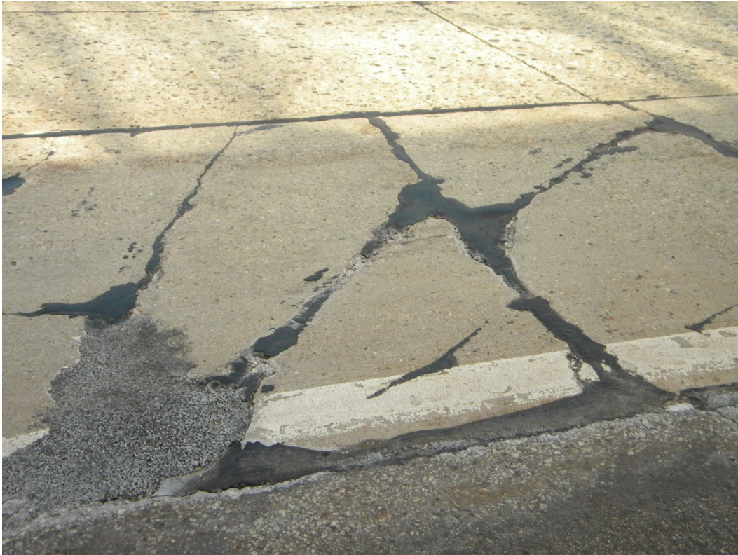
Figure 6. High-severity cracks and spalls on the on-ramp slabs on I-215.
