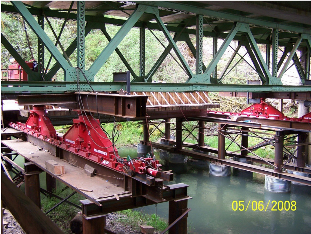
Figure 19. View of a complete hydraulic sliding system, including hydraulic jacks, hydraulic pumps, and the railing system.
