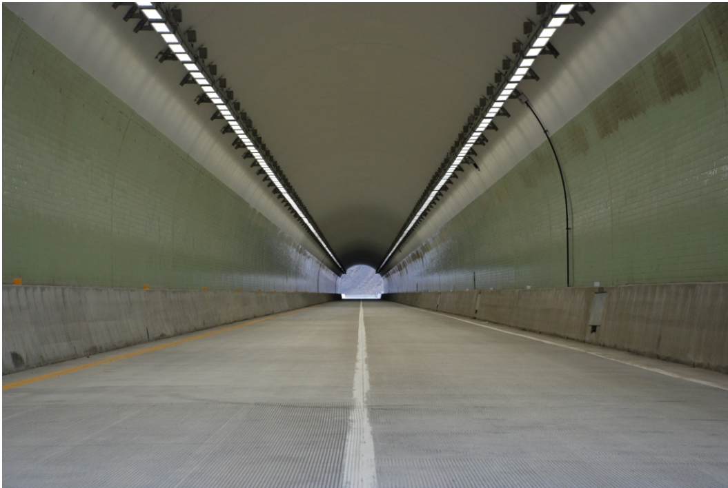
Figure 14. Photo. New LED lighting system.
