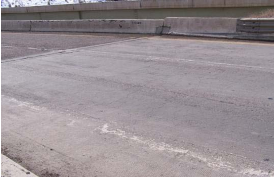
Figure 6. Photo. Existing bridge approach slab showing longitudinal and map cracking.
