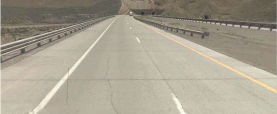
Figure 4. Photo. Rigid pavement in the vicinity of the Carlin Tunnels showing visible cracks on the surface.
