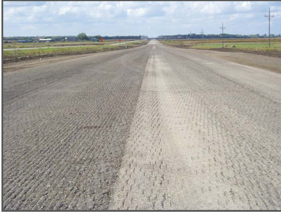
Figure 4. Rough-milled surface of the original HMA pavement.
