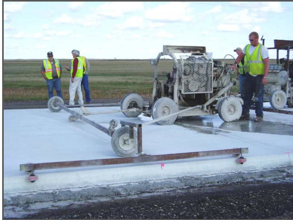
Figure 14. During the showcase, participants gathered by the paver to discuss the project and sawcutting operations.
