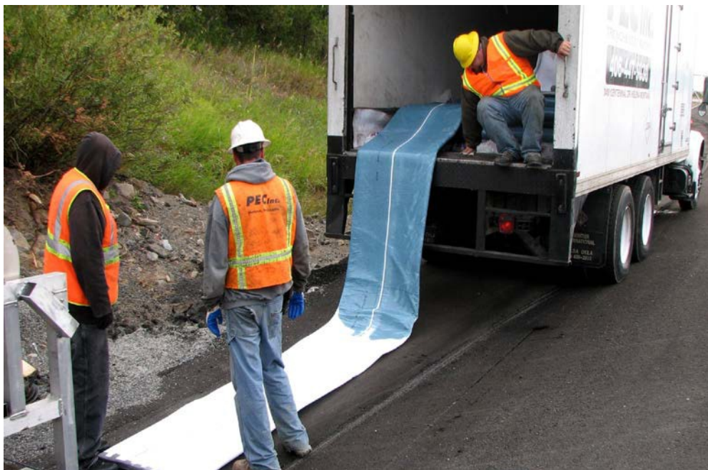
Figure 11. View of the refrigerated truck and the liner.
