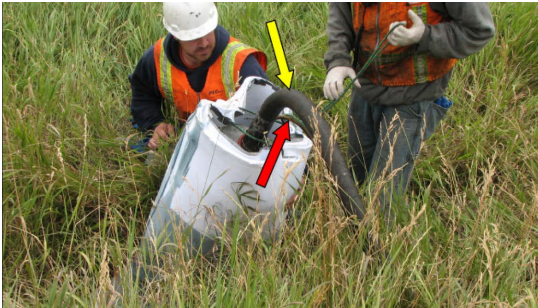
Figure 18. View of the rubber plug with air and steam line connections.
