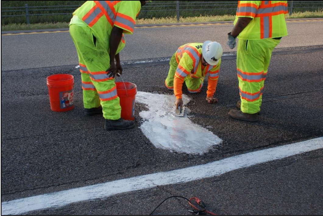
Figure 17. Photo. Workers fill distressed area with epoxy material prior to HFST application.
