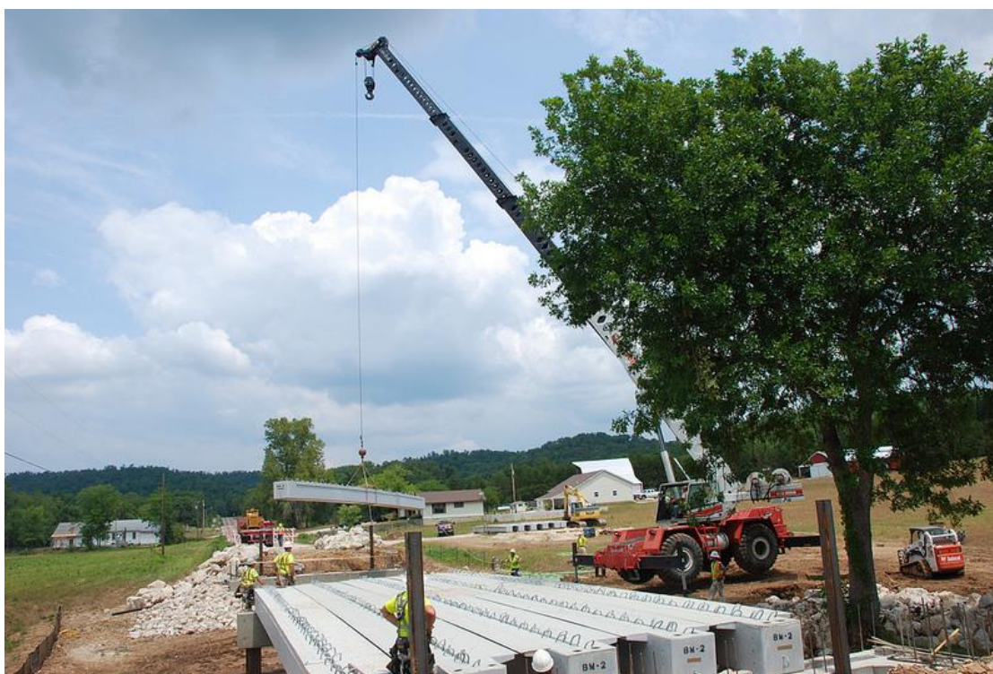
Figure 32. Begin beam placement on second span at Reynolds County site. (Photo courtesy of MoDOT)
