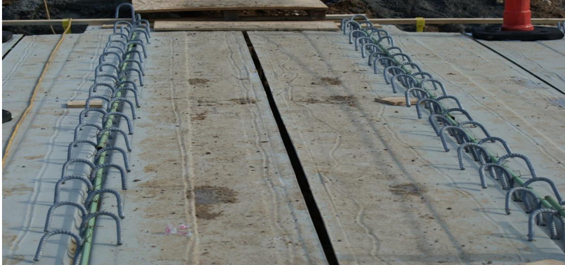
Figure 35. Gap between beam flanges.
