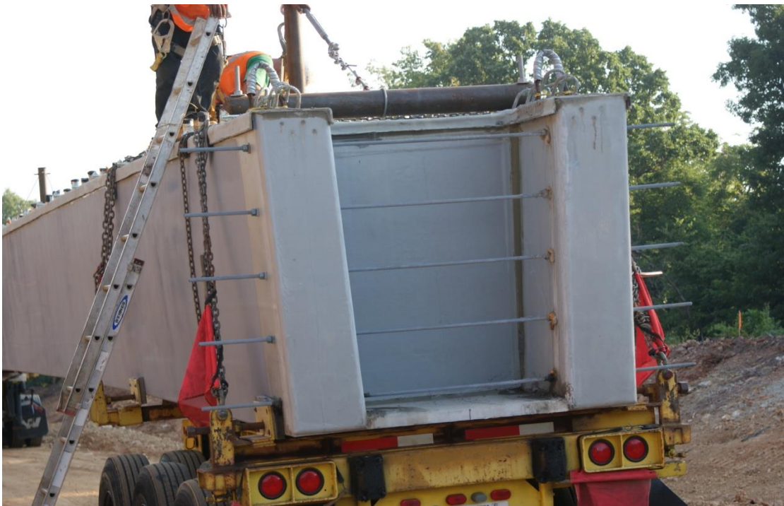
Figure 43. Beams are prepared for lifting into place. Note pipe bolted into place to accommodate lifting straps.
