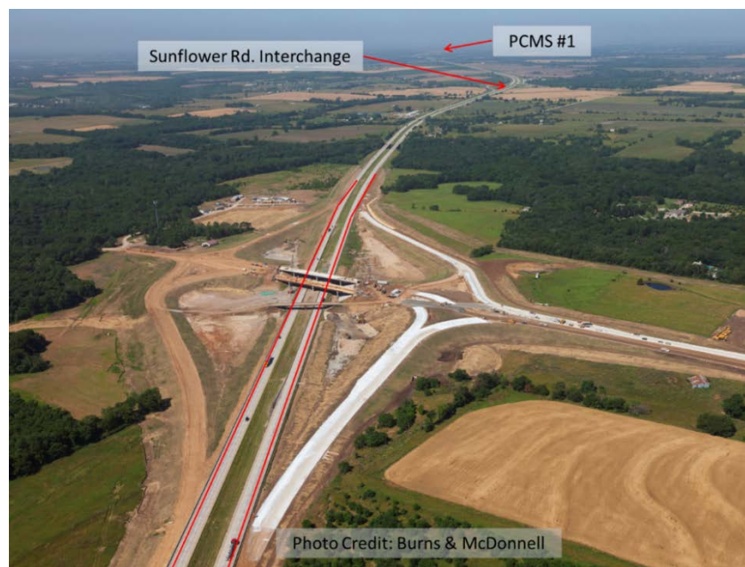
Figure 2. Photo. First portable changeable message sign location. (courtesy: KDOT)
