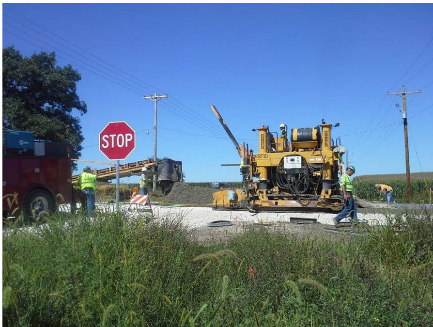
Figure 11. Photo. Placement of concrete at 1600E intersection. (courtesy: Knox County Highway Department)
