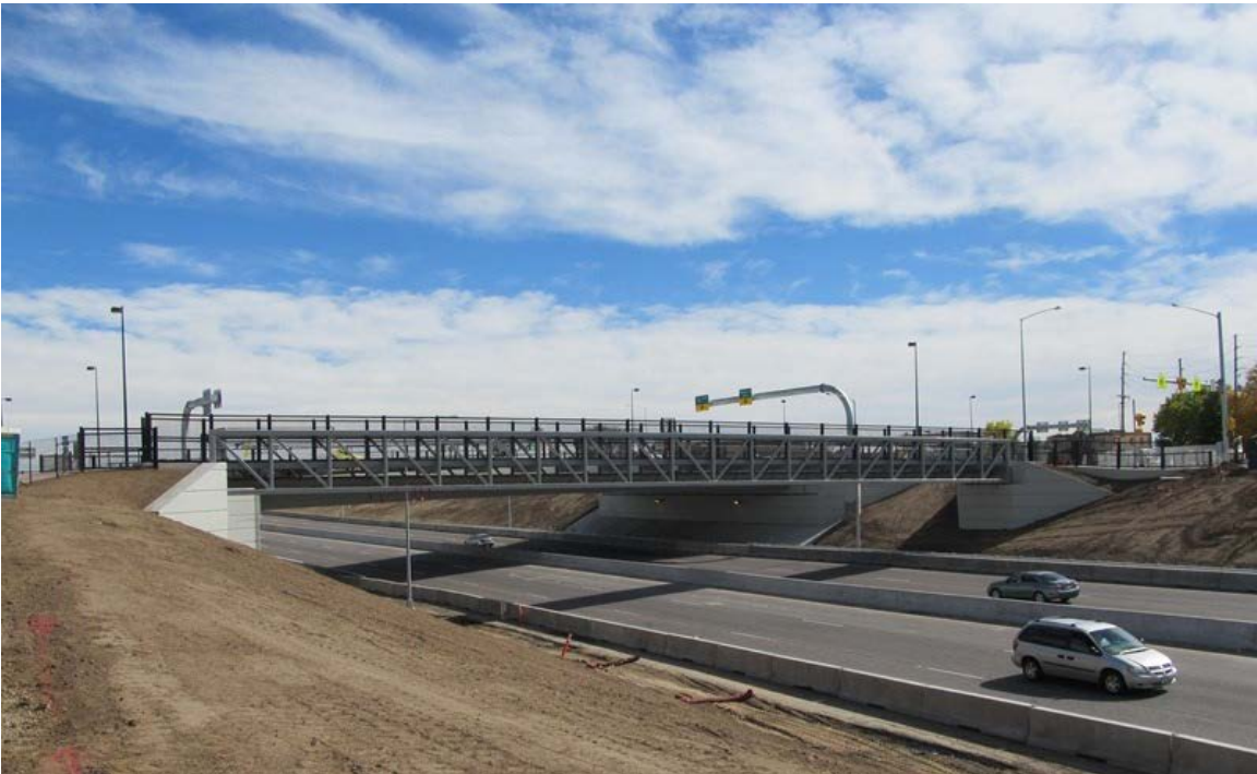
Figure 34. Photo. Completed pedestrian bridge on west side of Pecos Street Bridge (courtesy: Colorado DOT).
