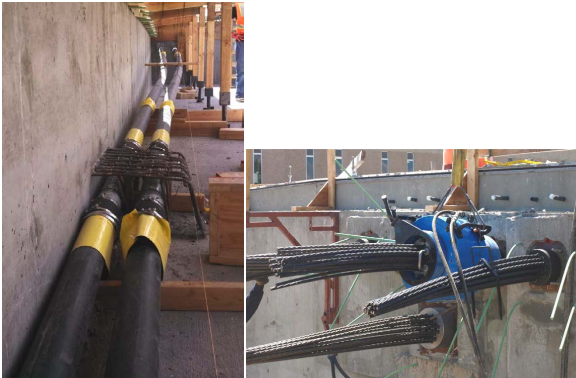
Figure 18. Photos. Longitudinal external tendons (courtesy: Colorado DOT).
