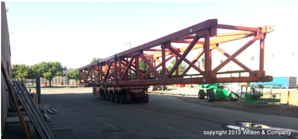
Figure 25. Photo. Frame used to connect equipment under lifting diaphragms (courtesy: Colorado DOT).
