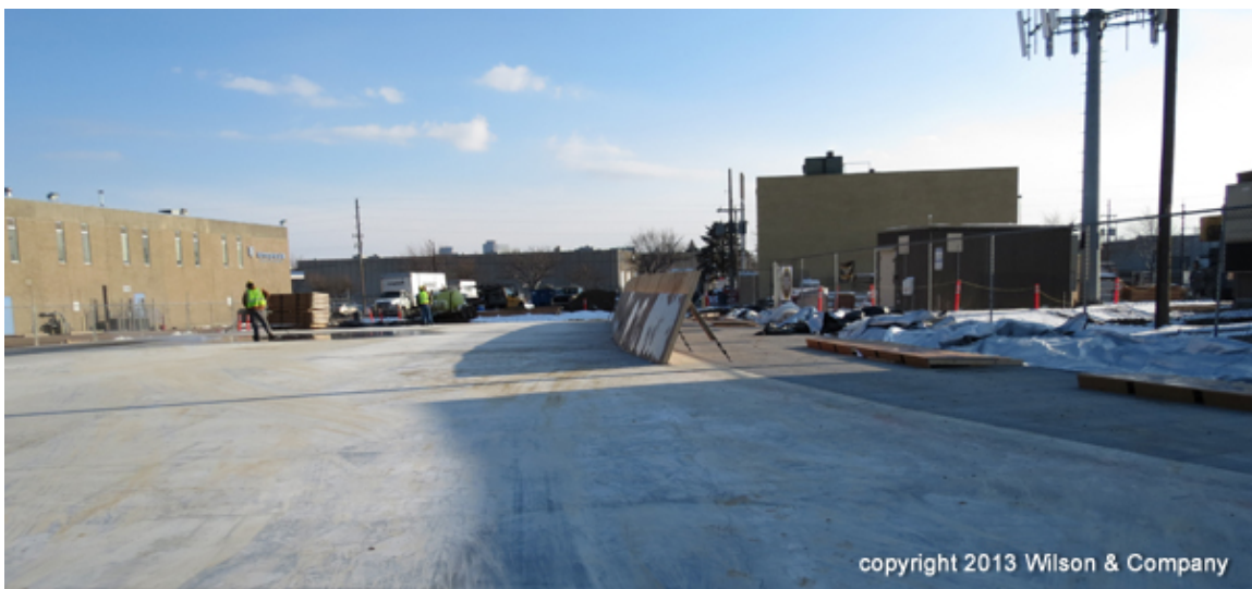
Figure 12. Photo. Close-up of completed “rat slab” or base slab construction (courtesy: Colorado DOT).
