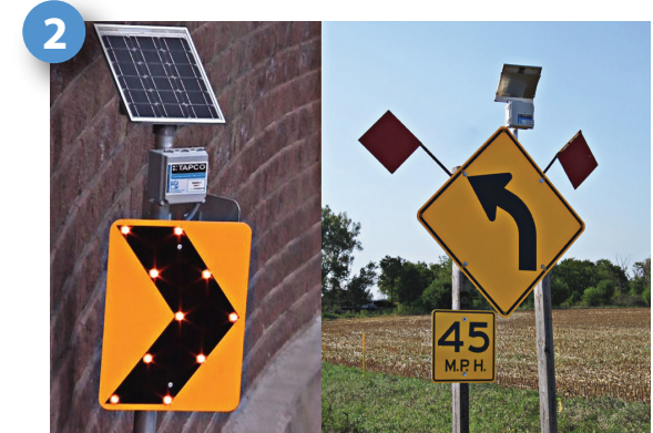
2 Approaching vehicles, sensed by a radar in the advanced curve warning sign, trigger the controller that wirelessly activates the LED signs to flash sequentially through the curves to warn speeding drivers to slow down.
