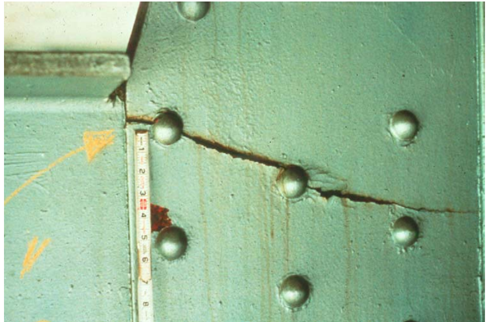
Figure 2.3.7 Fatigue Crack at Coped Top Flange of Riveted Connection
