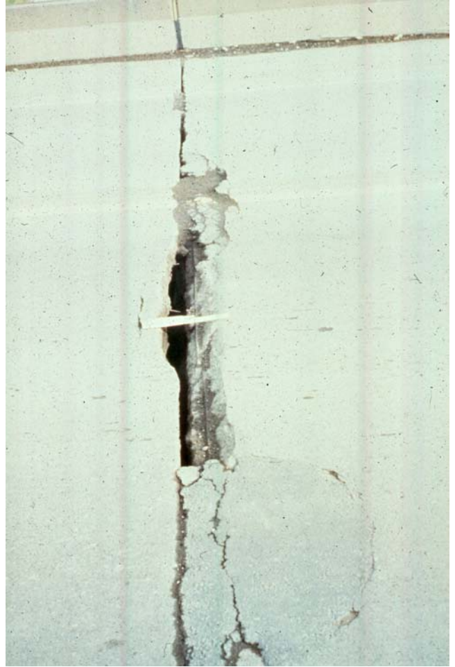
Figure 5.4.18 Failed Compression Seal
