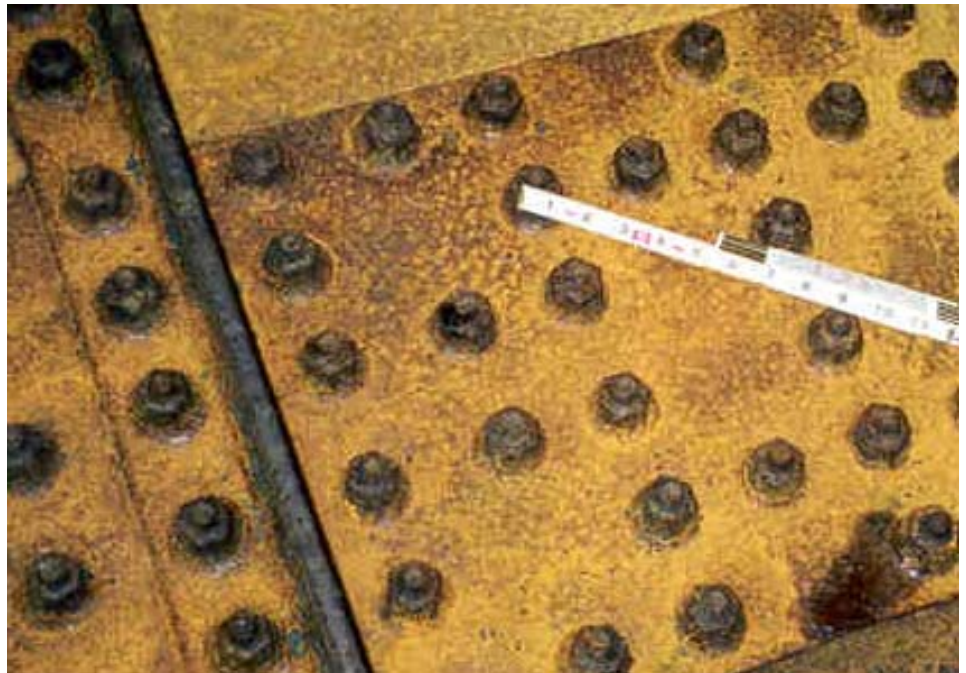
Figure 2.3.23 Yellow Orange – Early Stage of Exposure or Active Corrosion
