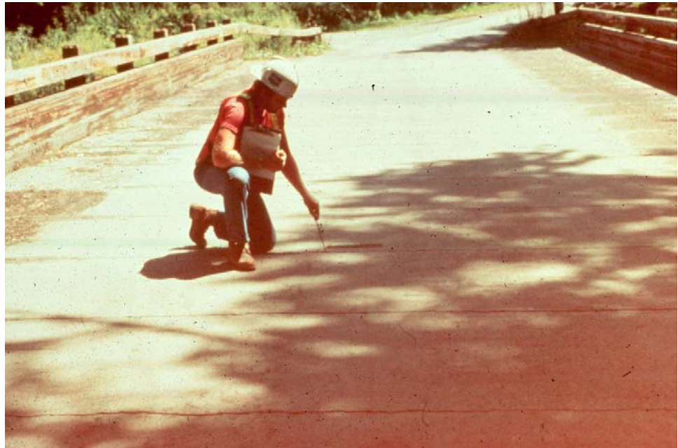
Figure 5.1.7 Inspector Probing Timber with an Ice Pick at Reflective Cracks in the Asphalt Wearing Surface
