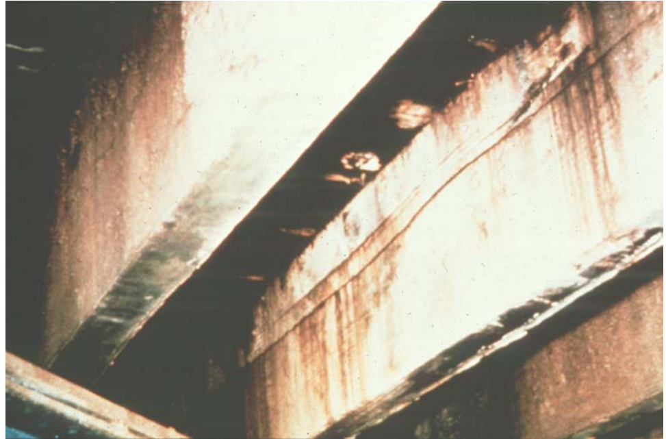
Figure 6.1.12 Horizontal Shear Crack in a Timber Beam
