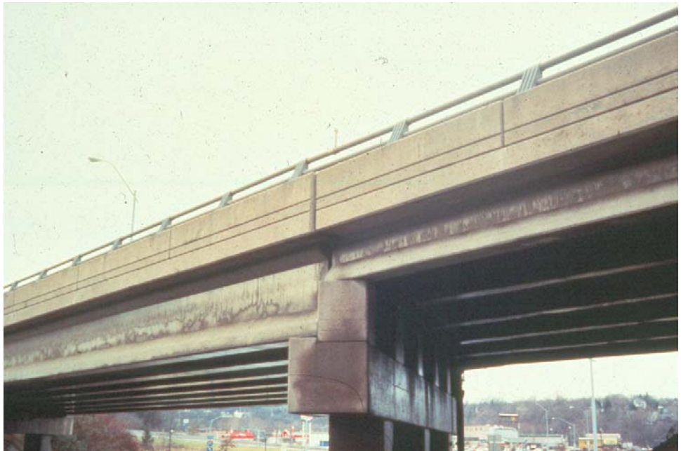
Figure 7.9.12 Leakage of Water at Inlet
