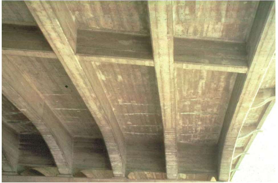
Figure 7.2.14 Flexure Cracks in Tee Beam Slab
