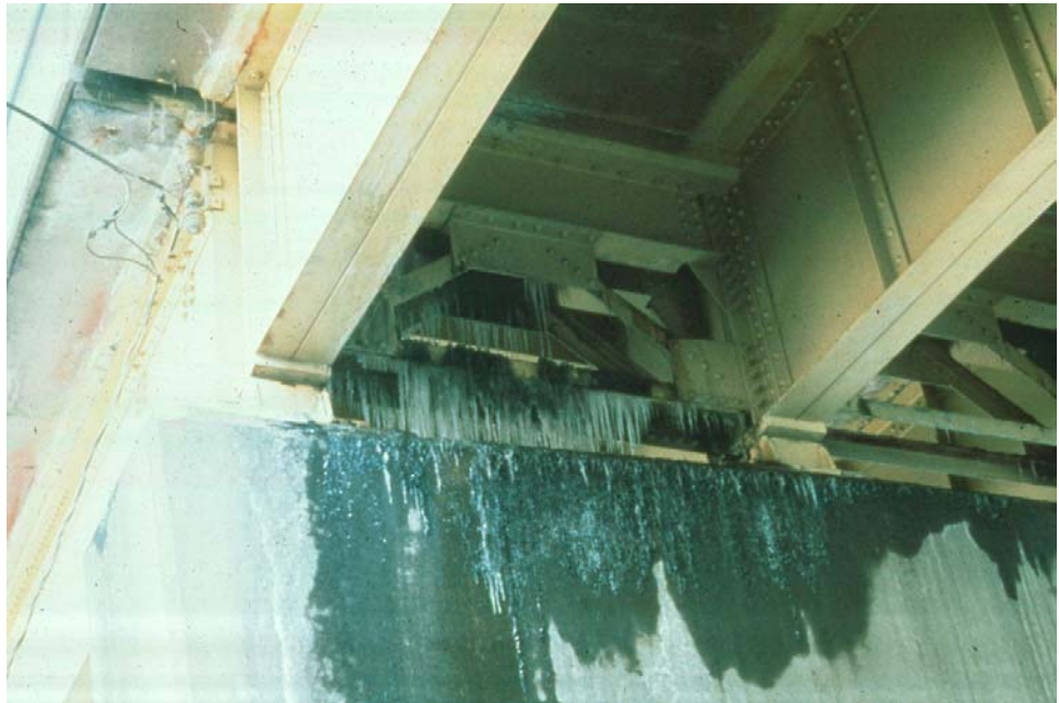
Figure 2.3.19 Water and Salt Runoff Under Expansion Dam Deck Opening
