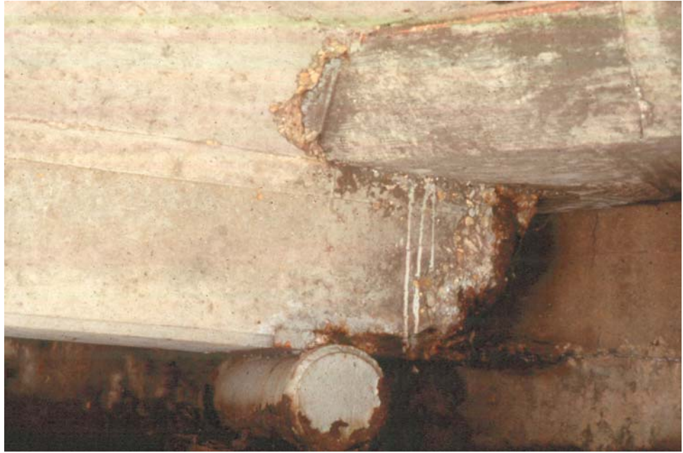
Figure 7.2.9 Spalled Tee Beam End
