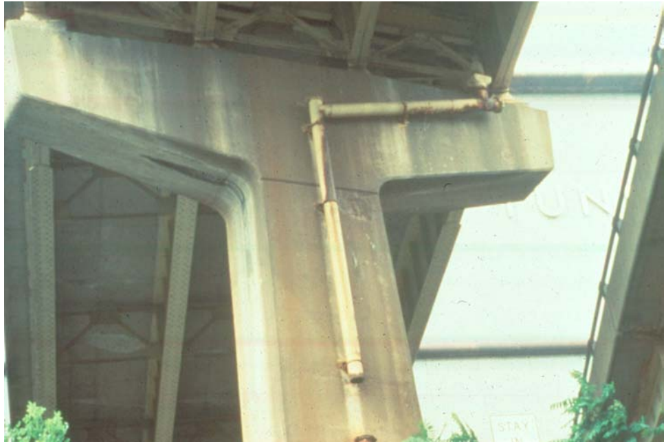
Figure 5.4.14 Downspout Pipe and Cleanout Plug
