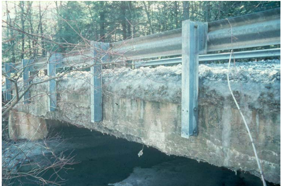
Figure 7.1.8 Deteriorated Slab Fascia due to Roadway Deicing Agents
