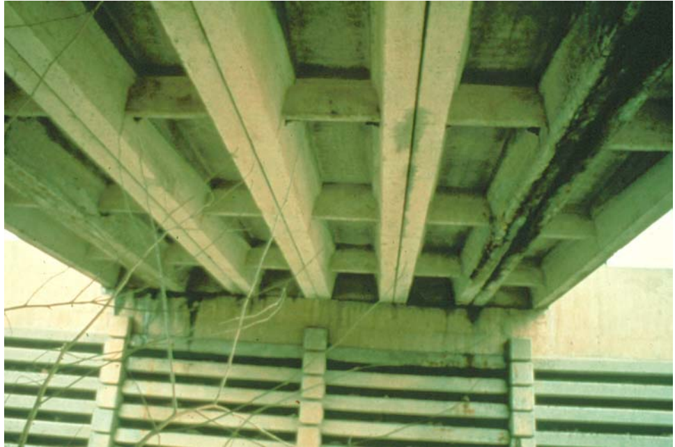
Figure 7.4.7 Joint Leakage Between Channel Beams
