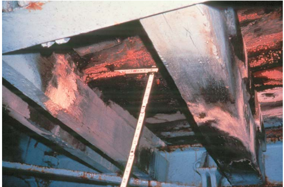
Figure 6.1.13 Decay in a Timber Beam
