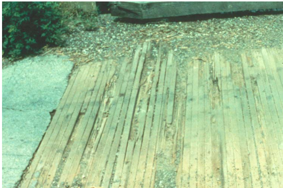
Figure 2.1.20 Abrasion Damage on a Timber Deck
