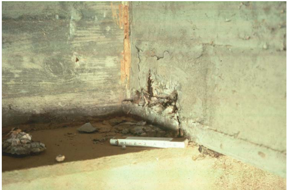
Figure 7.2.10 Deteriorated Tee Beam Bearing Area
