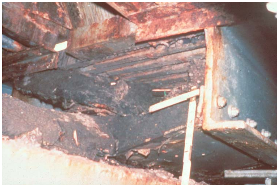
Figure 5.4.22 Drainage Trough with Debris Accumulation
