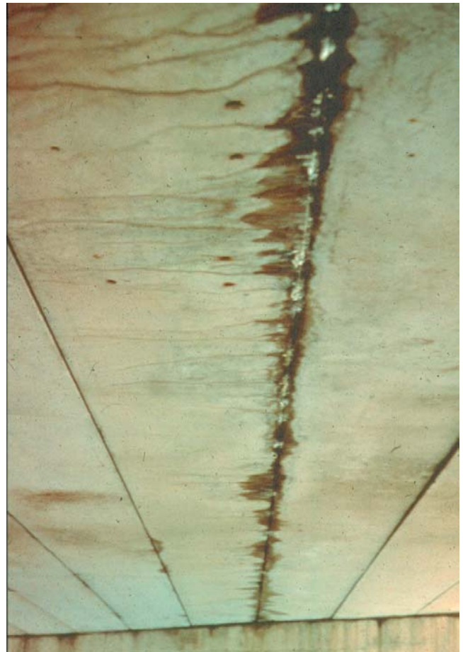
Figure 7.7.4 Leaking Joint between Adjacent Slab Units
