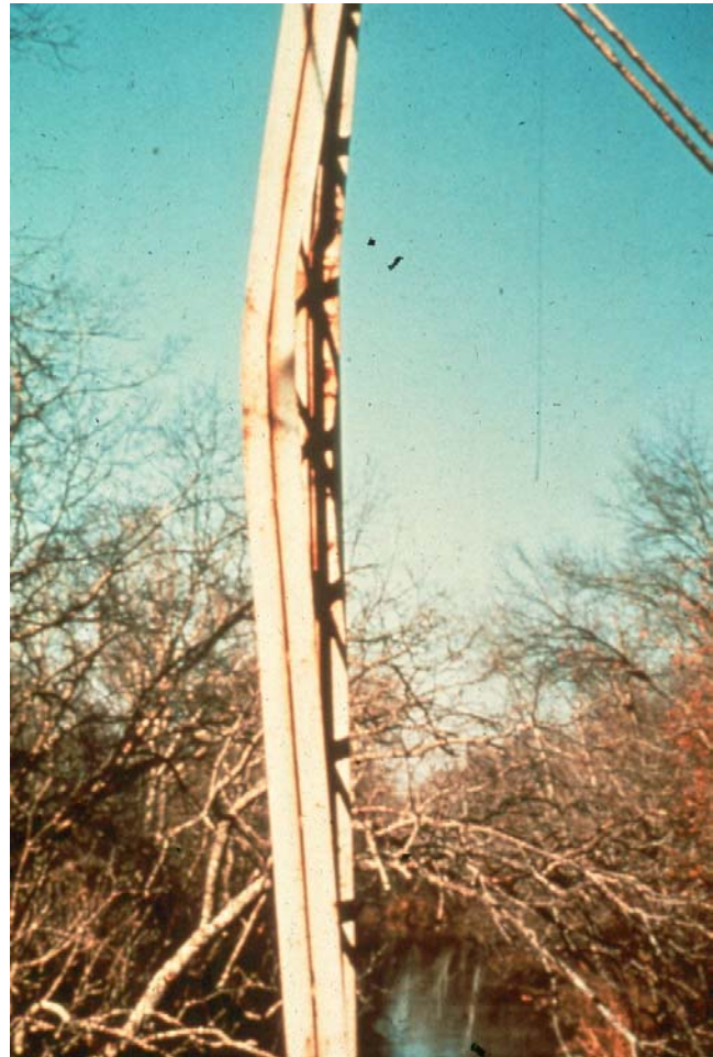
Figure 2.3.9 Collision Damage on a Steel Bridge
