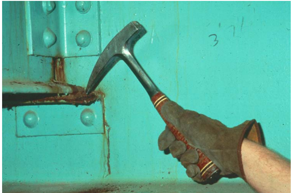
Figure 2.3.16 Corrosion of Steel
