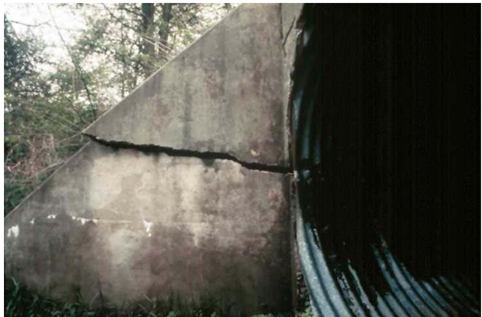
Figure P.3.23 Cracking of Culvert Due to Foundation Settlement
