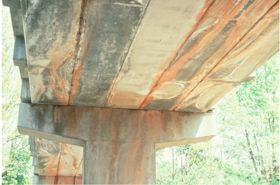
Figure 7.10.15 Joint Leakage and Rust Stain
