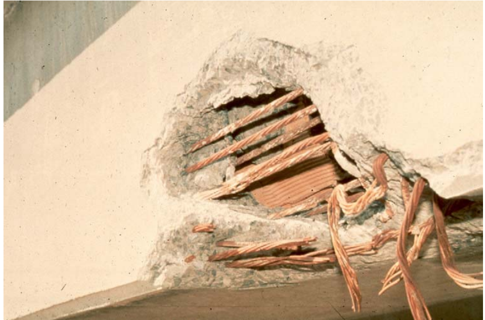
Figure 7.10.16 Close-up of Collision Damage
