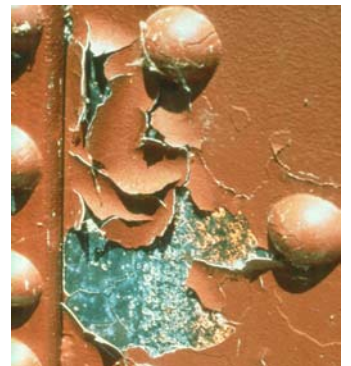
Figure 2.3.14 Paint Peeling from Steel Bridge Members
