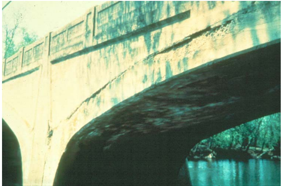
Figure 7.5.15 Deteriorated Arch/Spandrel Wall Interface
