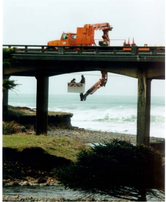
Figure 3.5.16 Underbridge Inspection Vehicle
