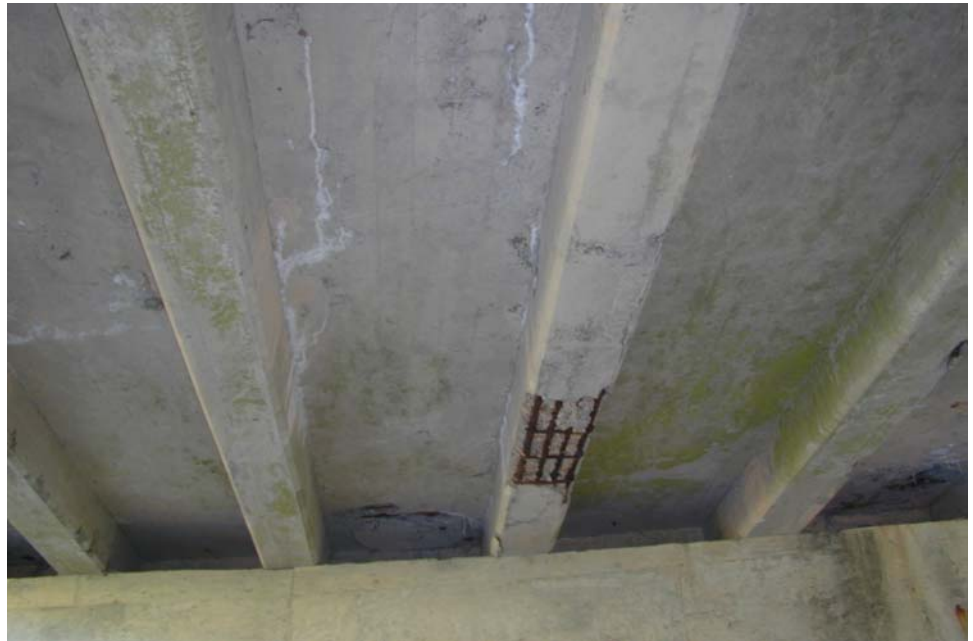
Figure 5.2.7 Underside View of Longitudinal Deck Crack
