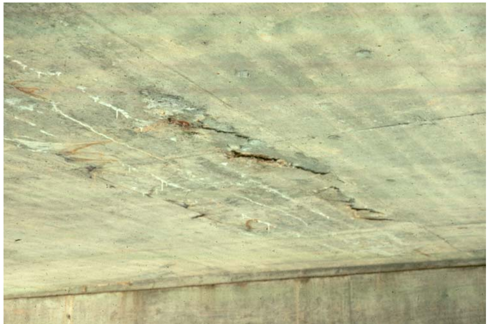
Figure 7.1.7 Delamination and Efflorescence with Rust. Stains on Slab Underside in Tension Zone
