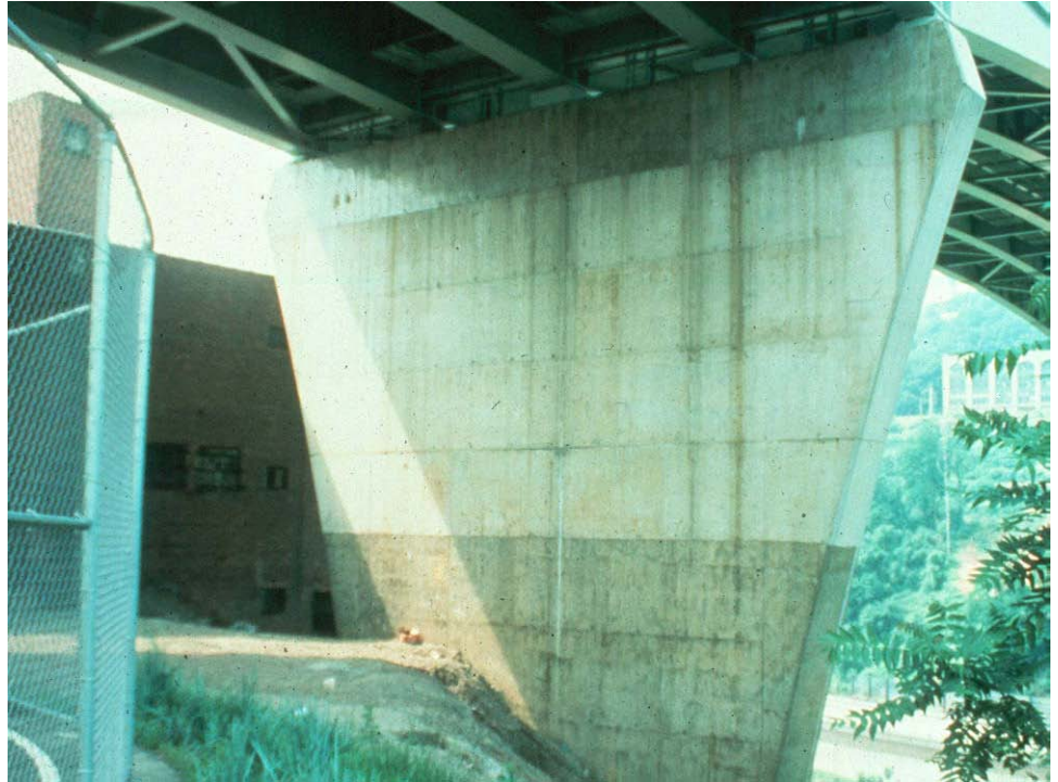
Figure 2.2.27 Anti-Graffiti Coating on Lower Area of Bridge Piers
