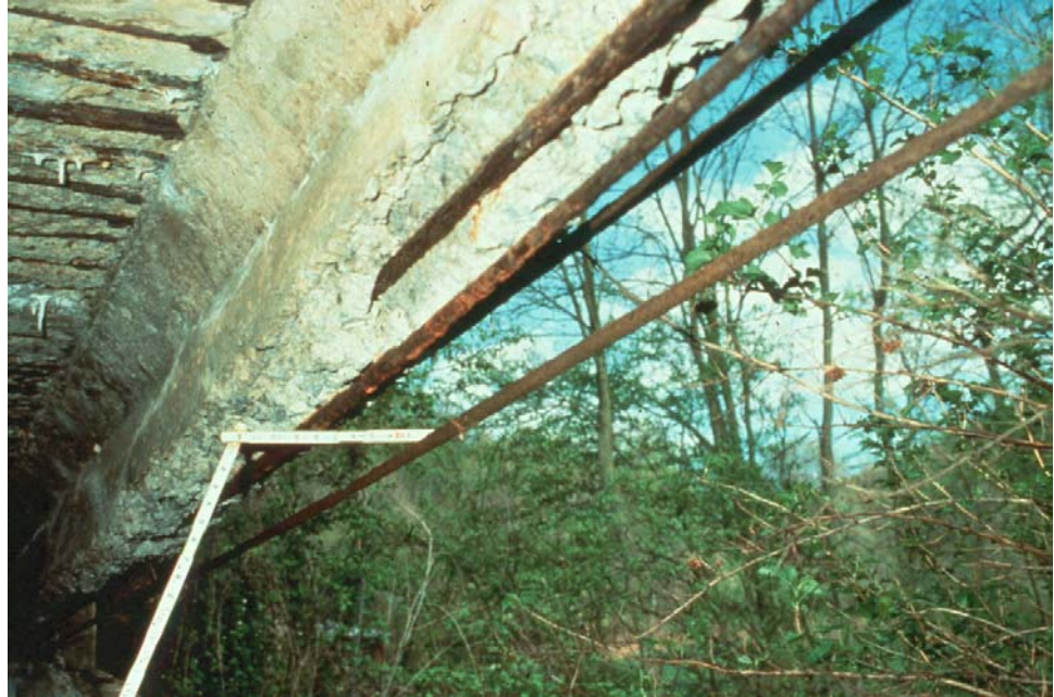
Figure 2.2.25 Corroded Reinforcing Bar
