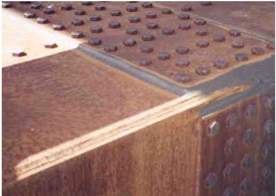
Figure 2.3.24 Light Brown – Early Stage of Exposure
