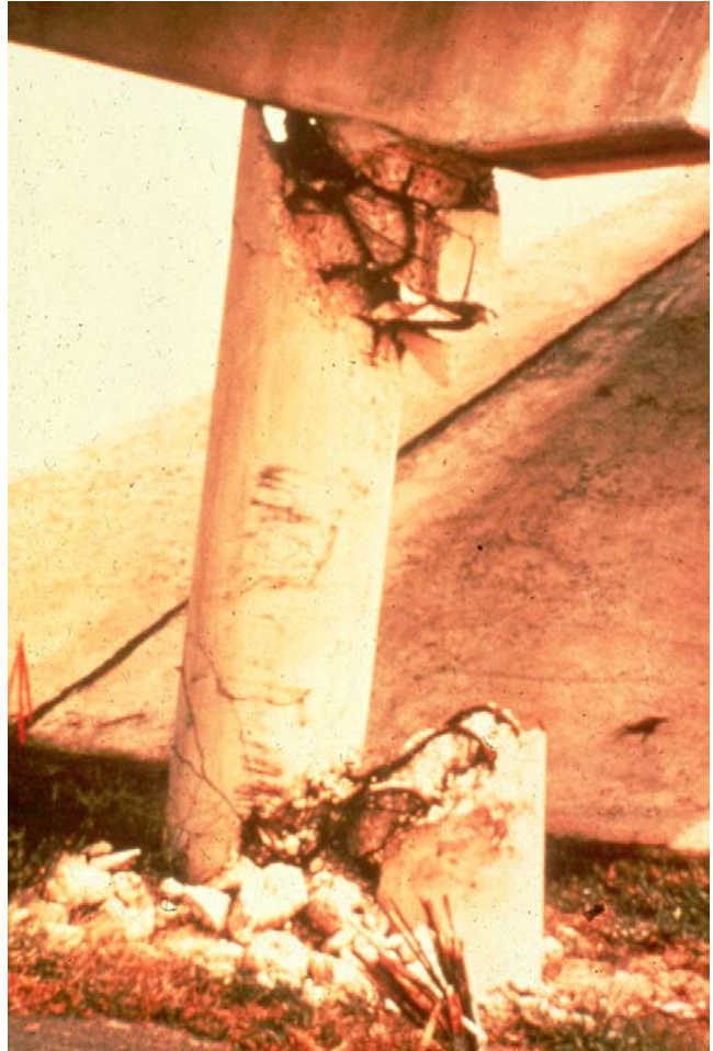
Figure 2.2.23 Concrete Column Collision Damage
