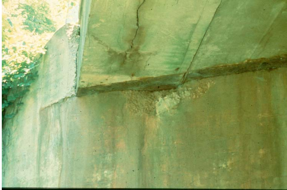
Figure 7.10.13 Longitudinal Cracks in Bottom Flange at Beam
