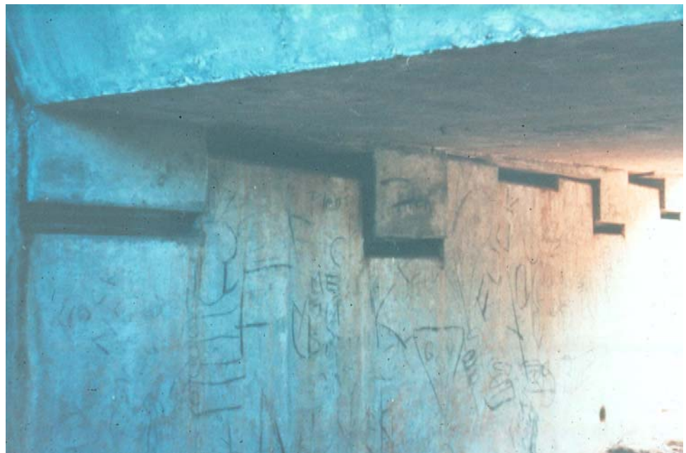
Figure 7.11.26 Shear Crack Location Near an Abutment
