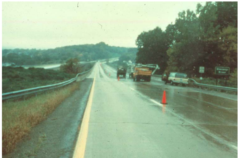
Figure 3.2.8 Inclement Weather Causing Slippery Bridge Members
