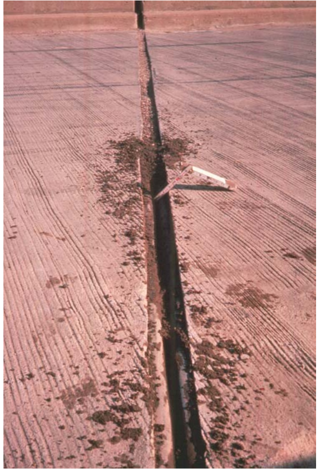
Figure 5.4.16 Dirt in a Compression Seal Joint
