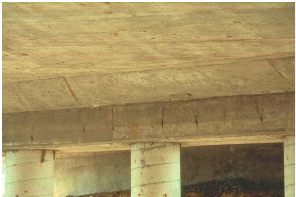
Figure 7.1.6 Shear Zone on the Underside of a Continuous Slab Bridge Near a Pier
