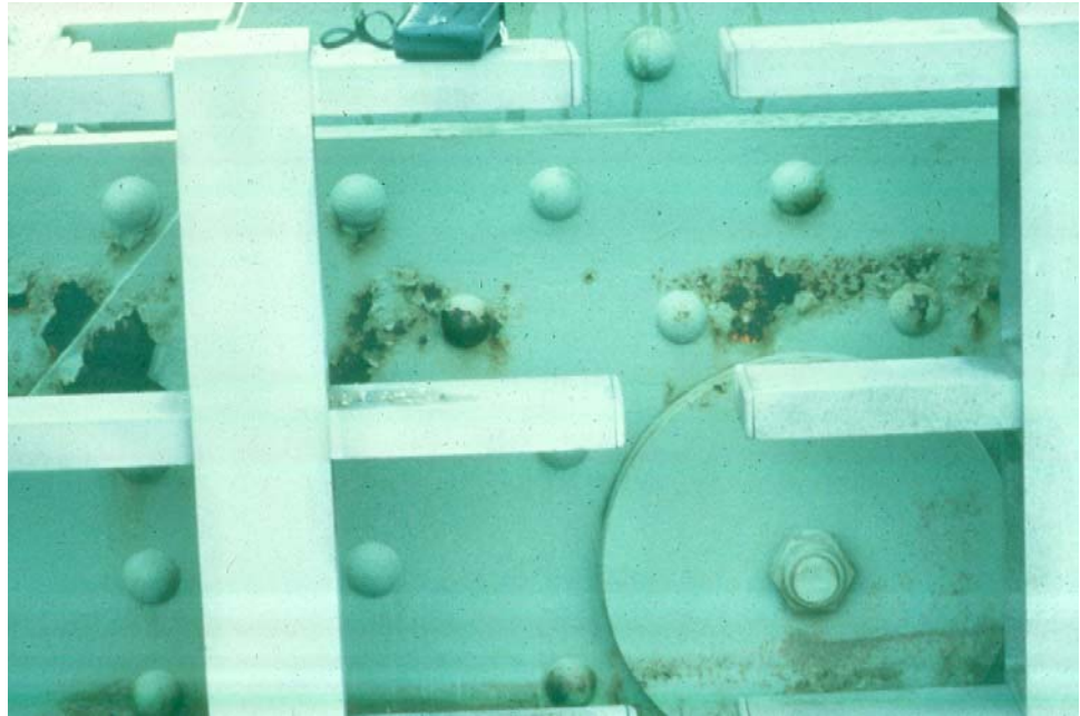
Figure 2.3.21 Roadway Splash Zone Damage (Note Aluminum Bridge Railing in Foreground)
