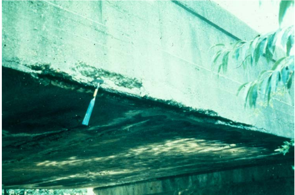
Figure 7.3.8 Exposed Reinforcement in a Through Girder (under hammer)
