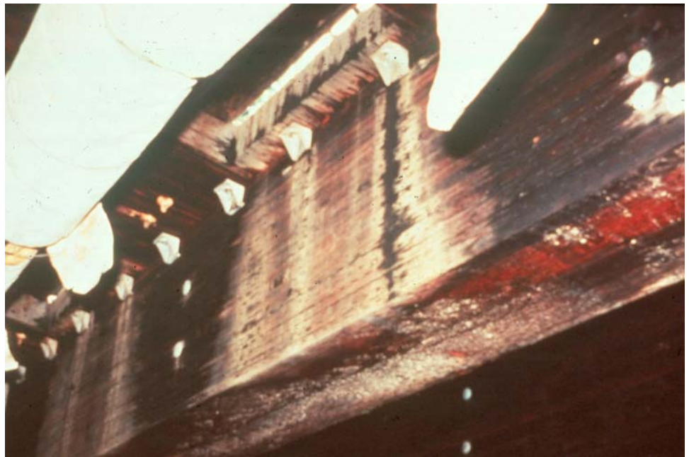
Figure 6.2.15 Decay on Glulam Beam
