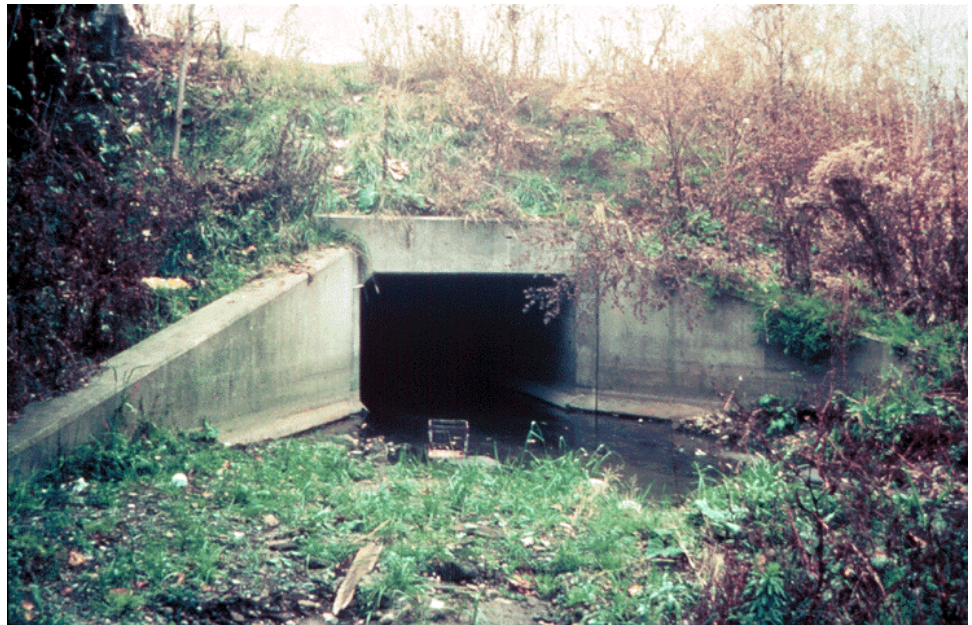
Figure P.3.30 Potential for Tilted Wingwalls
