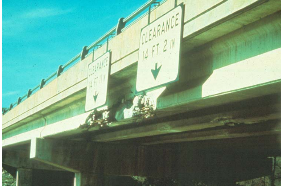
Figure 2.2.24 Collision Damage to Prestressed Concrete I-Beam
