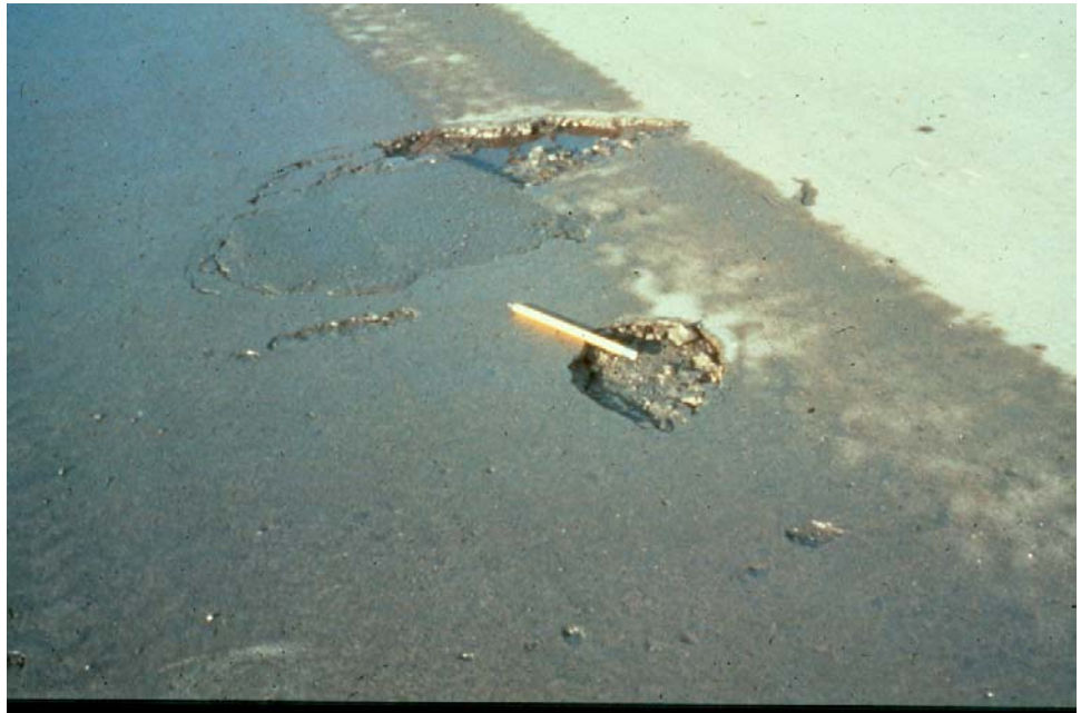
Figure 2.2.20 Spalling on a Concrete Deck
