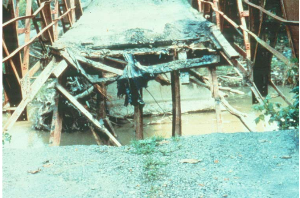
Figure P.1.20 Damaged Bridge due to Failure to Comply with Bridge Posting
