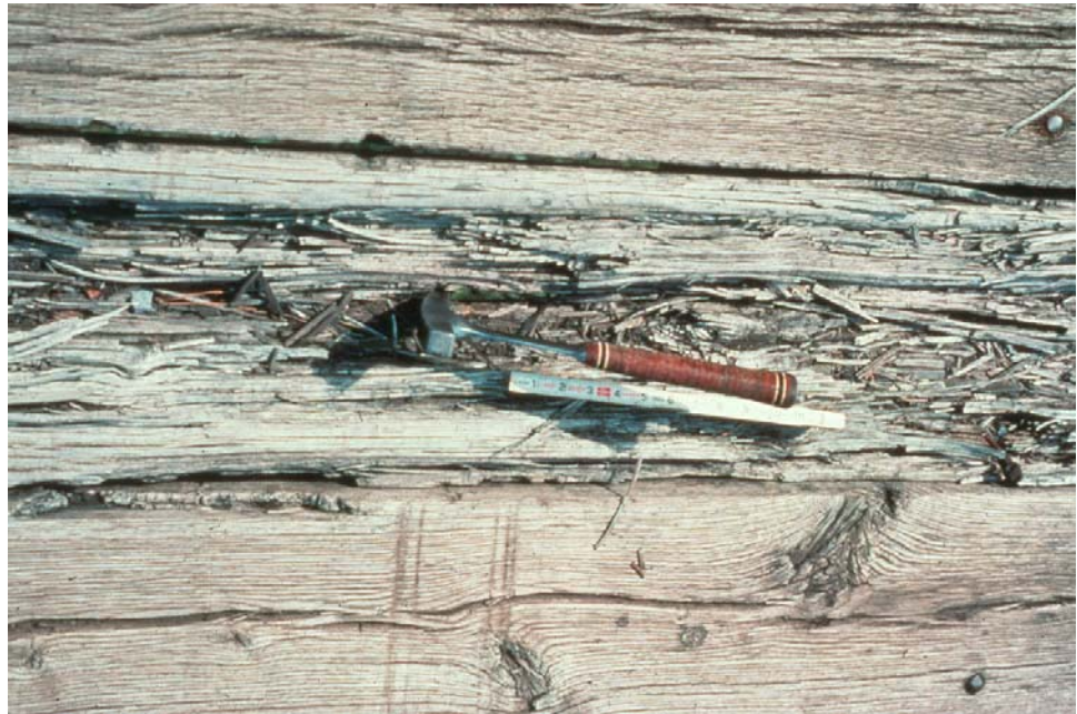
Figure 2.1.23 Weathering on Timber Deck
