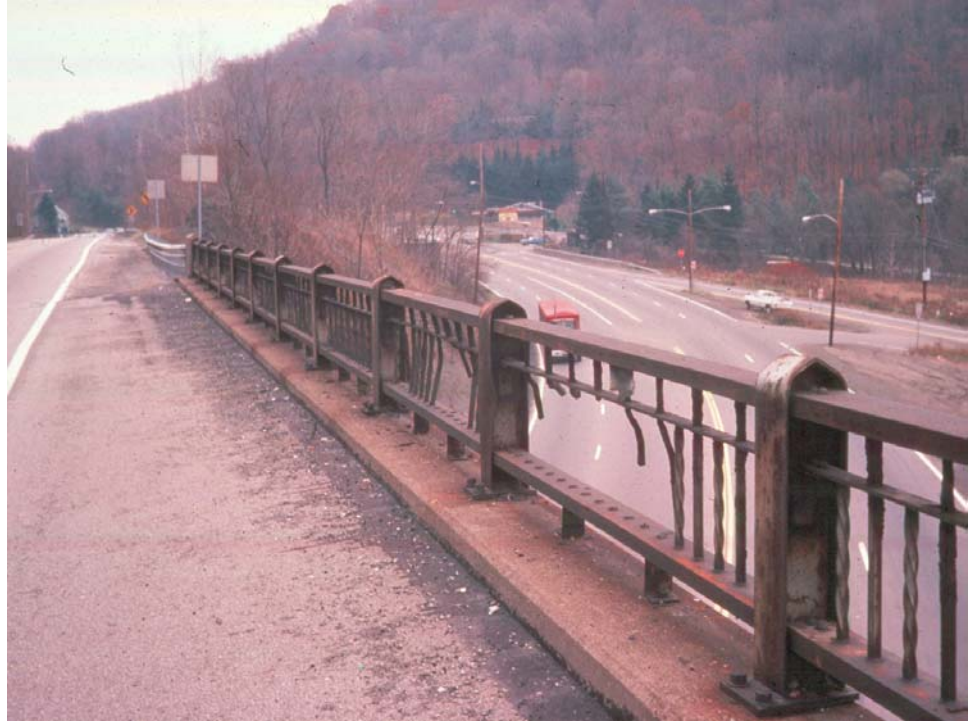
Figure 5.5.18 Damaged Steel Post Bridge Railing
