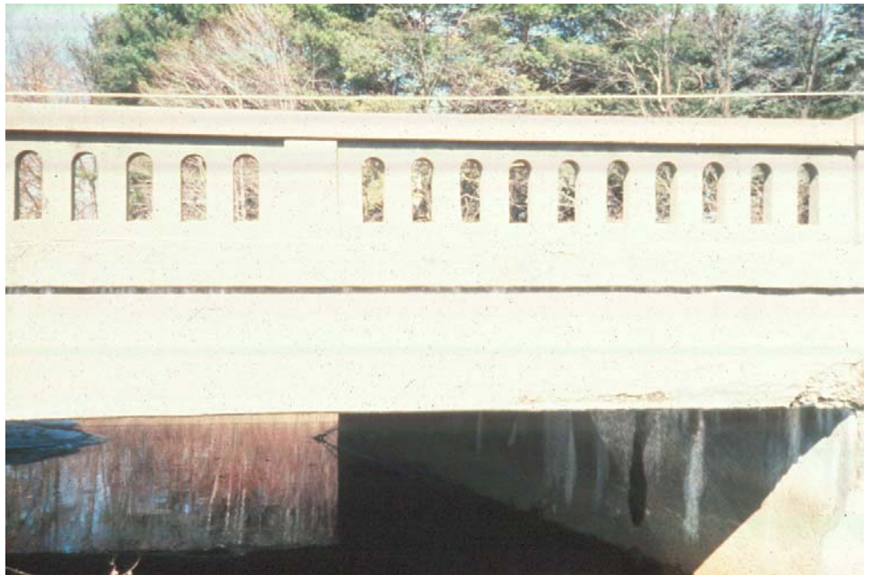
Figure 7.2.19 Deteriorated Tee Beam End Due to Drainage
