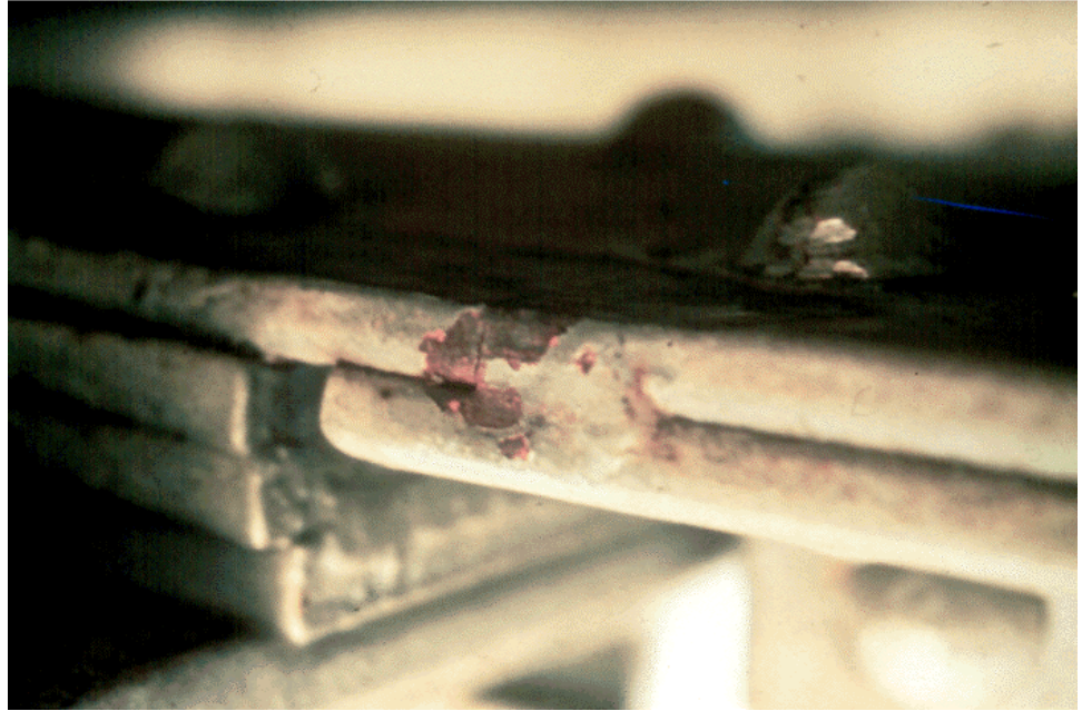
Figure P.2.22 Close-up of Tack Weld on a Riveted Built-up Truss Member
