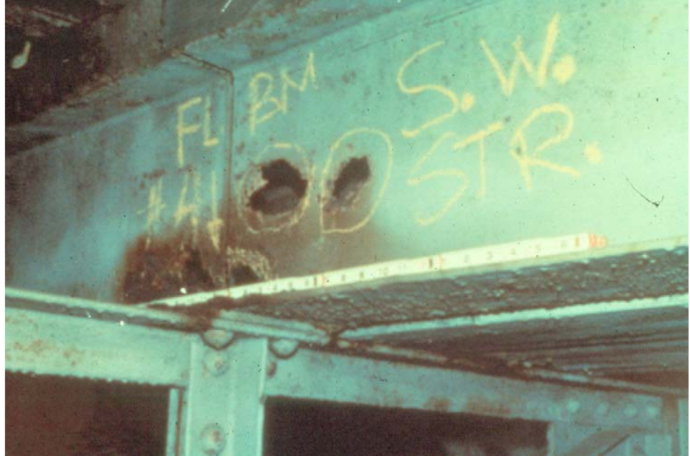
Figure 2.3.6 Steel Corrosion and Complete Section Loss on a Beam Web
