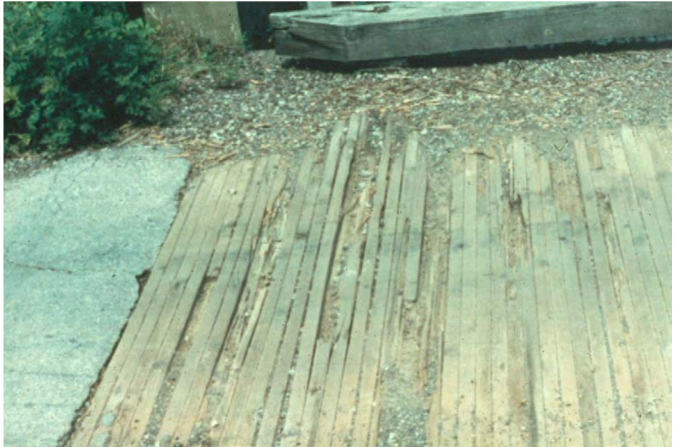
Figure 5.1.8 Wear and Weathering on a Timber Deck
