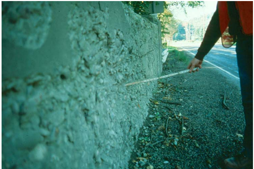
Figure 7.3.9 Close-up of a Girder with Heavy Scaling due to Deicing Agents
