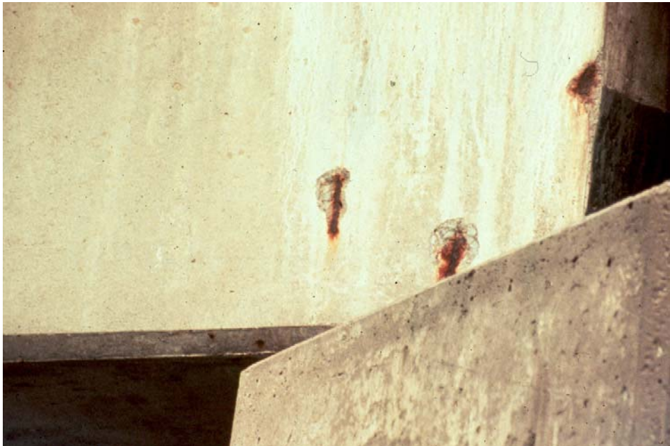
Figure 7.10.12 Exposed Bars at End of Box Beam
