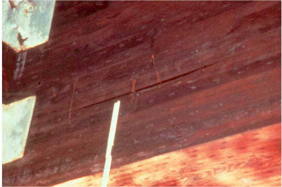
Figure 2.1.16 Delamination in a Laminated Timber Member
