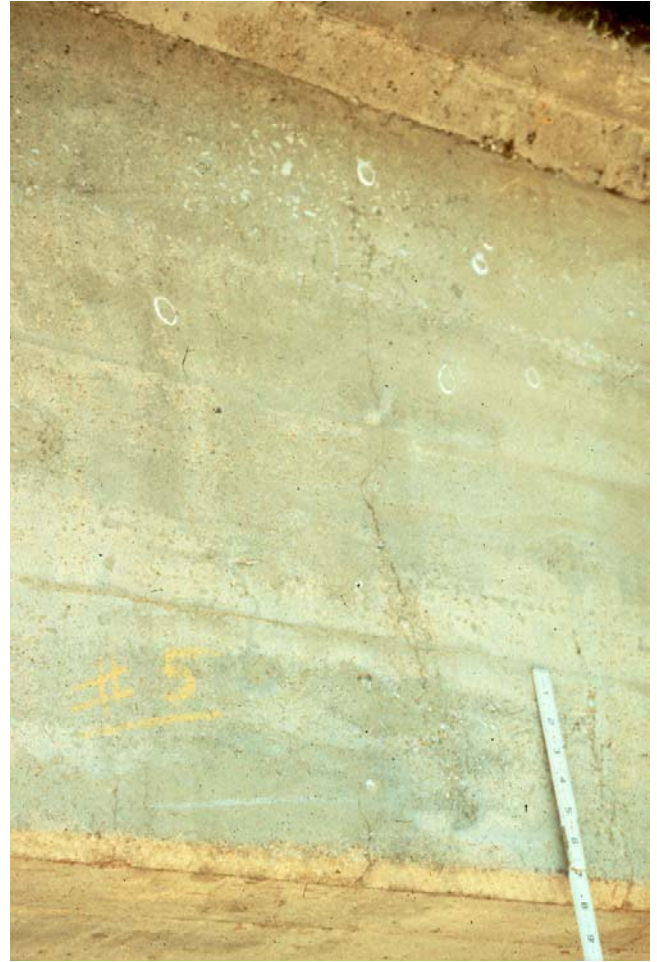
Figure 2.2.7 Flexural Crack on a Tee Beam
