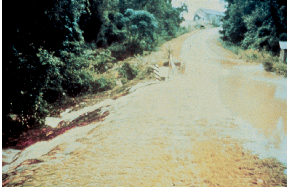
Figure P.3.26 Approach Roadway at a Culvert Site
