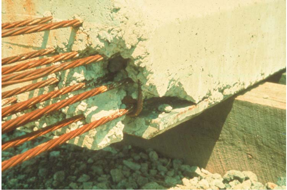
Figure 7.9.9 Spalling Due to Poor Concrete
