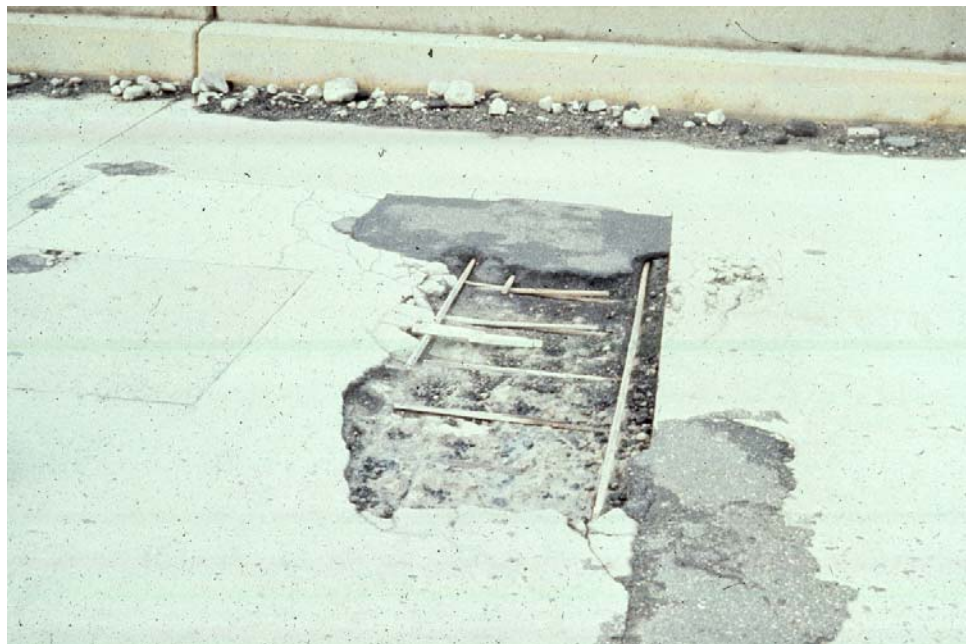
Figure 5.2.5 Pothole Showing Deck Reinforcing Steel Perpendicular to Traffic
