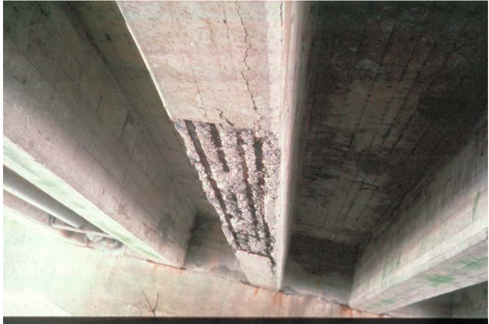
Figure 7.2.16 Spall on the Bottom of the Stem of a Cast-in-Place Tee Beam with Corroded Main Steel Exposed
