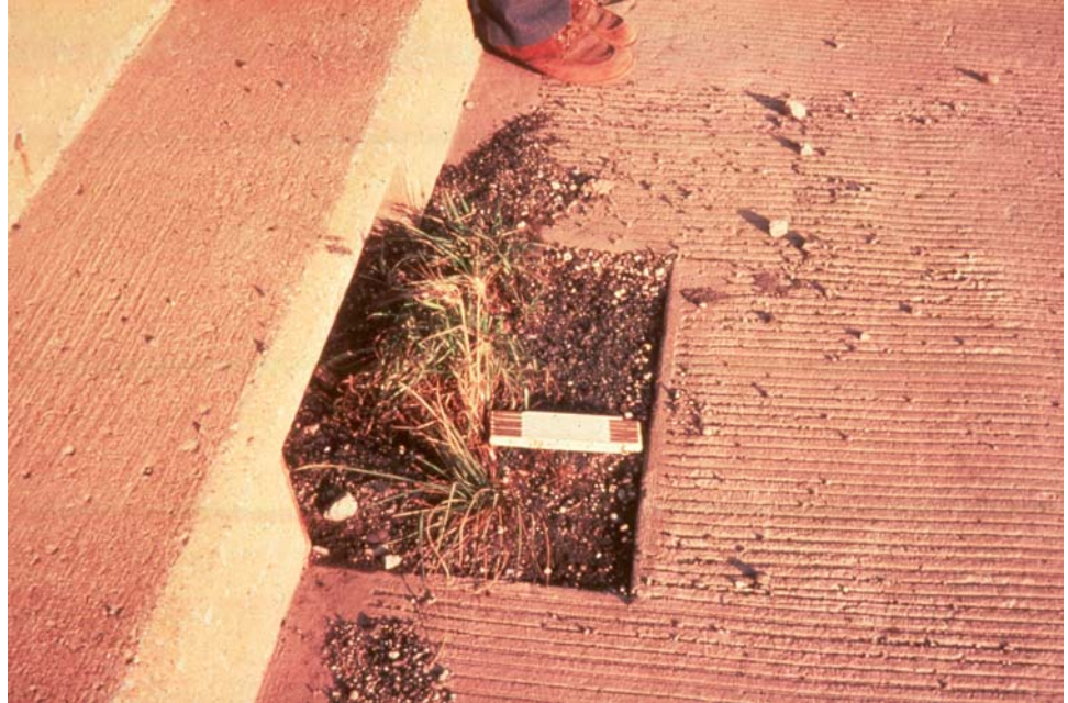
Figure 5.4.21 Clogged Drainage Inlet
