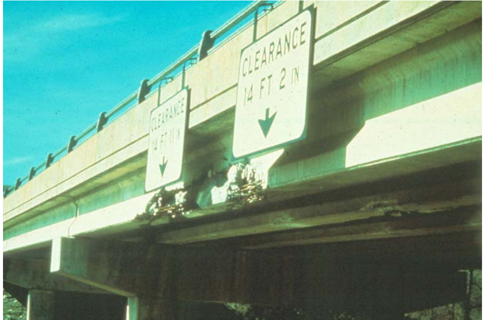
Figure 7.9.13 Collision Damage on Prestressed Concrete I-Beam
