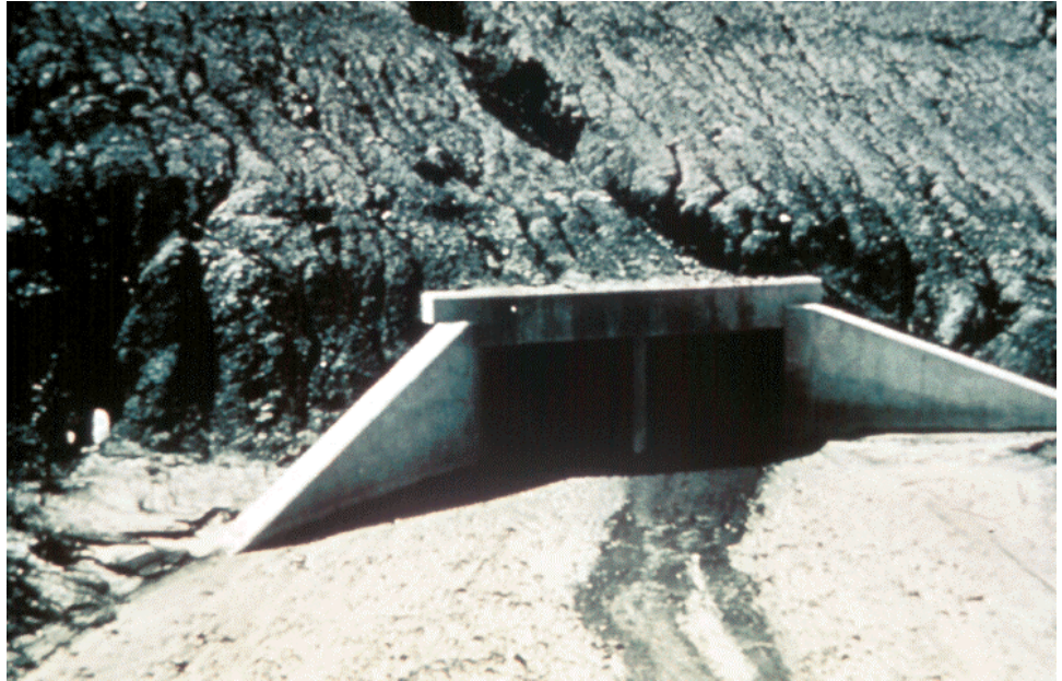
Figure P.3.28 Slide Failure
