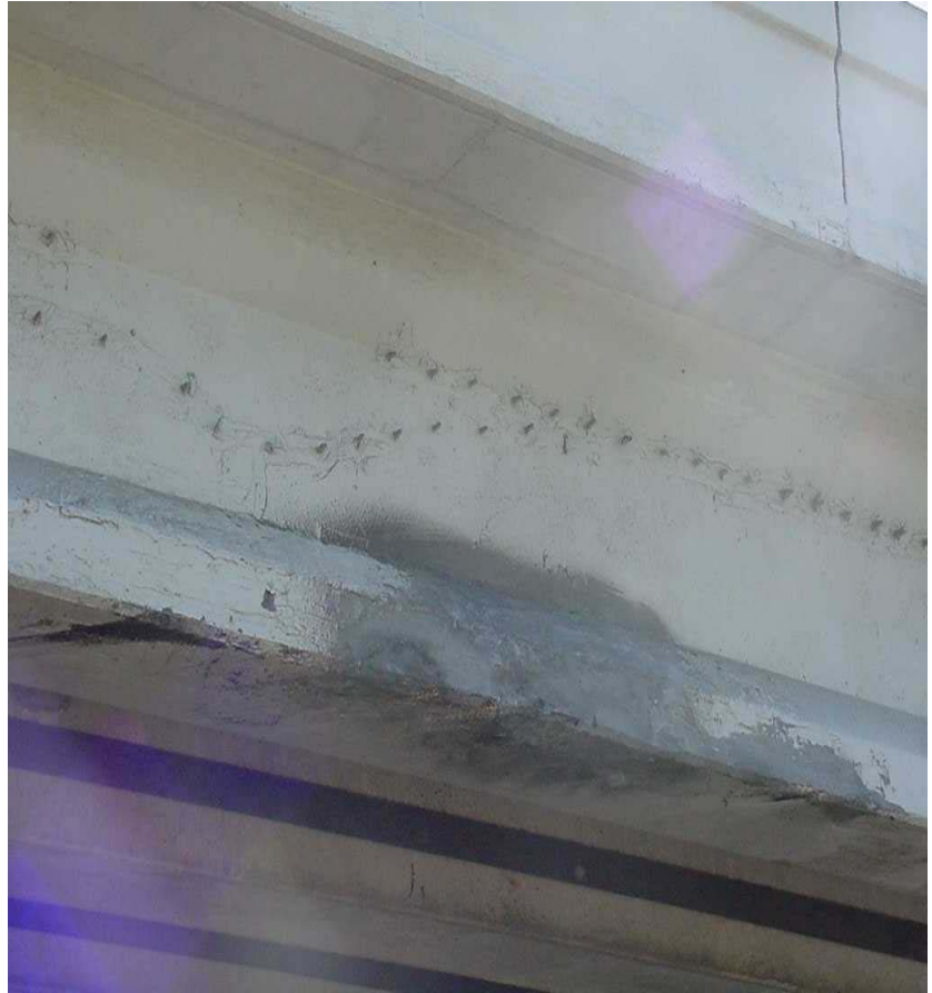
Figure 7.9.14 Collision Damage Repair on Prestressed Concrete I-Beam. Note Epoxy Injection Ports
