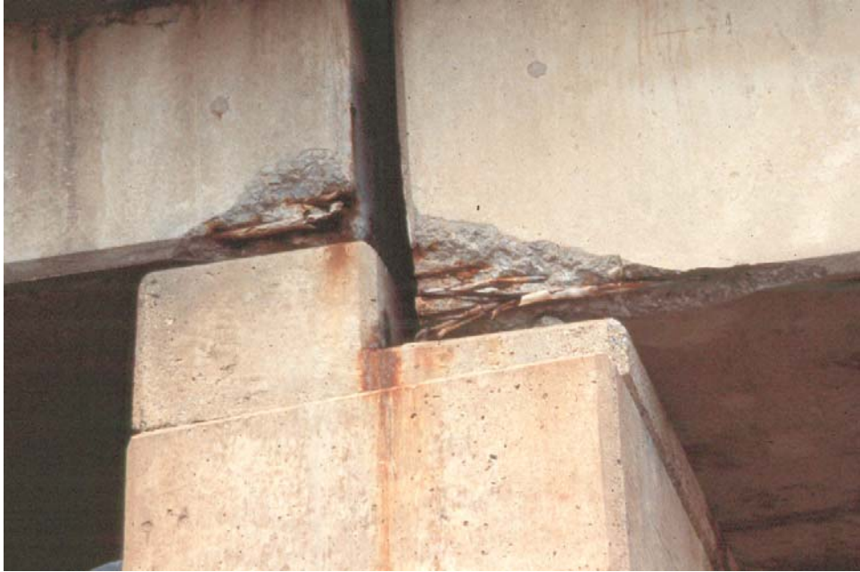
Figure 7.10.11 Spalled Beam Ends
