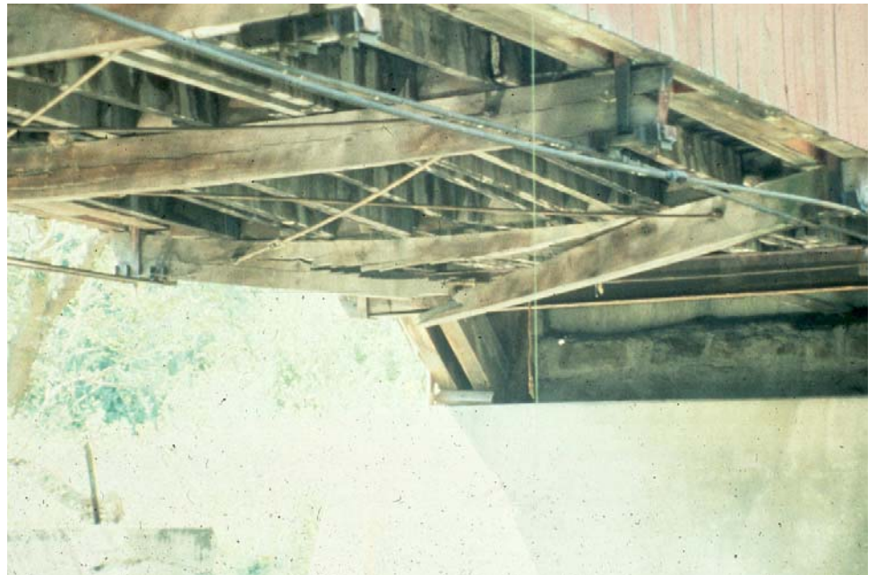
Figure 2.1.22 Failed Timber Floor Beam
