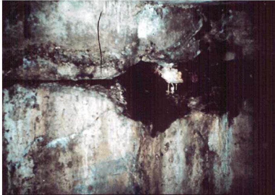
Figure 7.12.10 Spalls and Delaminations
