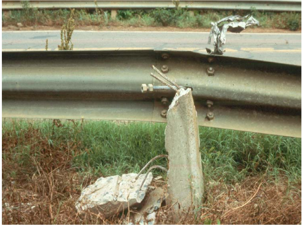
Figure 5.5.19 Approach Guardrail Collision Damage
