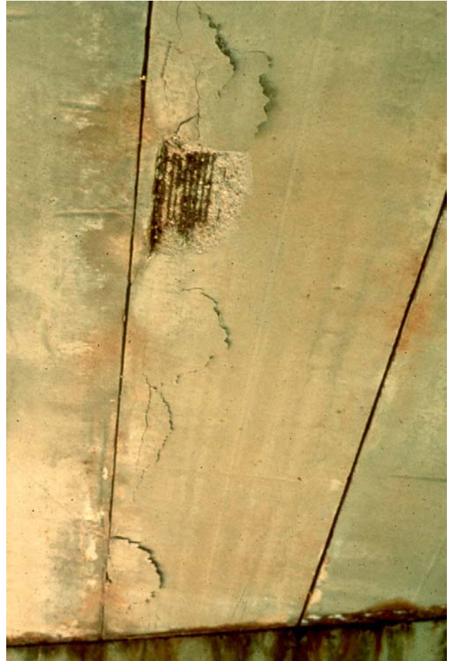
Figure 7.10.14 Spall and Exposed Reinforcement
