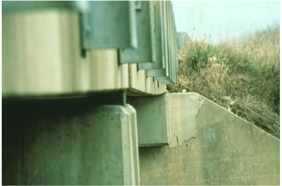
Figure 7.4.6 Excessive Deflection at Midspan
