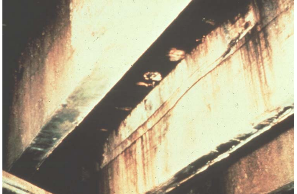
Figure 2.1.21 Horizontal Shear Failure in Timber Member
