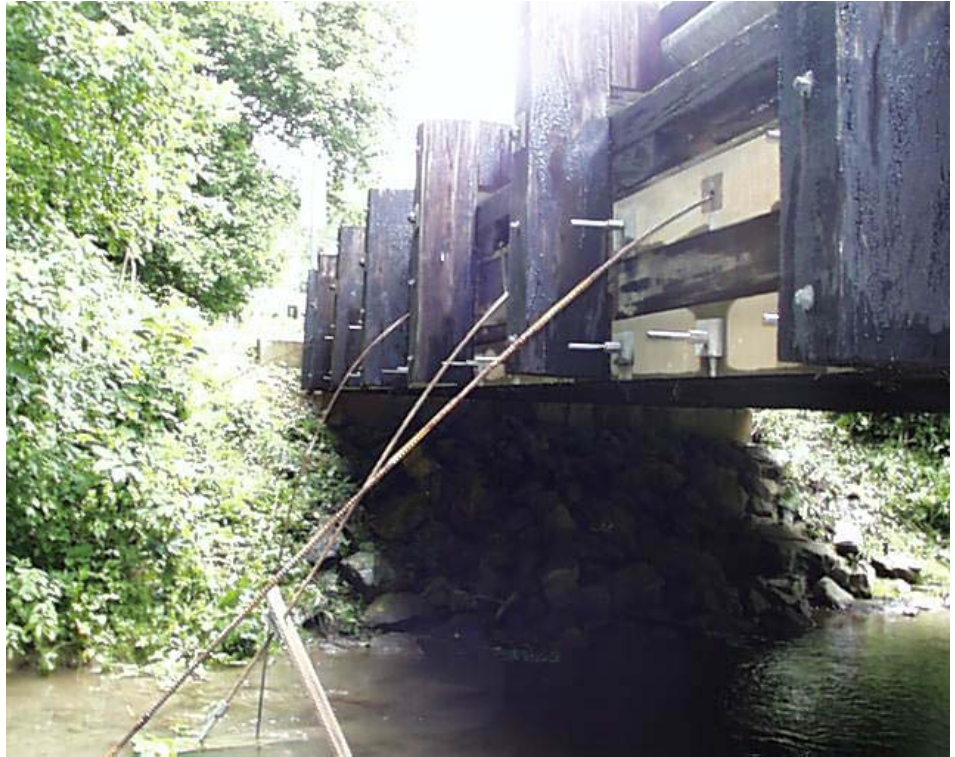
Figure 6.3.10 Broken Stressing Rods
