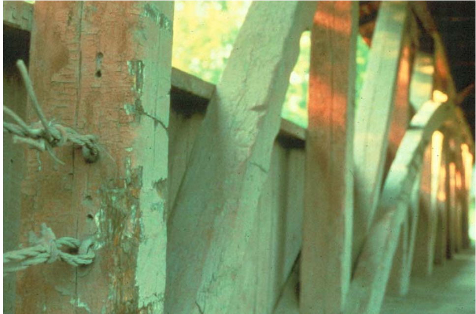
Figure 2.1.19 Impact/Collision Damage to a Timber Member
