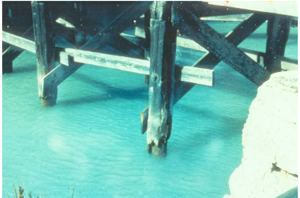
Figure 2.1.13 Marine Borer Damage to Wood Piling
