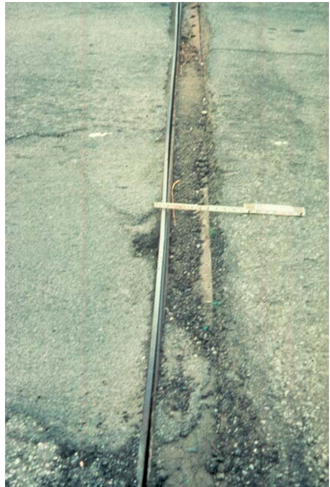
Figure 5.4.15 Debris Lodged in a Sliding Plate Joint
