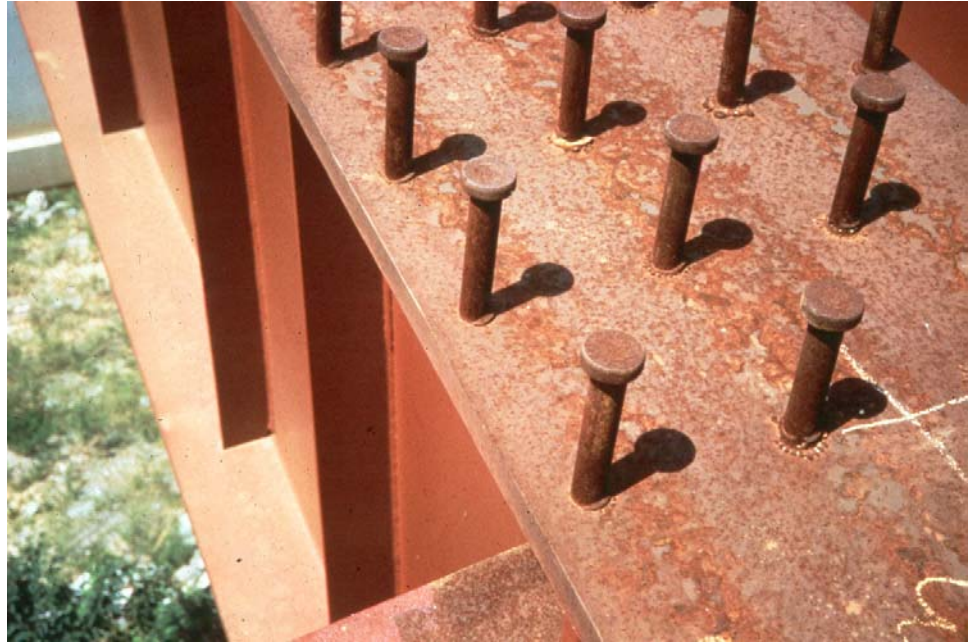
Figure P.2.28 Shear Studs on Top Flange of Girder before Concrete Deck is Poured
