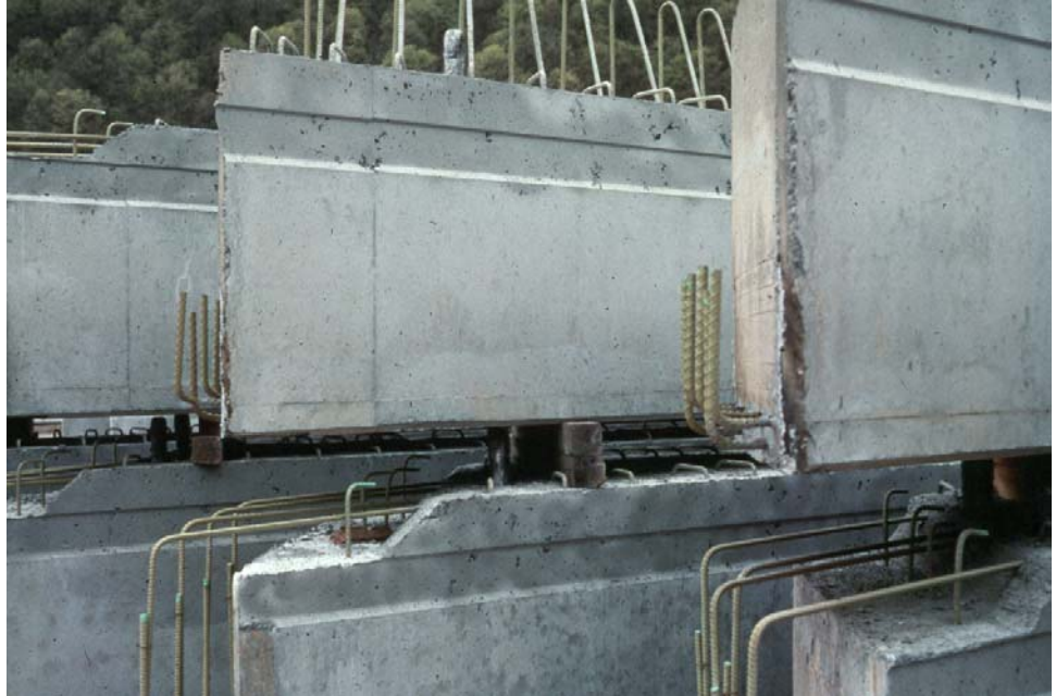
Figure 7.10.3 Box Beams at Fabrication Plant Showing Shear Connectors and Extended Rebar for Continuity
