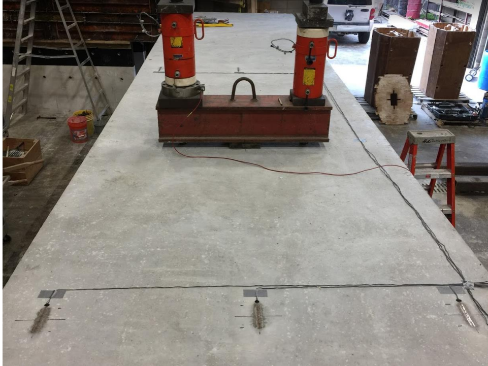
a) Strain gauge arrangement on concrete deck
