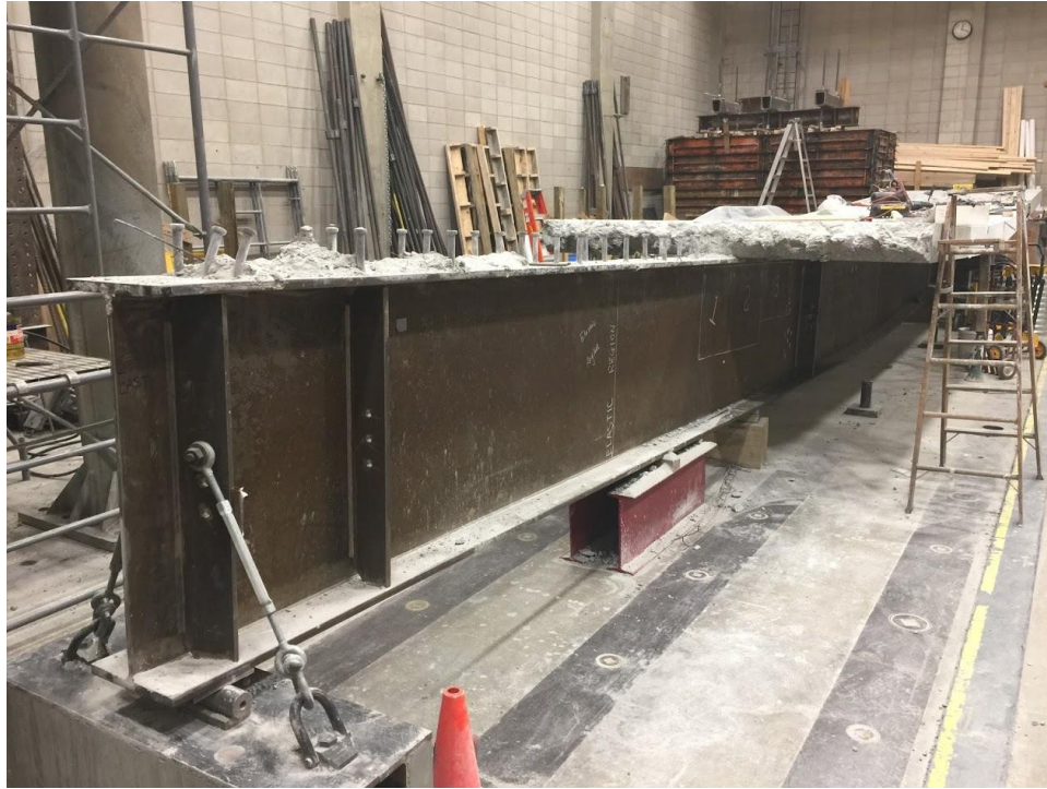
a) Beam after concrete deck removed
