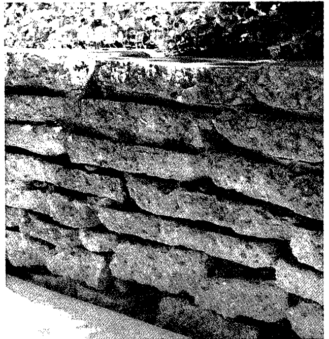
Broken concrete used as a retaining wall
