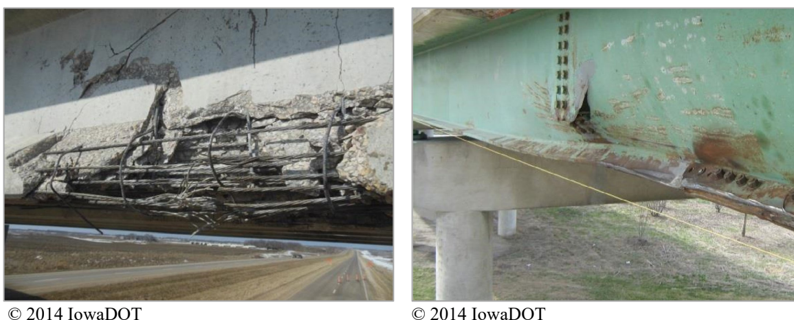
Figure 1. Photos. Examples of Truck Impact Damage.
