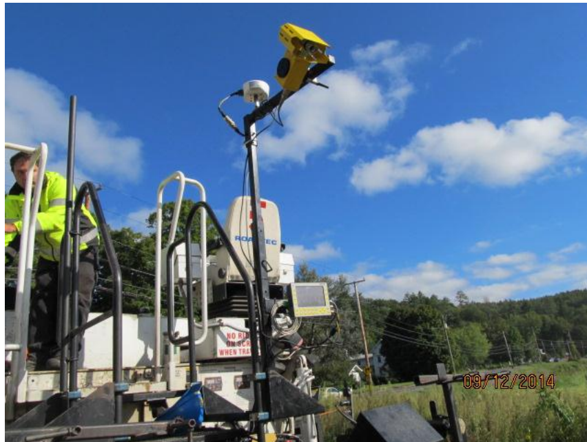
Figure 6. Photo. Infrared thermal scanner attached to rear of paver with interface controller mounted below. (courtesy: Vermont Agency of Transportation)
