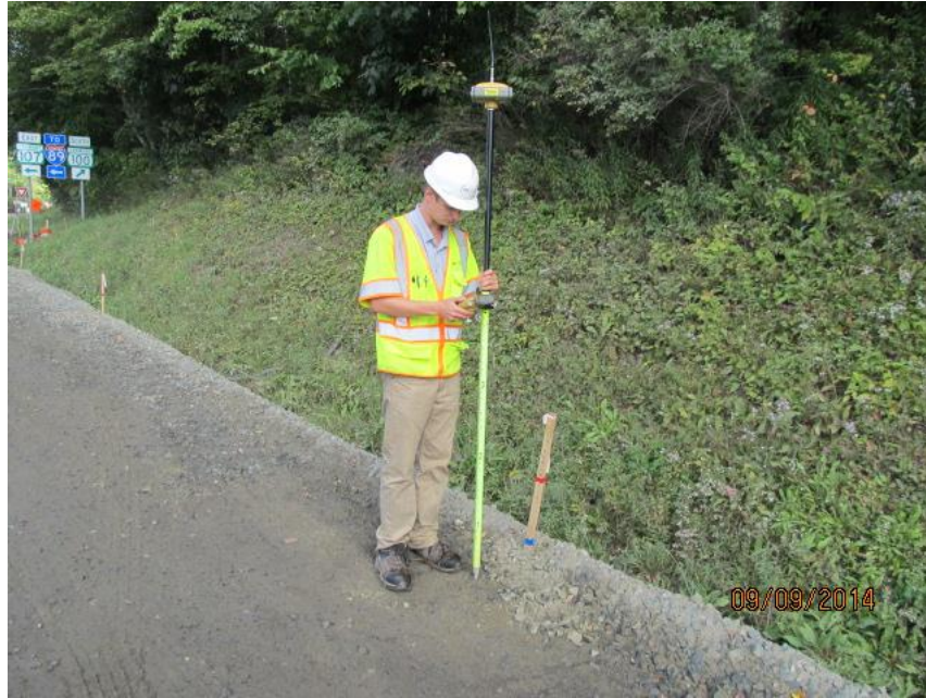
Figure 10. Photo. GPS rover and data collector used to check cut/fill levels for subbase. (courtesy: Vermont Agency of Transportation)
