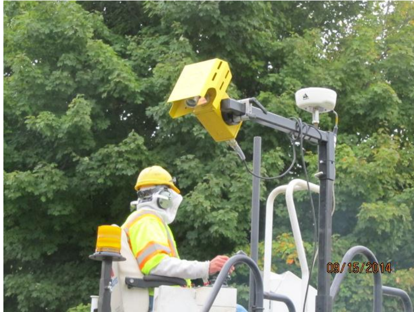
Figure 7. Photo. Infrared thermal scanner attached to rear of paver with GPS receiver behind it. (courtesy: Vermont Agency of Transportation)
