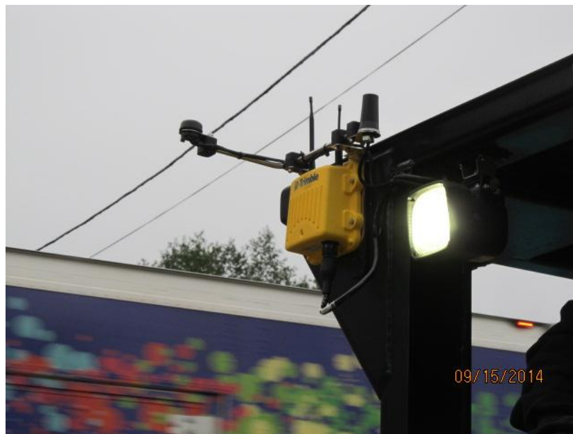
Figure 5. Photo. IC GPS and radio receiver mounted to paving roller Cat CB54 XW. (courtesy: Vermont Agency of Transportation)
