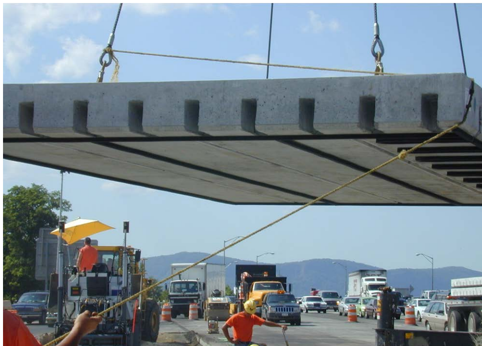
Figure 20. Inverted dovetail slots and foam gaskets underneath slab to control flow (image from project in New York State, 2002).
