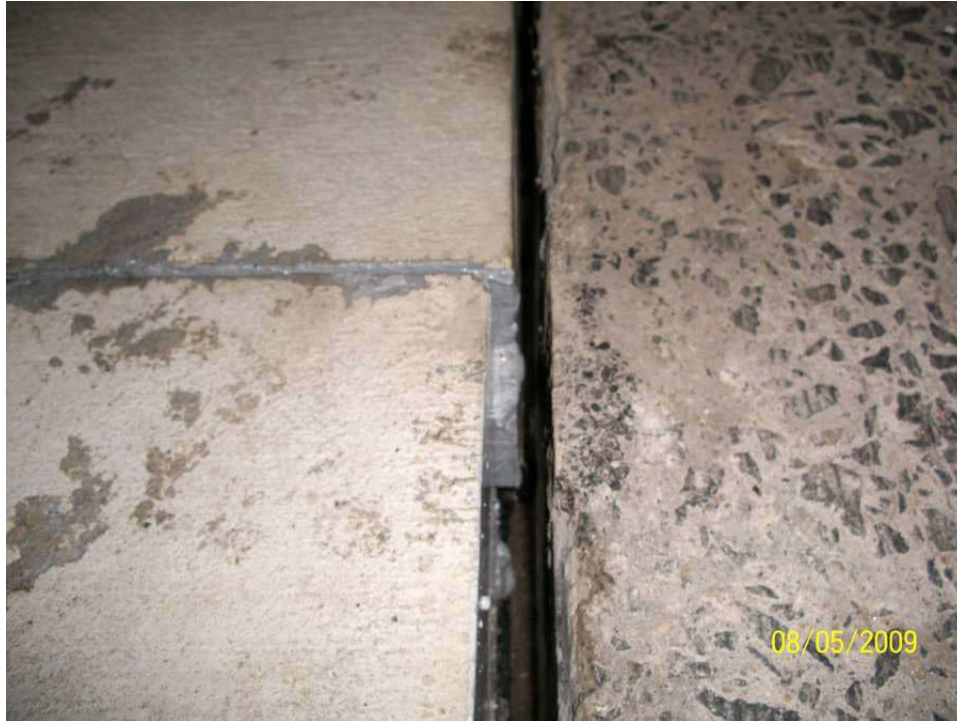
Figure 50. Transverse joint misalignment.
