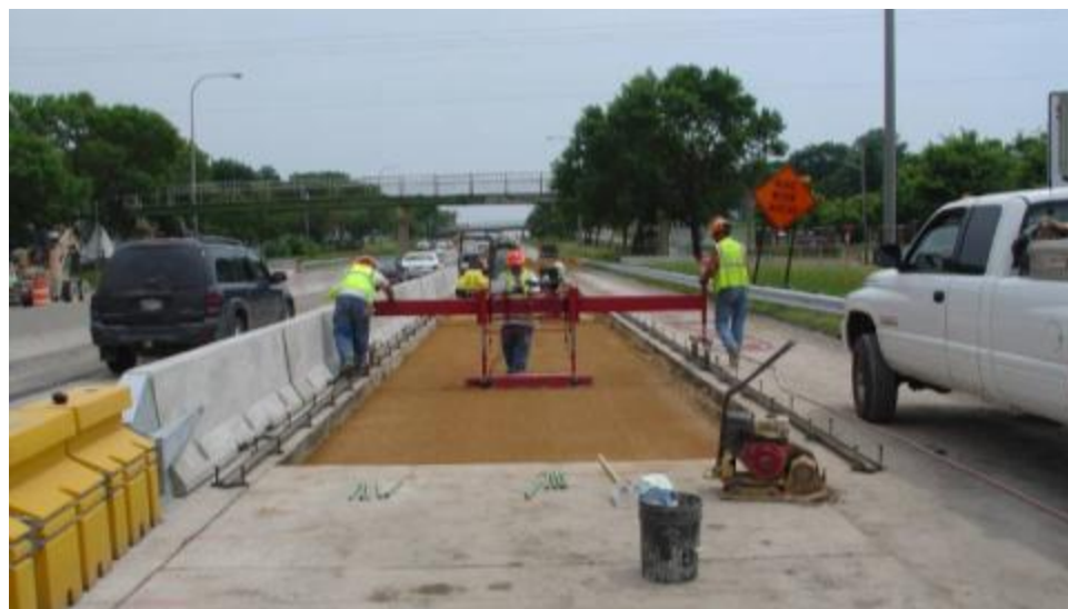
Figure 18. Hand-operated grader supported on rails (image from project in New York State, 2002).
