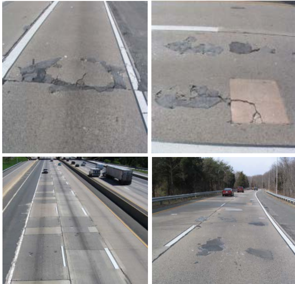
Figure 6. Surface condition of I-66 mainline and ramp leading to US 50 West in 2008.
