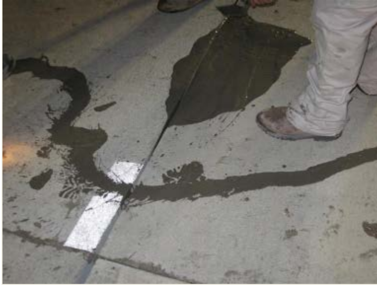
Figure 48. Grout leak from post-tensioning ducts.
