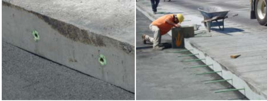
Figure 19. Mechanical connectors for tie bars and installed tie bars (image from project in New York State, 2002).
