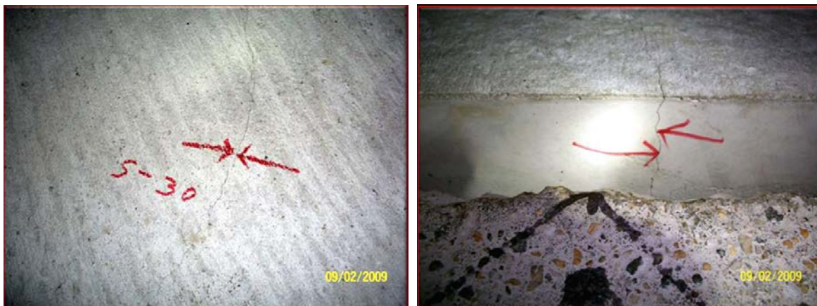
Figure 59. Slab cracking observed in the jointed PCPS panels on the ramp.
