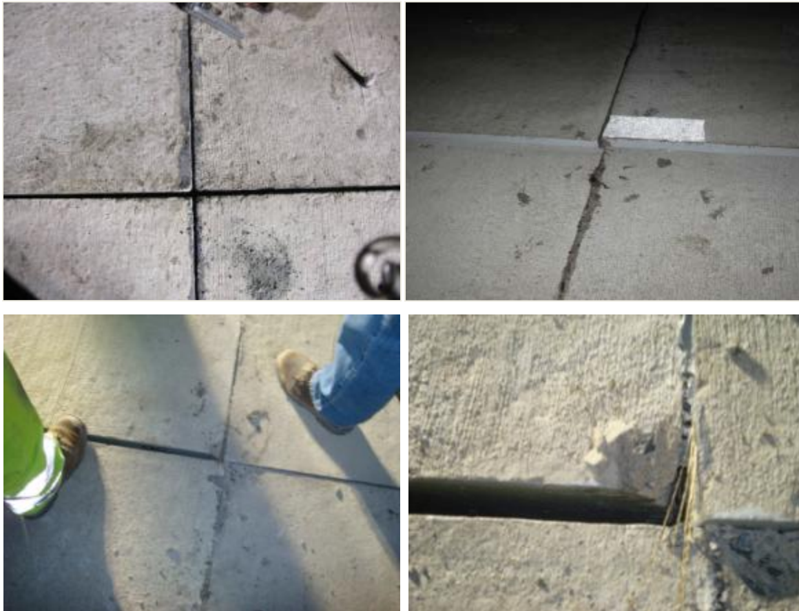
Figure 49. Issues with vertical and horizontal alignment of slabs and large joint openings.
