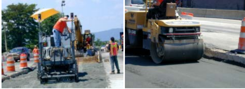
Figure 17. Use of specialized grading devices and base finish achieved (image from project in New York State, 2002).
