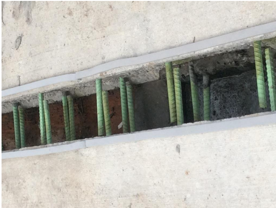
Figure 11. Photo. Transverse Deck Joint. (courtesy: UDOT)
