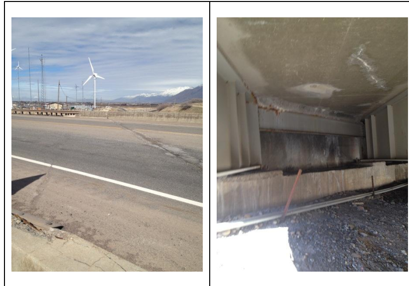
Figure 2. Photos. C-679 bridge condition prior to reconstruction. (courtesy: UDOT)
