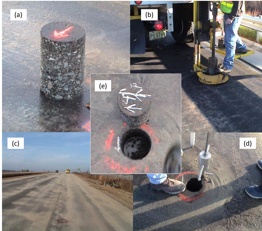
Figure B-1 Representative photos from the field: (a) core from Project R-2241A in Roxboro, (b) coring in Roxboro, (c) identified section and marked spots for coring for Project X-002CC in Fayetteville, (d) DCP measurements, and (e) core and core hole from Project X-002CC, I-295.
