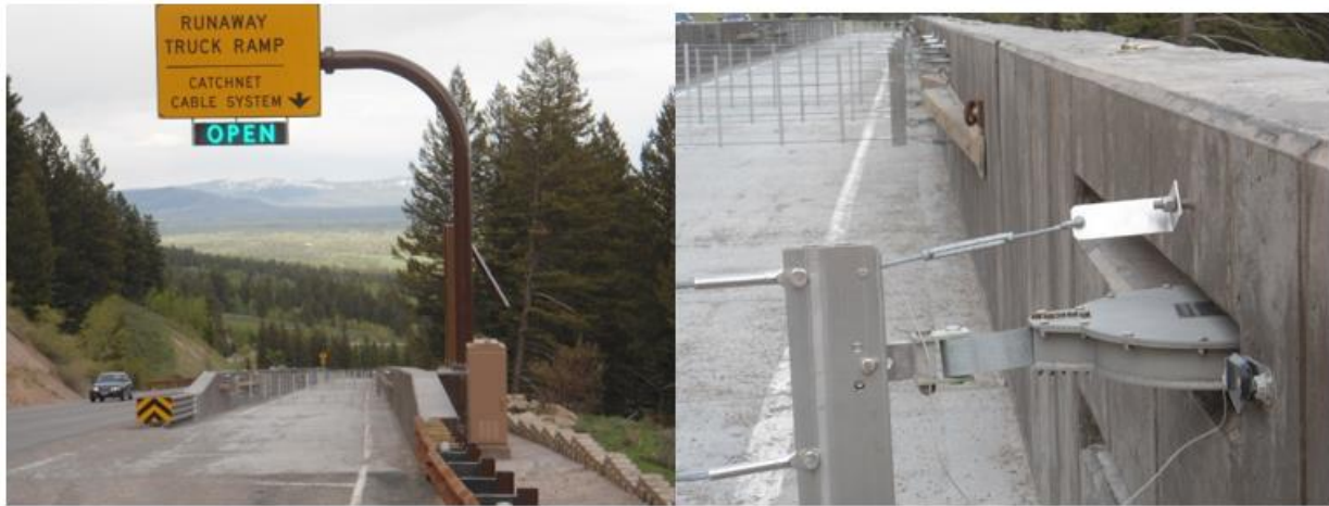
(A) Cable Catch-Net System at Teton Pass (WY-22).
