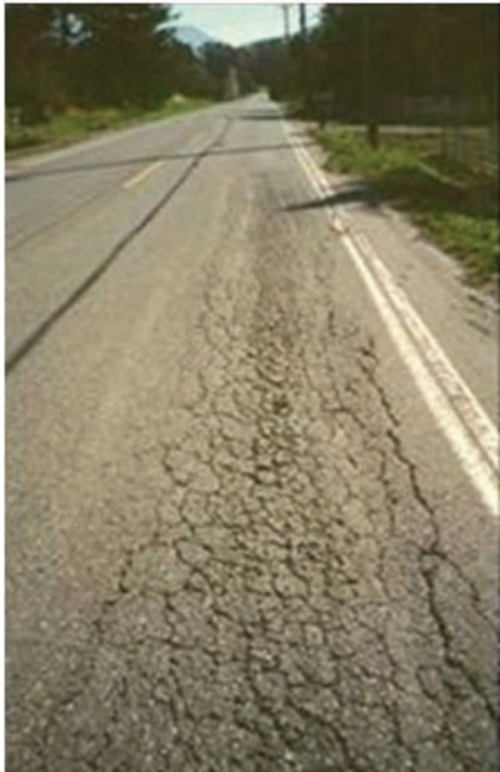
Figure 1.1 Advanced fatigue cracking (photo courtesy of G. Huber).
