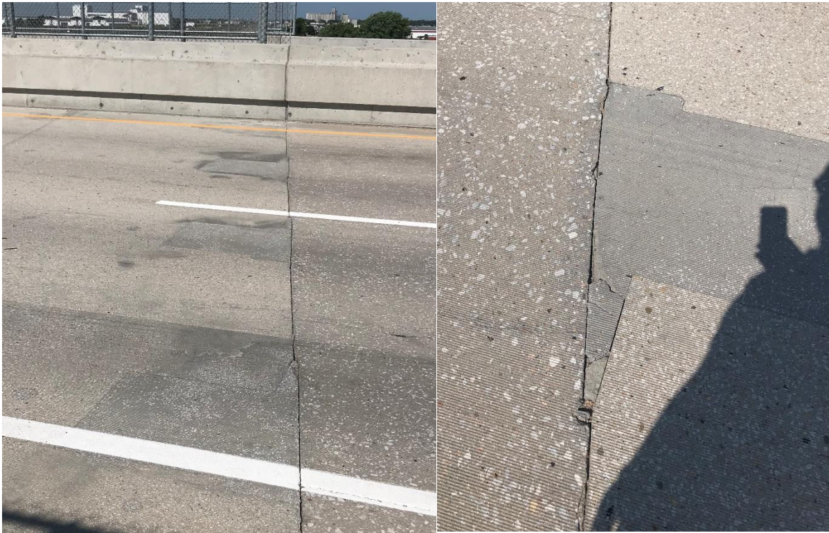
FIGURE 2.28 North (left) and south (right) PT anchorage blocks of the precast deck
