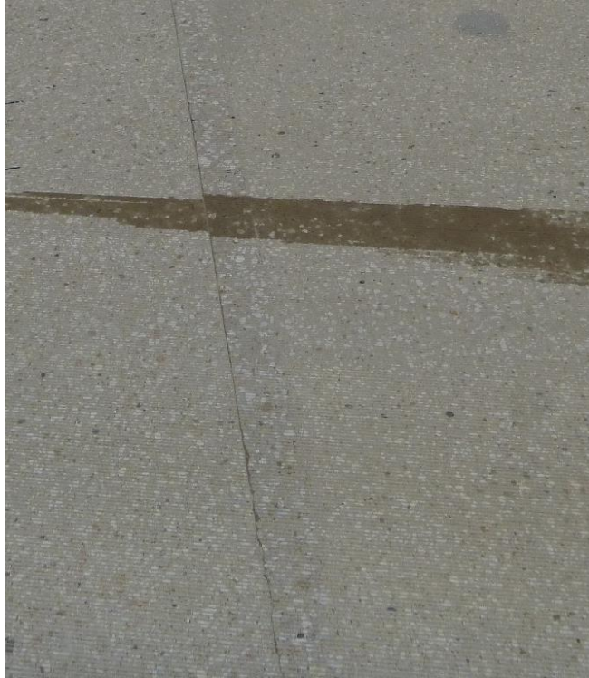
FIGURE 2.7 Transverse joint with pour line between cast-in-place and precast concrete at the intermediate pier
