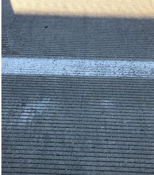
FIGURE 2.21 One of the transverse cracks extending the full width of CIP deck
