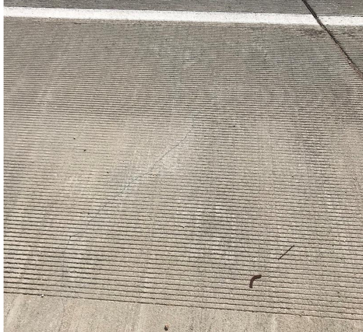
FIGURE 2.26 One of the transverse cracks extending the full width of CIP deck
