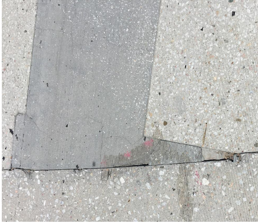
FIGURE 2.18 Random cracking at one of the south anchorage blocks
