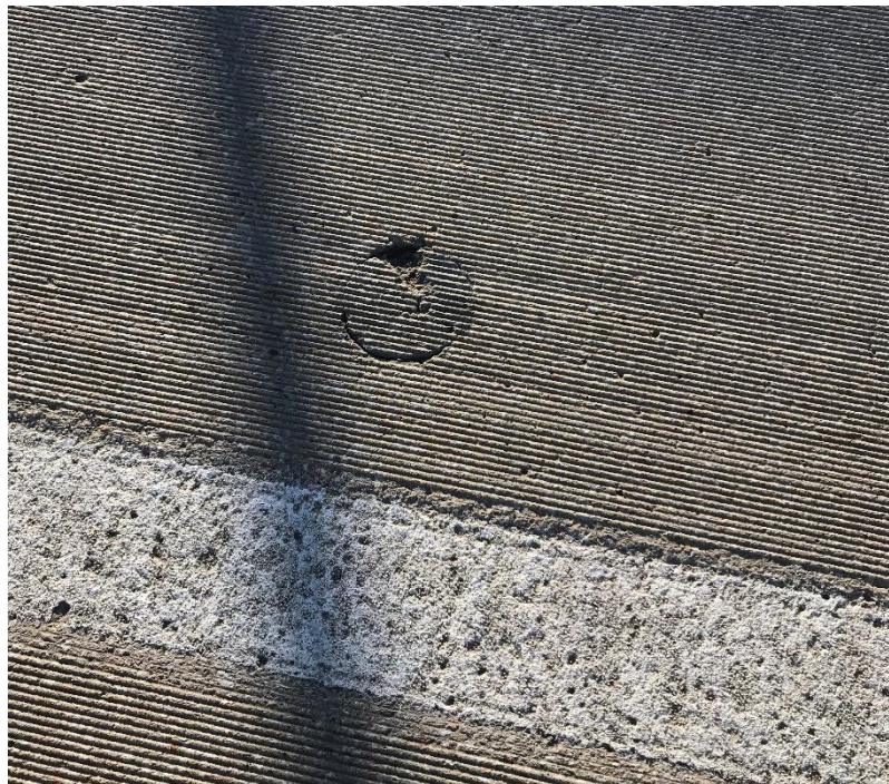
FIGURE 2.24 One of the grouting holes with signs of distress
