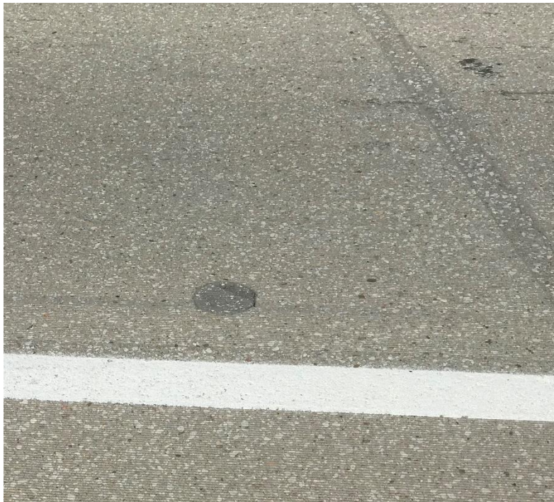
FIGURE 2.29 One of the grouting holes with cracking
