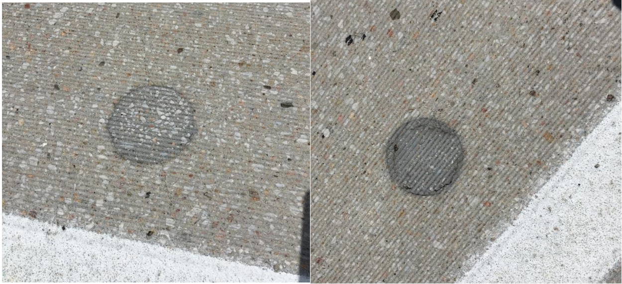
FIGURE 2.16 Fine cracks inside some of the grouting holes of the precast concrete deck
