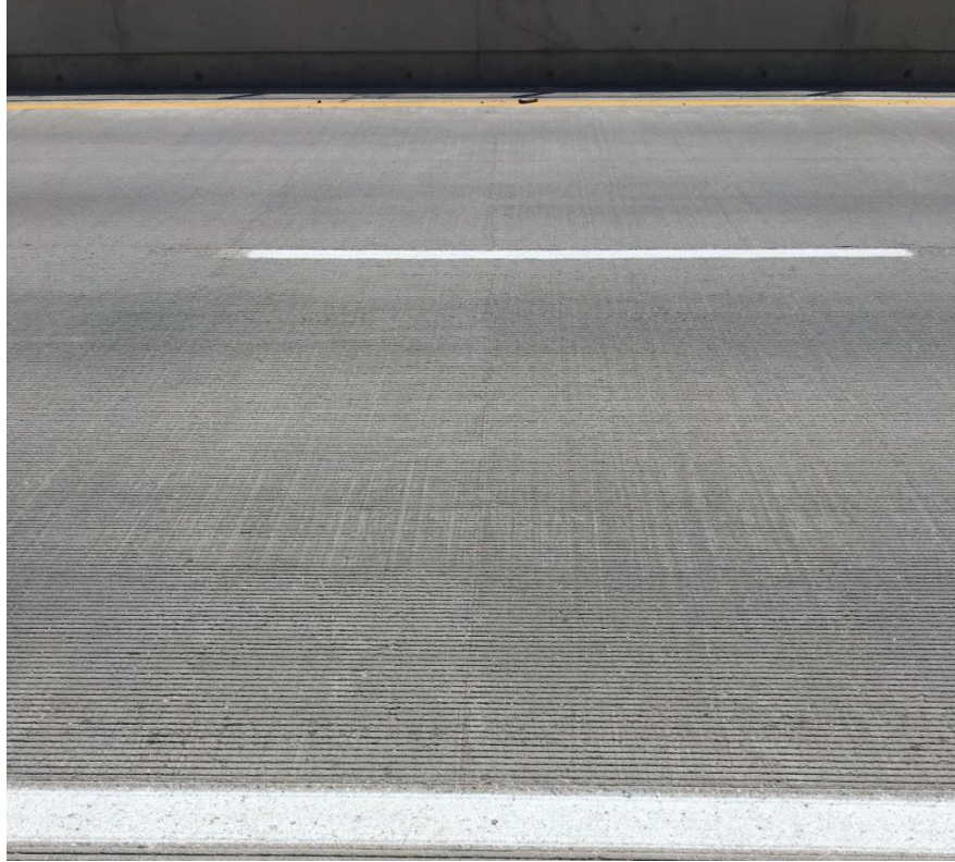
FIGURE 2.12 Transverse cracks in the cast-in-place concrete deck at mid-span section
