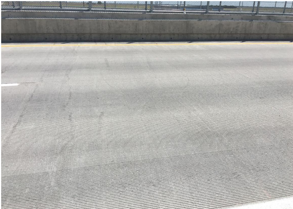
FIGURE 2.13 Transverse cracks in the cast-in-place concrete deck at the intermediate pier
