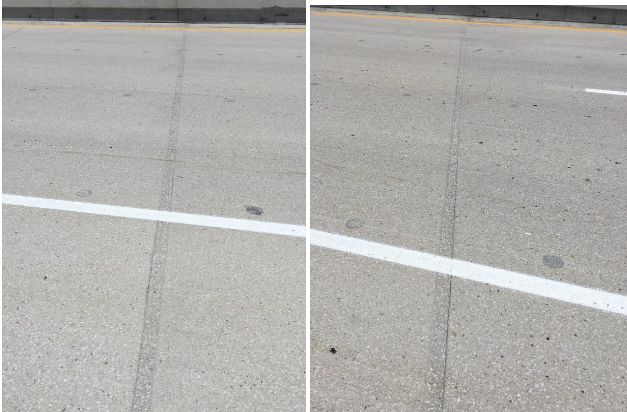
FIGURE 2.14 Transverse joints between precast concrete deck panels at the intermediate pier section (left) and mid-span section (right)
