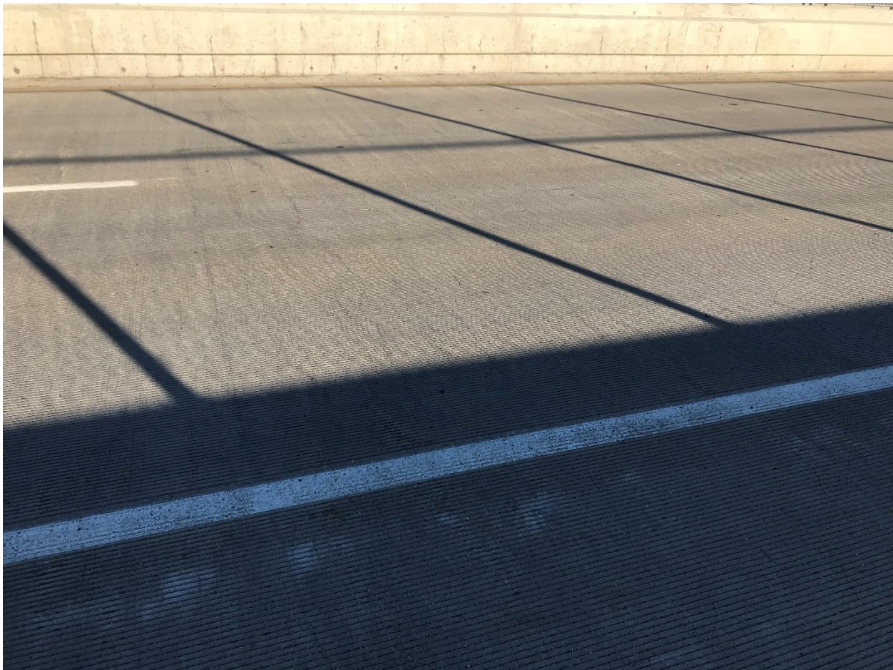
FIGURE 2.20 Multiple transverse cracks at the negative moment region of CIP deck
