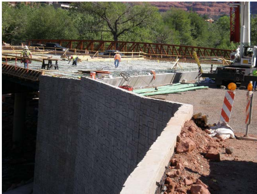
Figure 24. Construction of the first phase of the new Oak Creek Bridge (prefabricated pedestrian bridge already constructed in the background).
