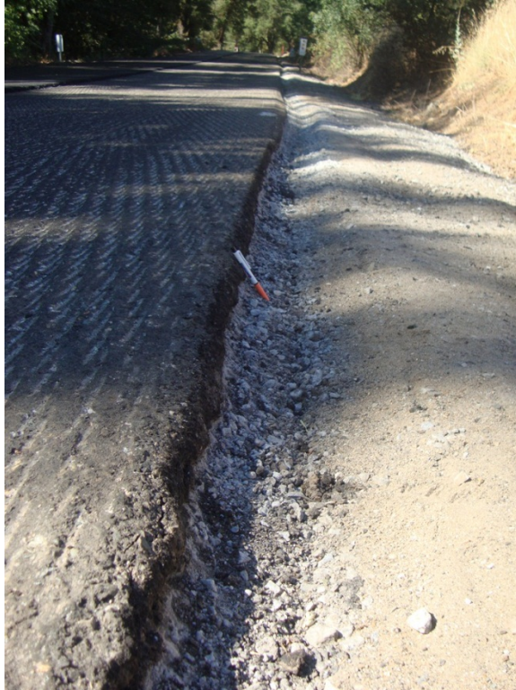
Figure 40. In many locations the shoulder material was clipped below the level of the existing pavement surface, resulting in Safety Edge heights greater than the overlay thickness.
