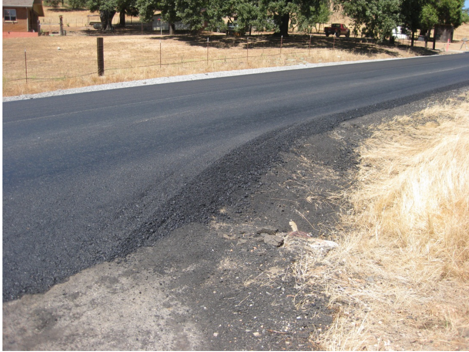
Figure 31. The Safety Edge shoe was lowered to the original position at the end of driveways and cross streets.
