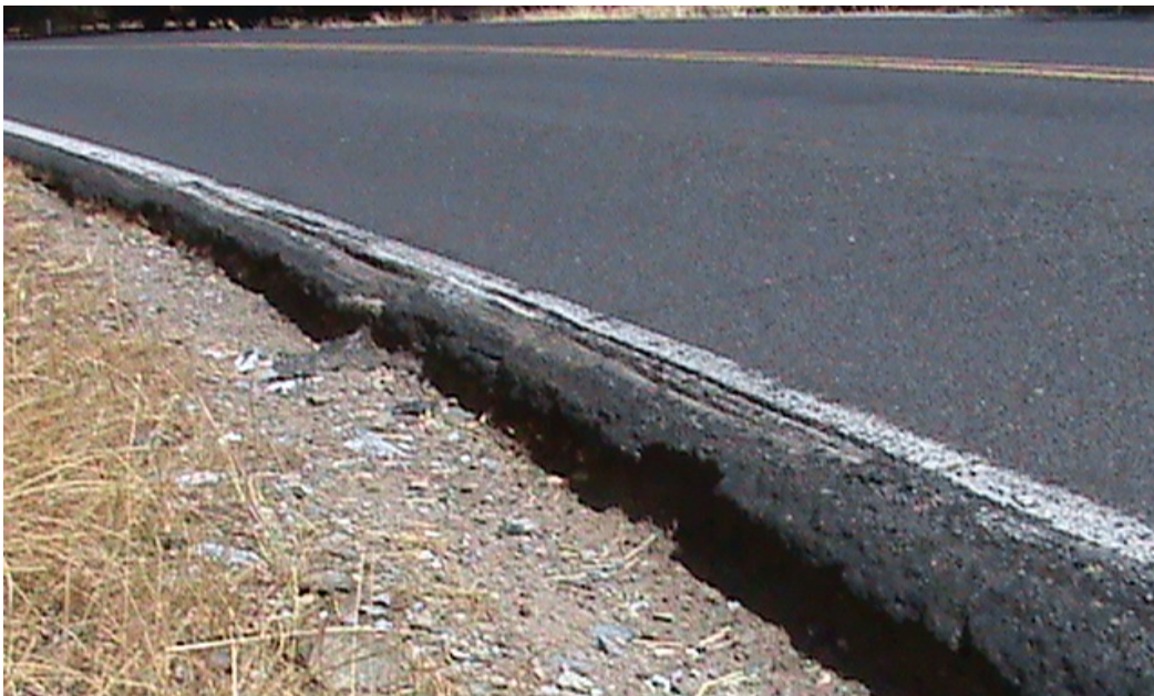
Figure 3. Typical car shackle bolt damage to Mountain Ranch Road edge on inside of turn.
