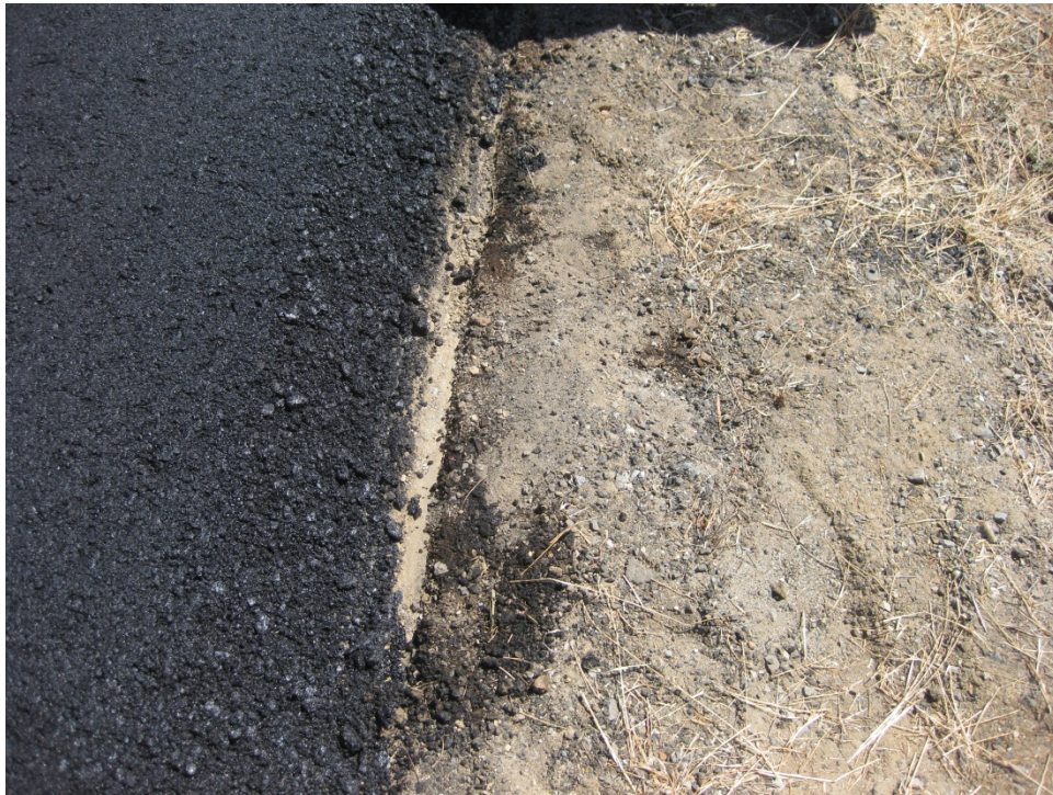
Figure 28. In a few locations, the Safety Edge shoe was too low and it pushed into the shoulder material.
