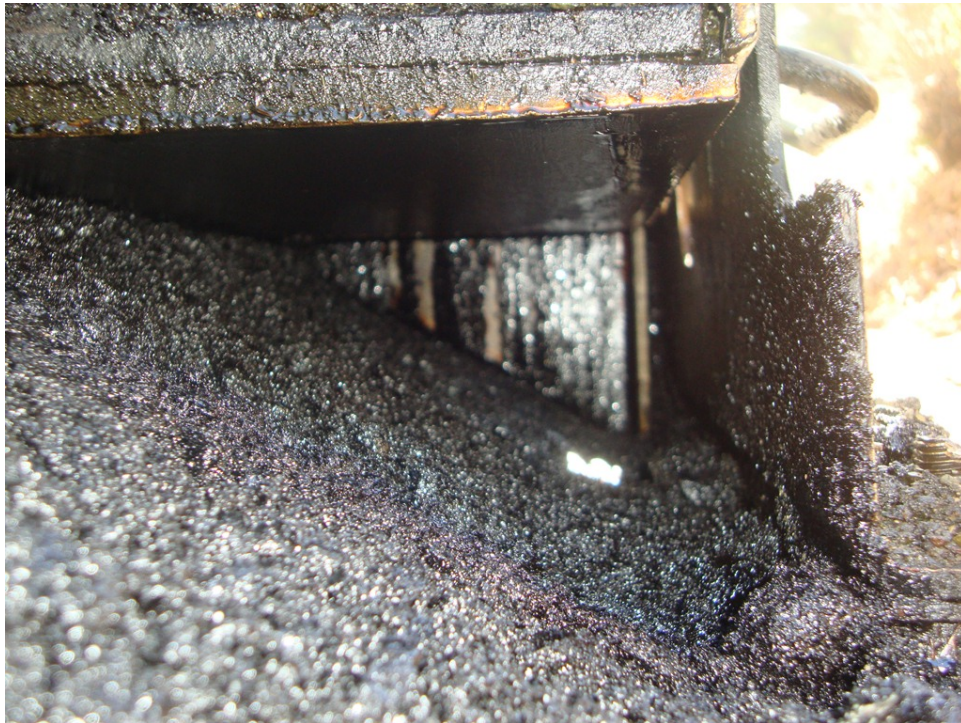
Figure 18. Safety Edge shoe of the Advantedge® device engaged onto the HMA to form the Safety Edge.
