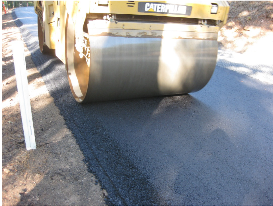
Figure 21. Breakdown steel drum vibratory roller compacting the HMA mat (edge pass with the drum typically about 2 in over the edge of the mat, although in some cases the drum was almost 12 in over the edge).
