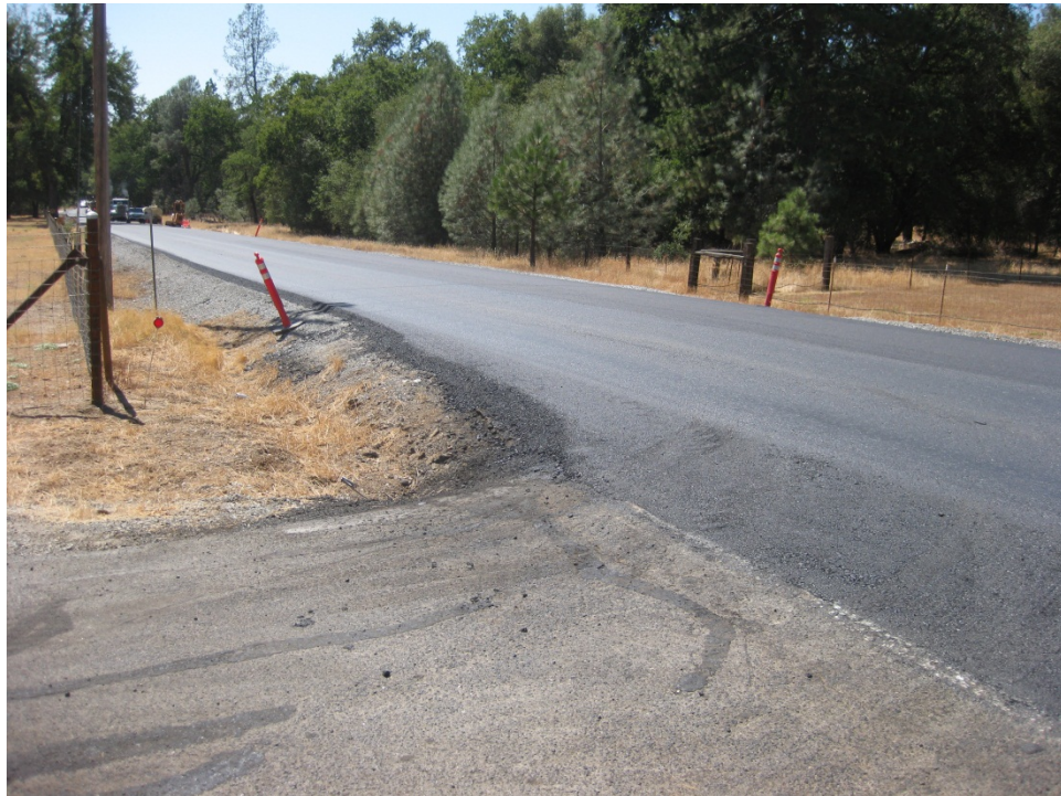
Figure 30. The Safety Edge shoe was raised when encountering driveways and cross streets.
