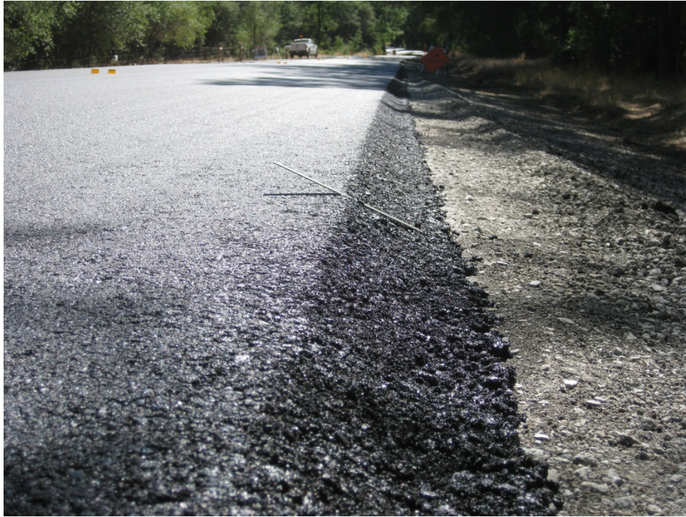
Figure 27. Typically formed Safety Edge on Mountain Ranch Road showing uniform break point and Safety Edge slope.
