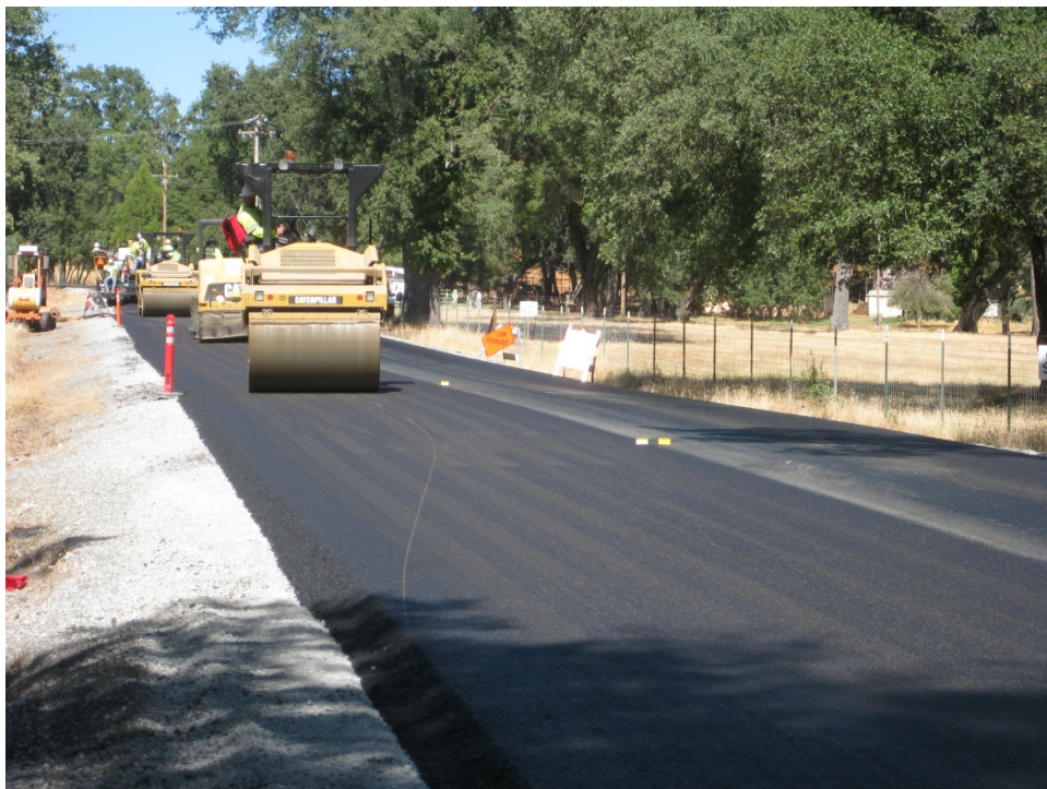
Figure 20. Three rollers used on the project to densify the 2-in HMA mat.
