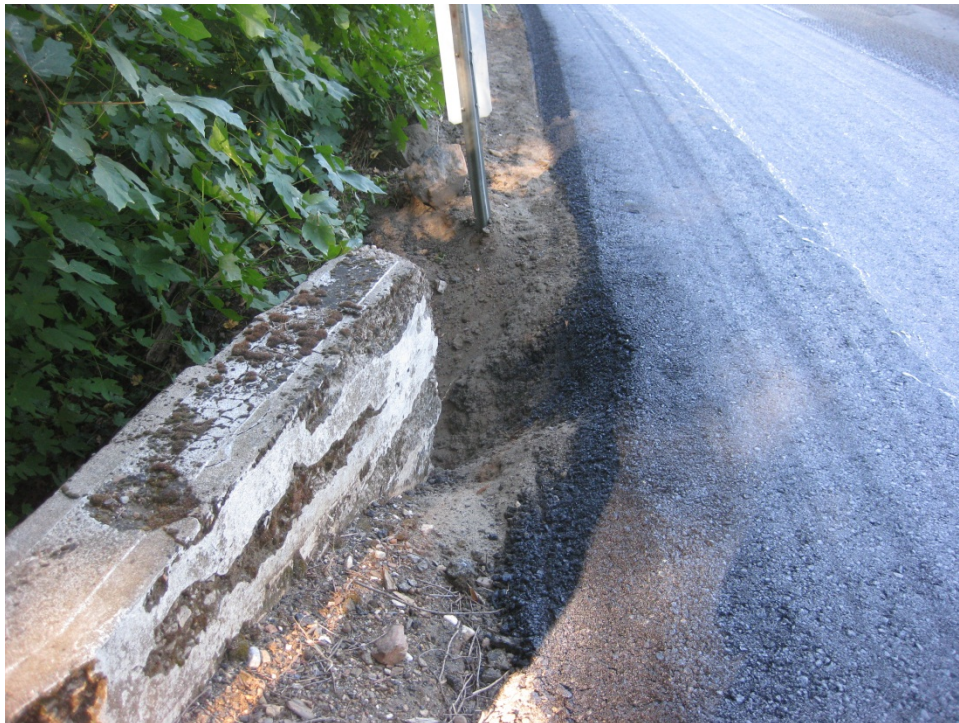
Figure 24. Small clearances between roadway edge and appurtenances such as culverts resulted in difficulty paving the Safety Edge consistently.
