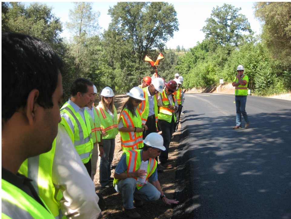
Figure 45. Ken Kochevar of FHWA explaining details of the Safety Edge during the field trip.
