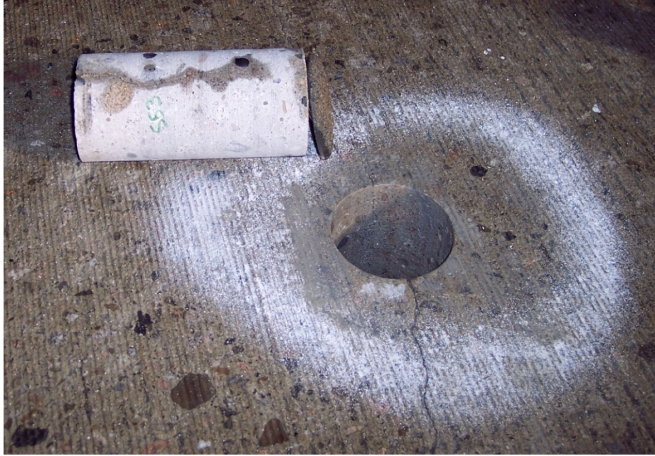
Figure 20. Cracked panel and core.
