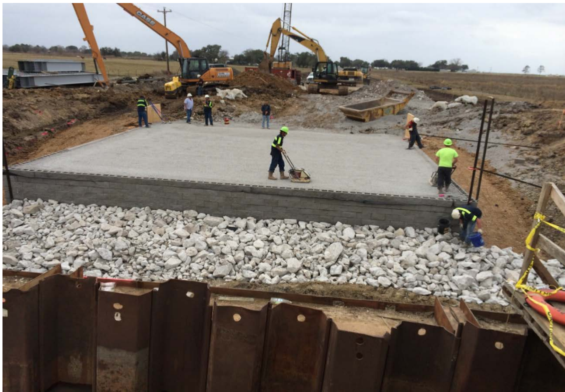
Figure 16. Photo. Installation of fifteenth row of blocks and completion of riprap of the face of wall (courtesy: LADOTD).
