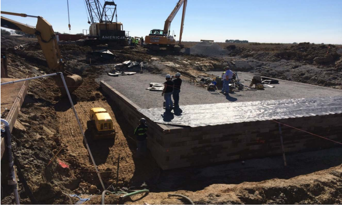
Figure 13. Photo. Installation of seventh row of blocks and backfill along the side walls (courtesy: LADOTD).
