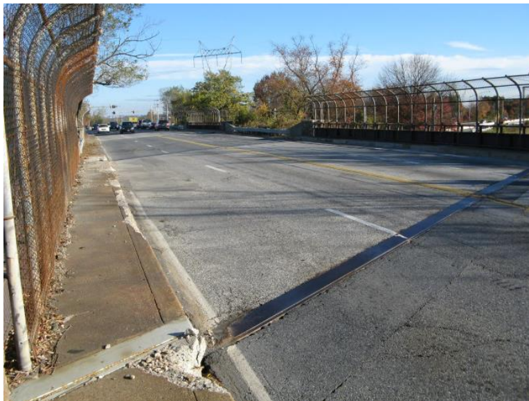
Figure 7. Sidewalk and deck deterioration.
