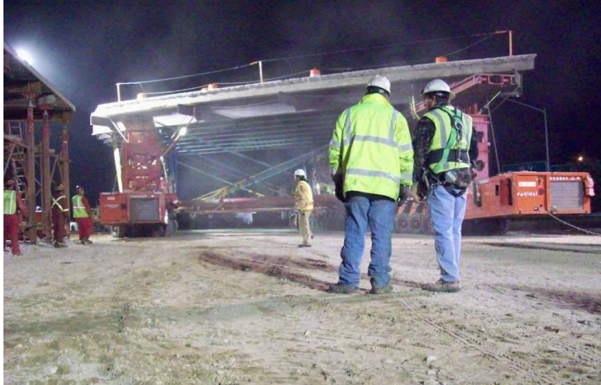
Figure 35. Old superstructure on MD 295 southbound being moved into place in the median.
