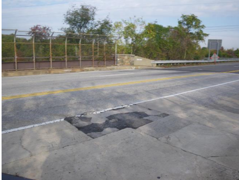
Figure 6. Extensive patches in bridge deck.
