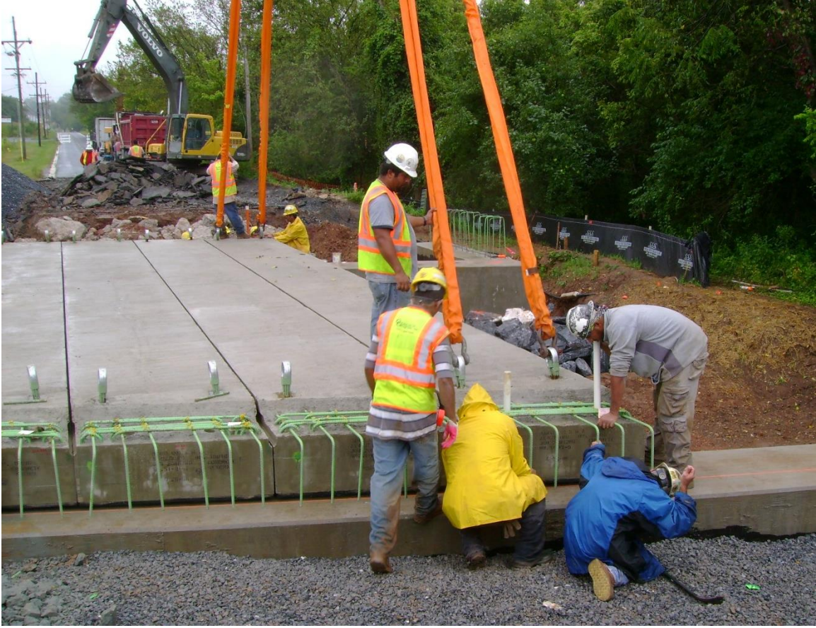
Figure 10. Alignment of elastomeric bearing pads for Slab No. 6 at MD 28 project.
