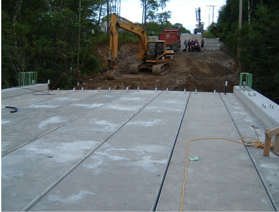
Figure 9. Looking eastbound on the Lamson Bridge Project across the top of the adjacent prestressed voided deck beams. The beams were post-tensioned transversely so the deck would act as a single unit (note the precast segmental retaining wall units on-grade in the background, next to the local residents who took interest in the construction progress).
