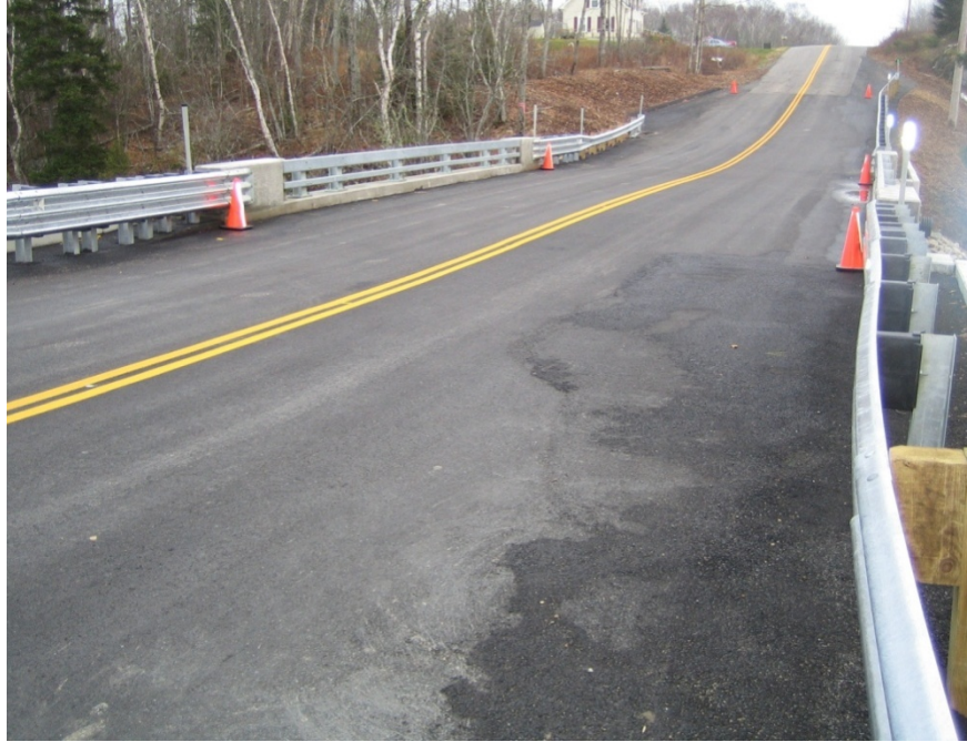
Figure 23. Finished Lamson Bridge pavement (note the irregularity in the right foreground).
