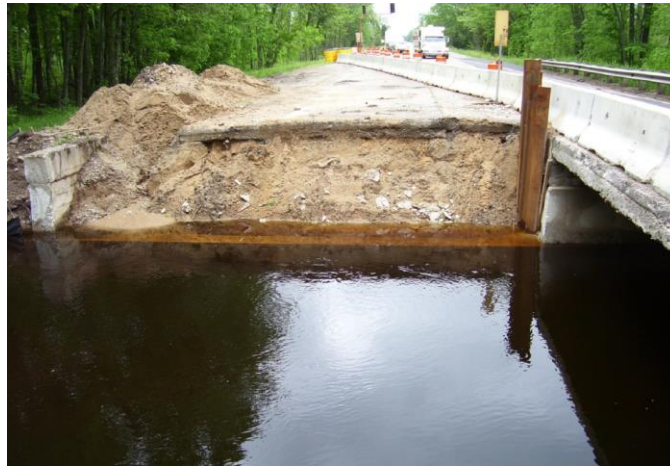
Figure 10. Removal of part of the old bridge with one-lane traffic on the rest of the bridge.
