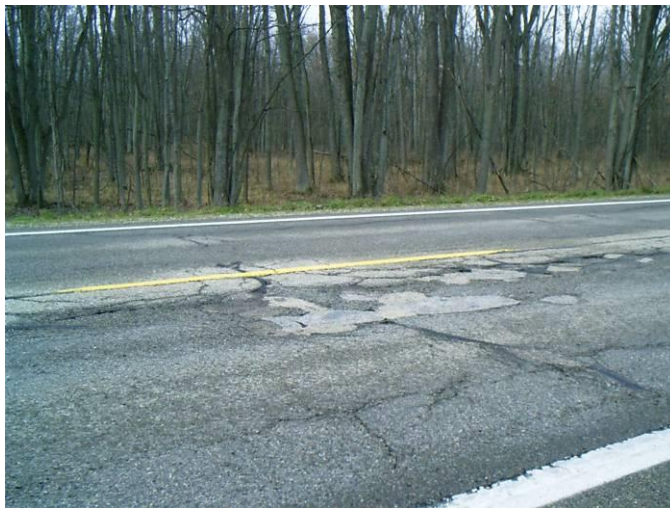
Figure 6. Typical delamination of HMA overlay.
