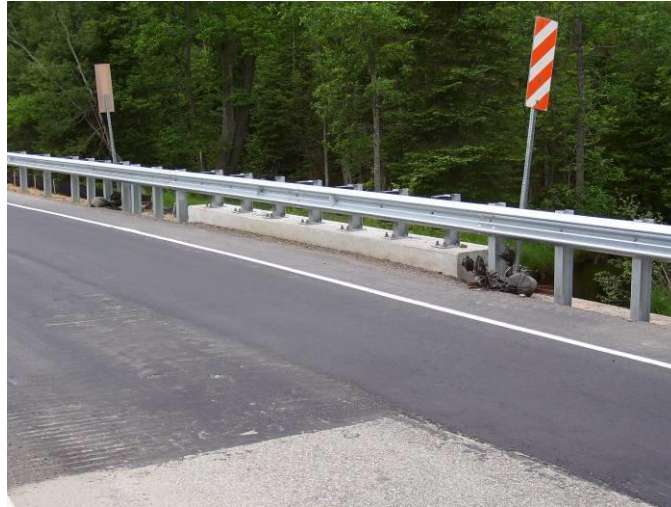
Figure 18. Completed placement of the bridge with AC shoulder before application of the HMA surface layers over the bridge.
