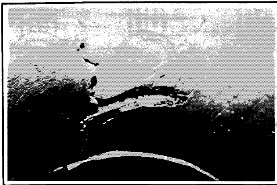
Exhibit 110. Severe longitudinal cracks with differential movement and spalling.
