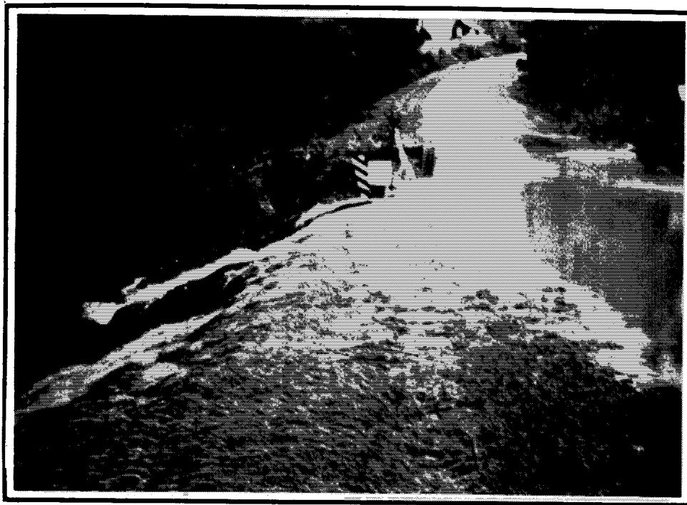
Exhibit 63. Culvert failure due to overtopping.
