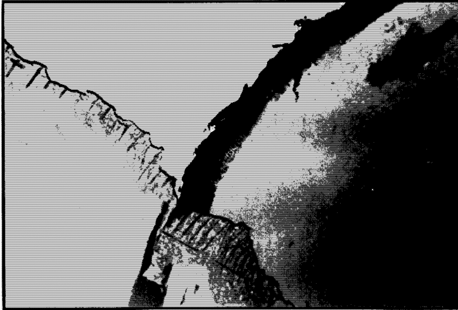
Exhibit 112. Spalling exposing reinforcing steel.
