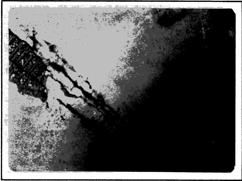
Exhibit 29. Reinforcing steel in concrete may corrode when exposed to water due to spalling or cracking.
