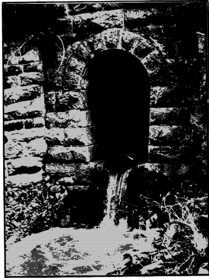
Exhibit 60. Scour at outlet of masonry culvert.
