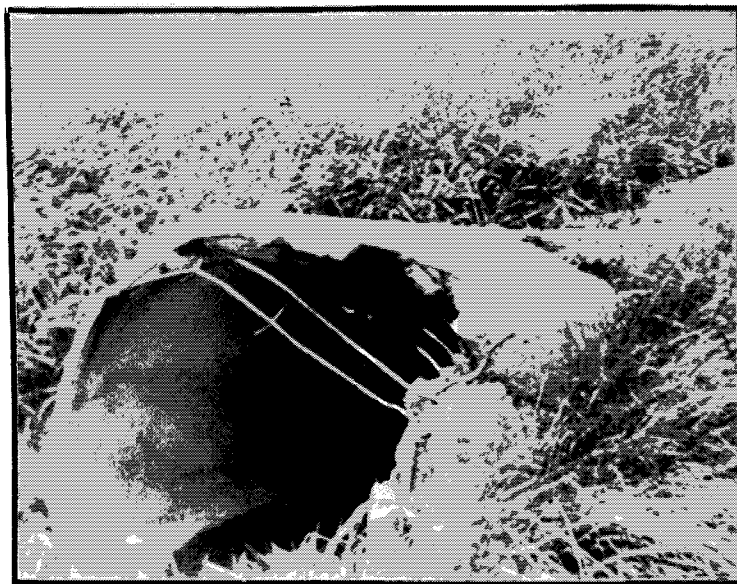
Exhibit 57. Impact damage to end of concrete pipe.
