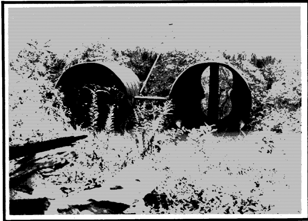
Pipes at same location as top photo require bracing to prevent excessive deflection. Bracing is a temporary measure until permanent repairs can be made.
