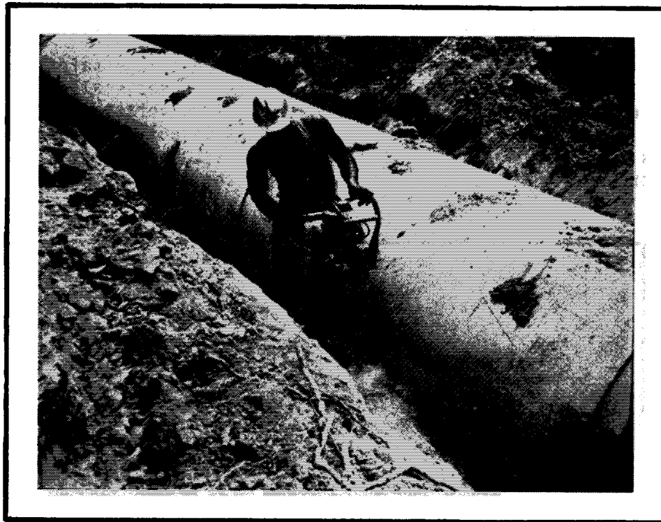
Exhibit 2. Attention to construction details such as compaction, bedding, and trench width is critical to proper culvert performance.
