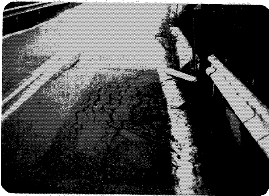
Exhibit 47. Pavement patches and pavement distress beside culvert. Distress is being caused by embankment spilling over wingwall.
