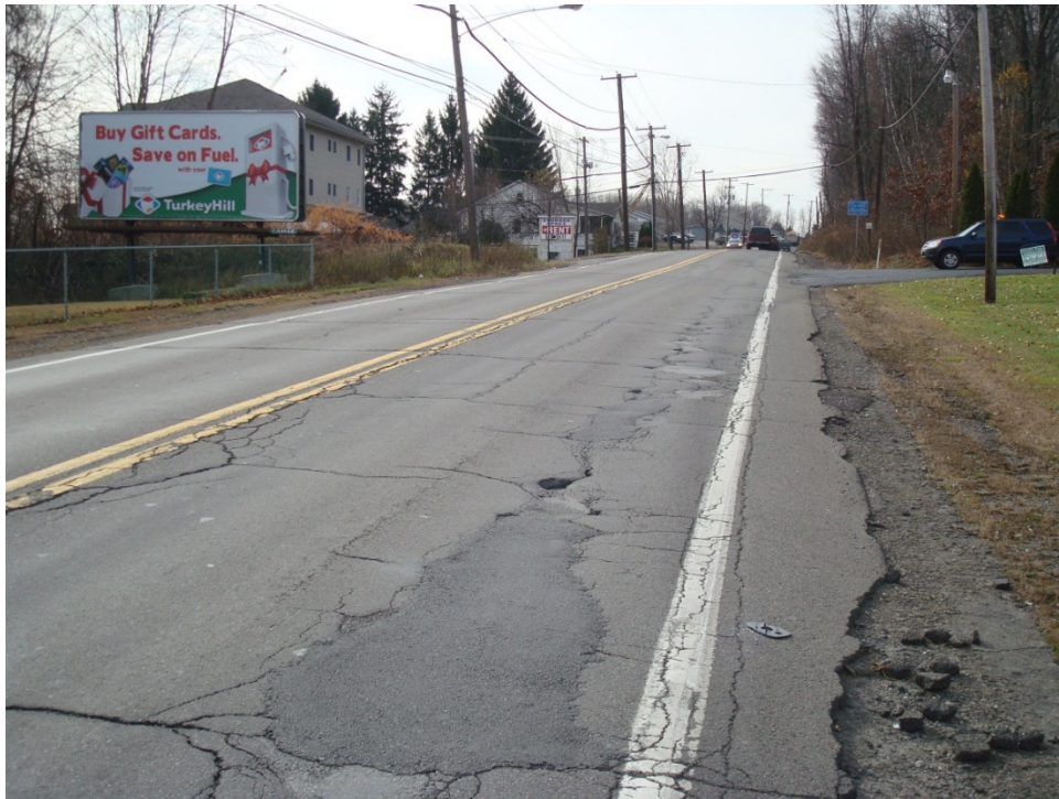
Figure 5. Photo. Close-up of existing roadway showing severe fatigue cracking and other distresses.
