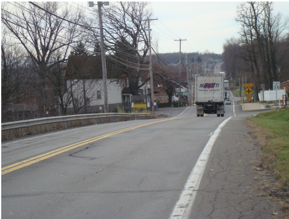
Figure 3. Photo. Existing roadway showing deterioration and truck traffic.
