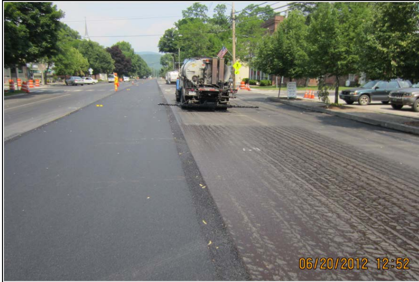
Figure 7. Tack coat (RS-1H emulsion) being applied to the surface of the leveling course before overlay placement.
