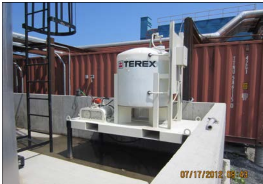
Figure 8. Terex foamer installed at the plant for producing foamed WMA.
