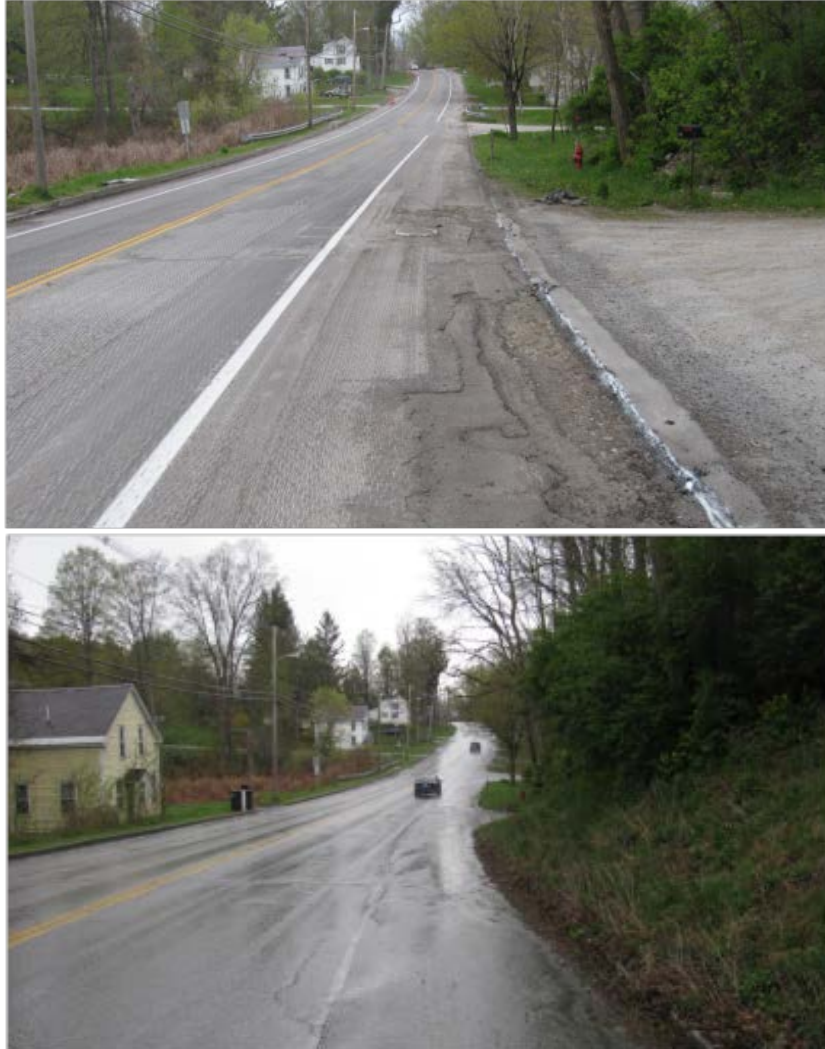
Figure 4. General view of pavement condition in two areas of the project before rehabilitation on U.S. 4A near Castleton. Condition of the other segments was similar. (Photos courtesy of Chris Thomas, Peckham Construction.)
