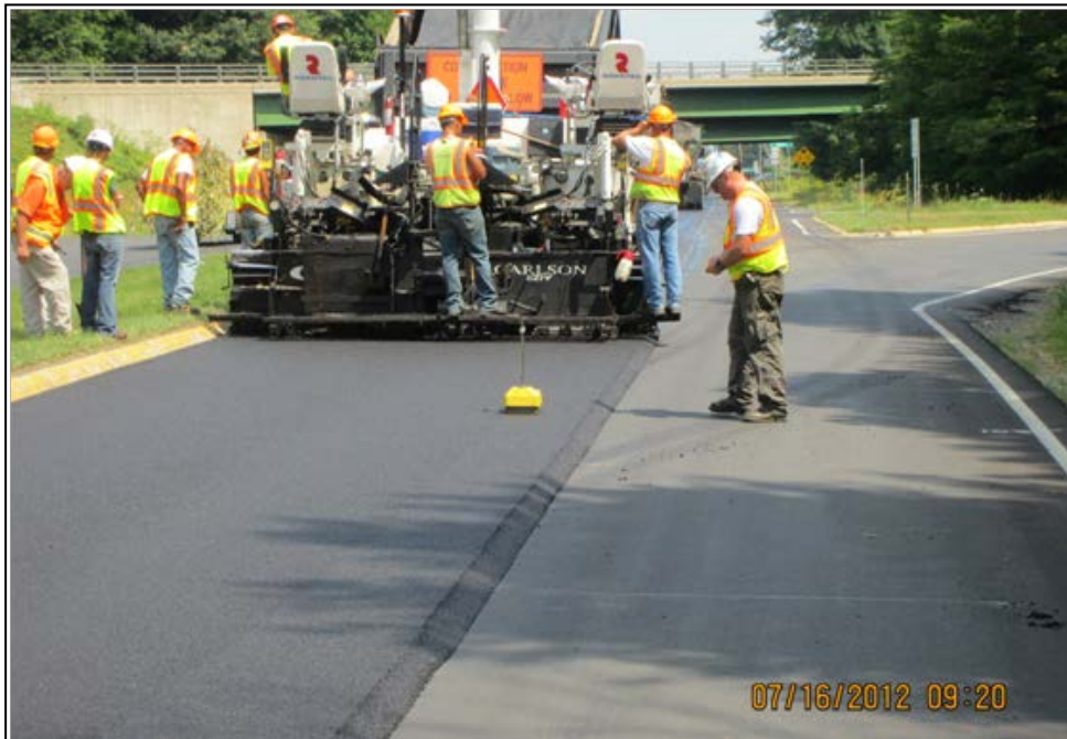
Figure 20. QC personnel taking density readings in the control strip with a nuclear density gauge.
