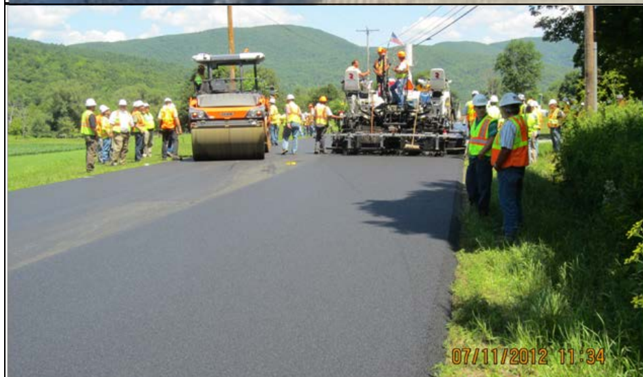
Figure 38. Field visit to showcase the paving and compaction operations along U.S. 4A.
