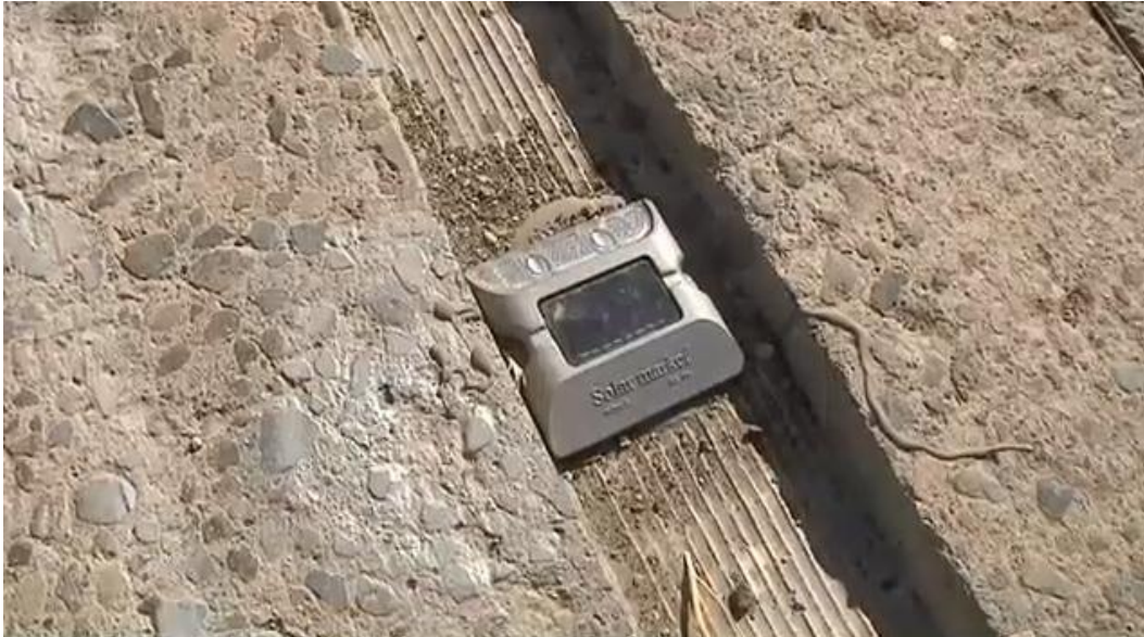
Figure 13. Photo. RPM style LED delineator installed on I-90.
