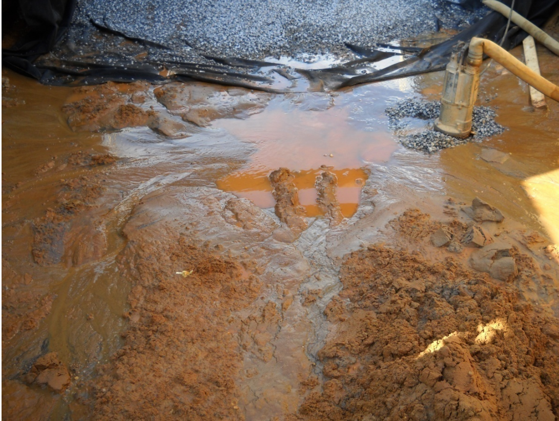
Figure 12. Saturated subgrade conditions.
