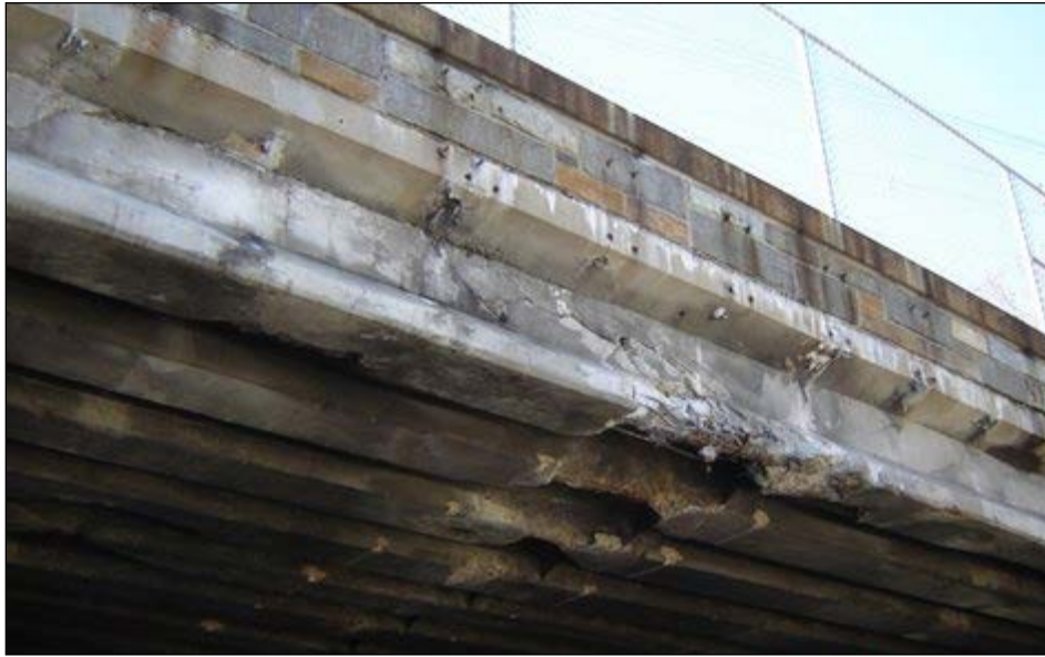
Figure 3. View of vehicular damage to the bridge beams.
