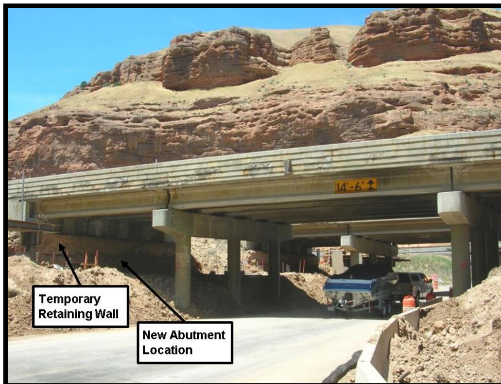
Figure 3-2 Three-Span Overpass Bridge Converted to a Single-Span on the I-80 Echo Road Bridge Project (Before)
