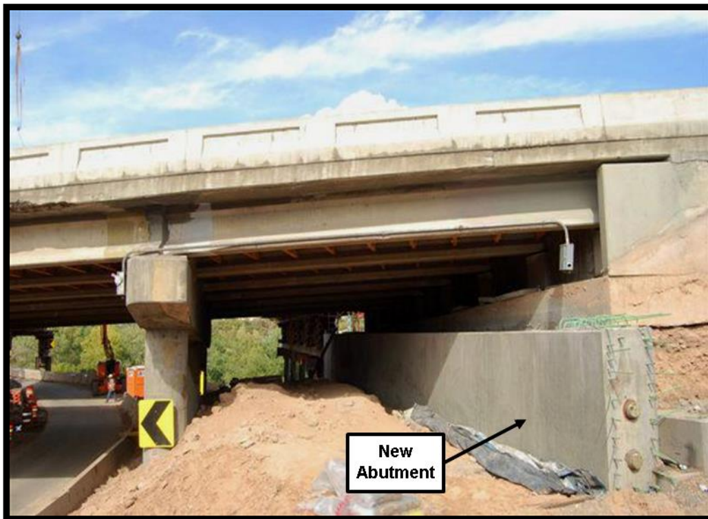
Figure 3-7 New Abutment Constructed under Existing Structure for the I-80; 2300 E. Bridge Slide, Utah
