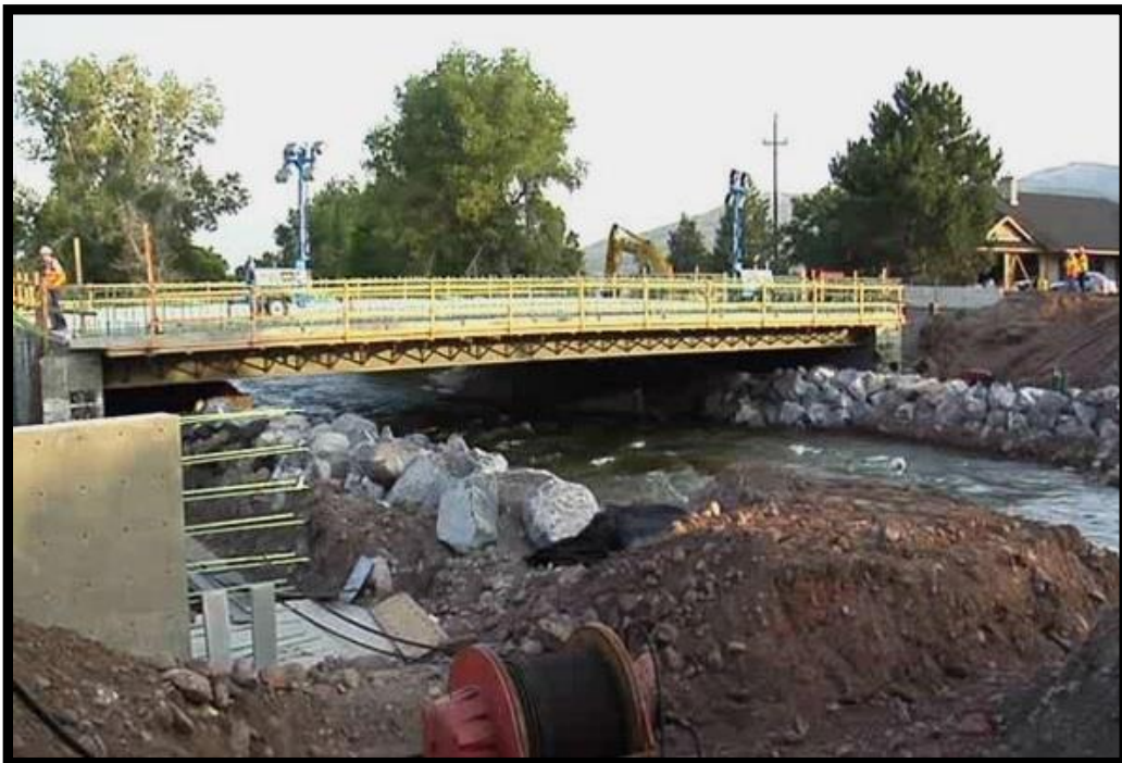
Figure 1-4 SIBC for a Small Stream Crossing for the SR-66 over Weber River Bridge Project, Utah
