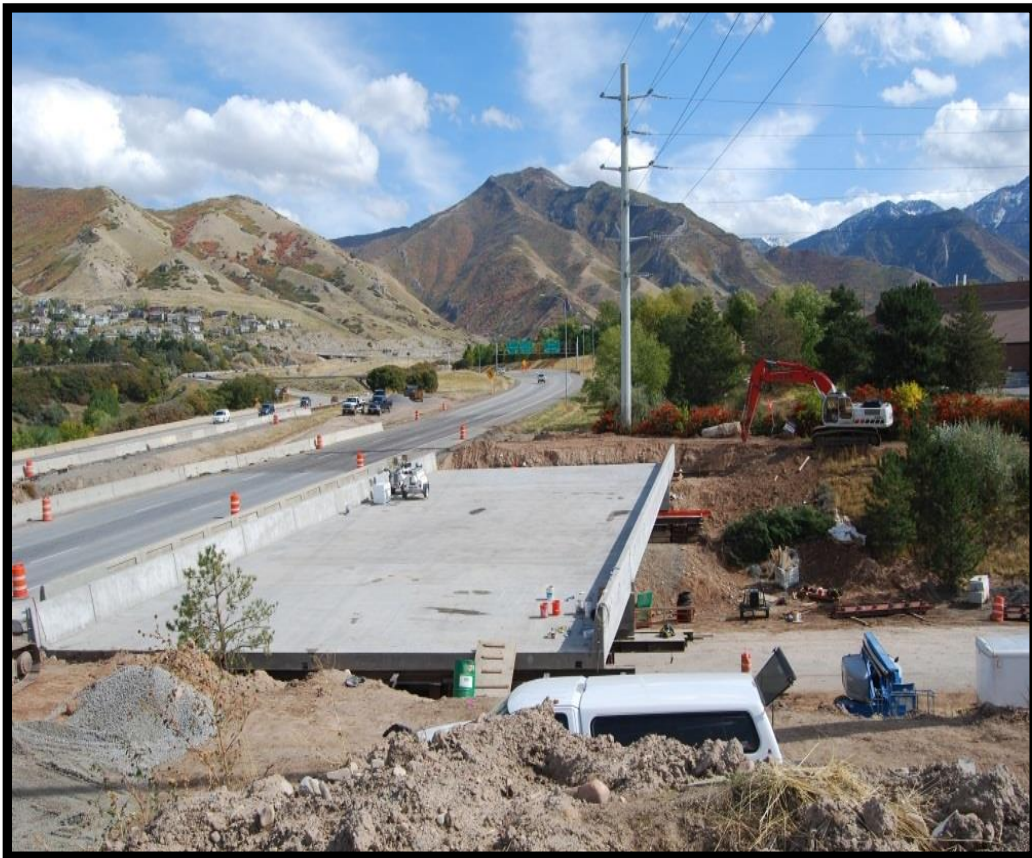
Figure 2-1 SIBC that Avoided Use of Temporary Crossovers on I-80; 2300 E. Bridge Project, Utah
