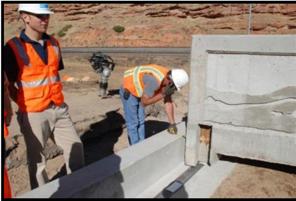
Figure 3-13 Inverted “T” Precast Sleeper Slab on the I-80 Echo Road Bridge Project, Utah
