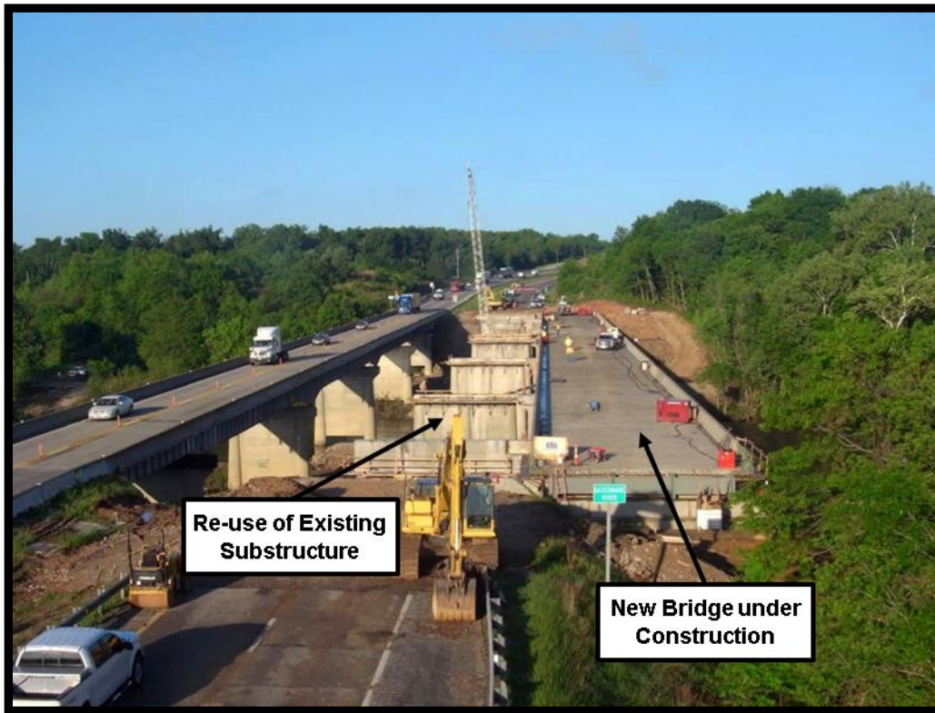
Figure 3-10 SIBC Using Existing Substructure on the I-44 Gasconade River Bridge Project, Missouri
