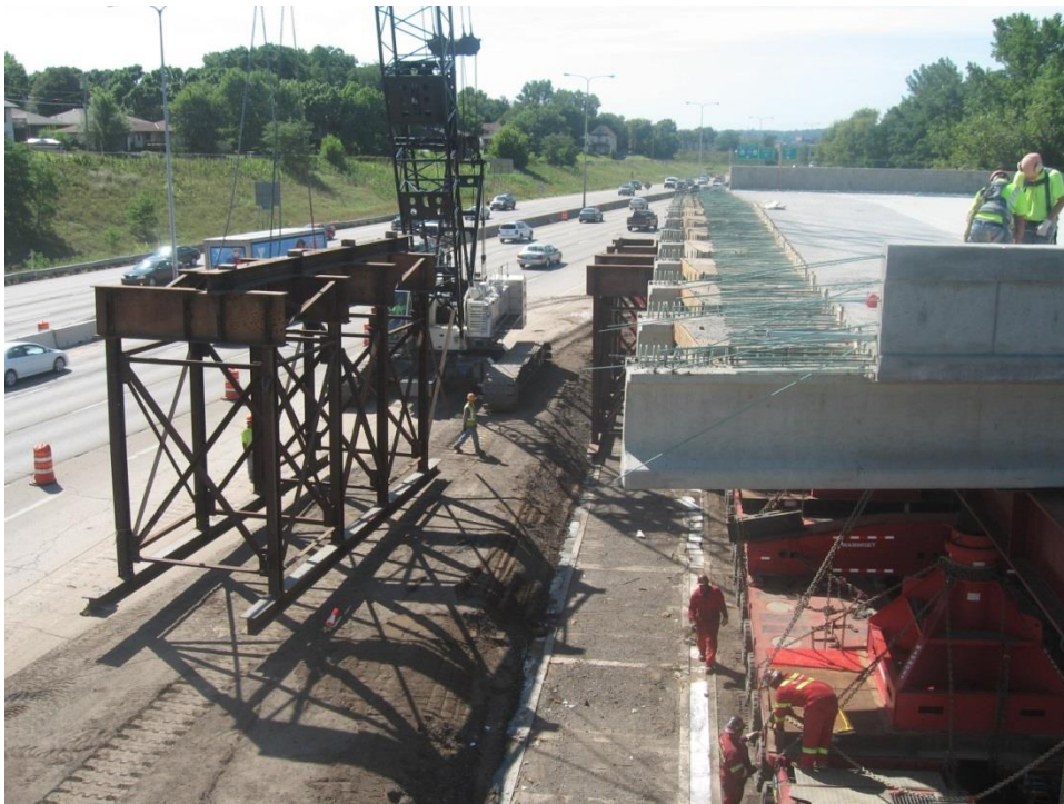
Figure 65. Photo. The falsework was removed after the bridge was fully supported by the SPMT to clear the path for the SPMT move.
