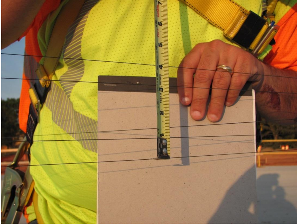
Figure 64. Photo. Strategically placed stringlines were used during lifting, moving, and placement of the spans to ensure that deflections and torsions of the span were within tolerance.
