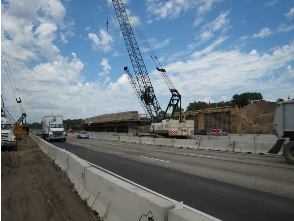
Figure 48. Photo. Medium-shot view of the construction of the abutments and midspan pier with traffic lanes open on I-35E.
