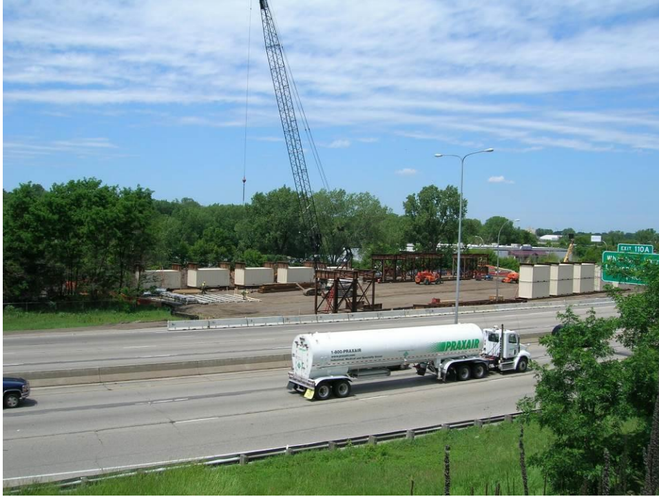
Figure 13. Photo. Long-shot view of construction of the falsework at the bridge staging area to support bridge 62626 superstructure.
