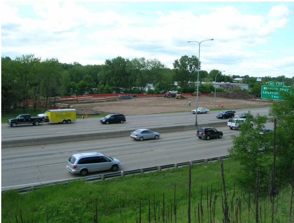
Figure 9. Photo. Long-shot view of staging area for bridge 62626 superstructure construction alongside southbound I-35E.
