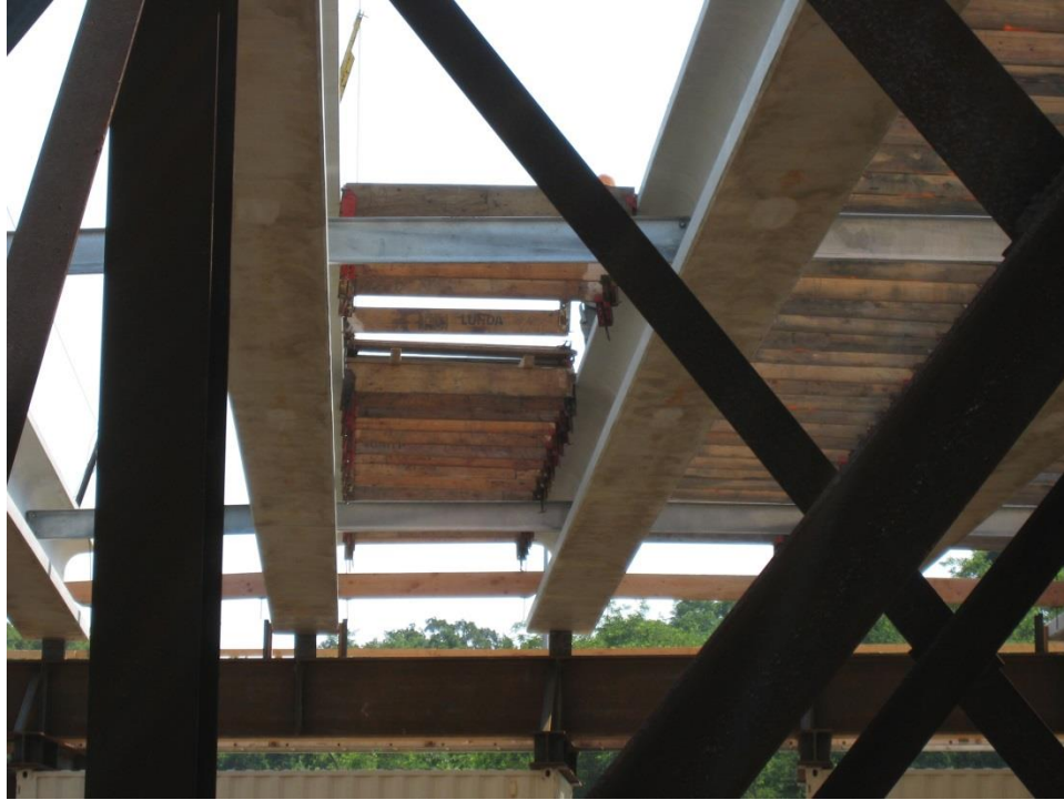
Figure 25. Photo. Setting the wooden support beams on the the concrete girders prior to placement of the wooden forms for the deck concrete.
