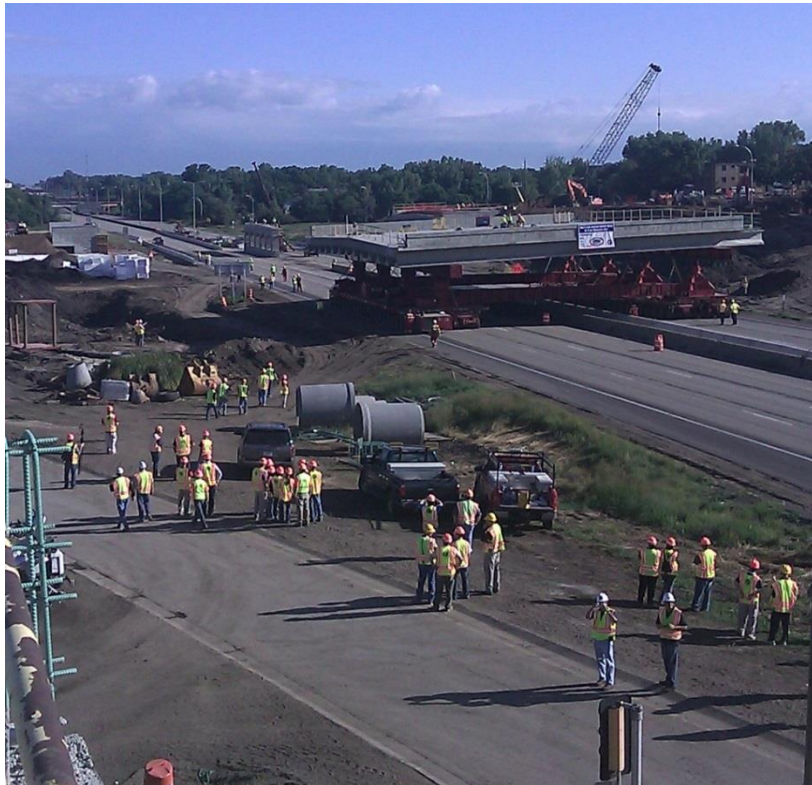
Figure 77. Photo. Many members of the public, as well as representatives from MnDOT and other Federal and State transportation agencies, witnessed the replacement process.
