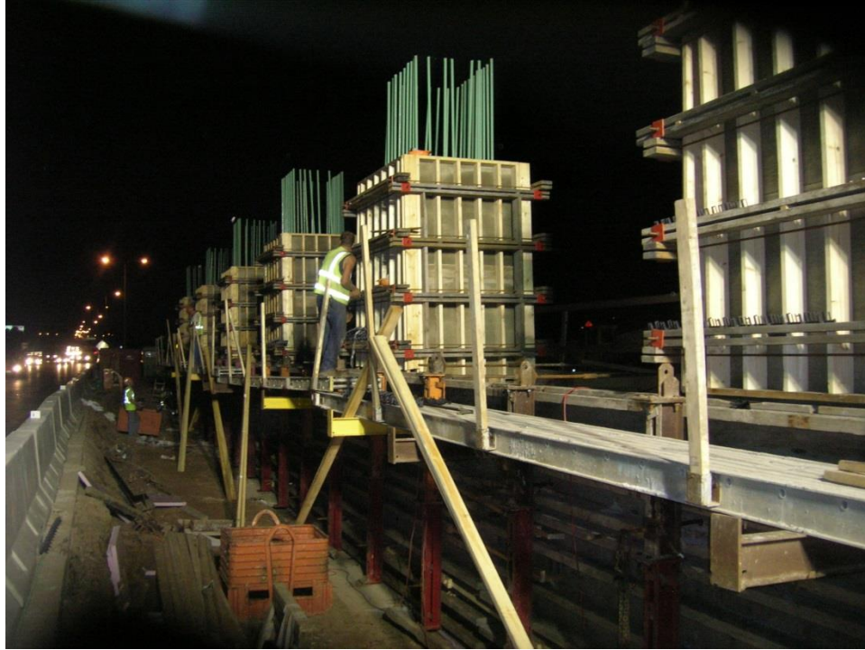
Figure 46. Photo. Constructing the CIP crash wall and support columns for the midspan pier in the median of I-35E with lanes open to traffic.
