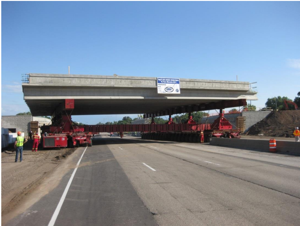
Figure 67. Photo. Moving the first span of Maryland Ave. bridge 62626 on I-35E using the SPMT.
