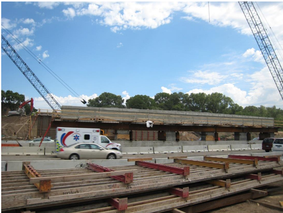
Figure 49. Photo. Close-up view of the construction of the midspan pier with traffic lanes open on I-35E.
