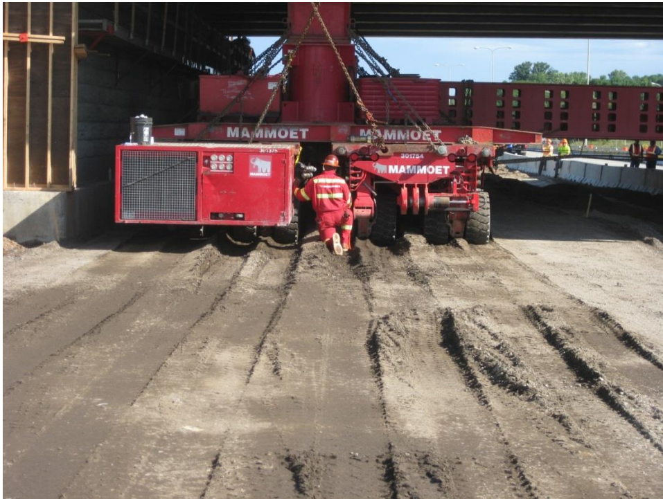
Figure 75. Photo. During placement of the first span, some of the SPMT wheels dug into the soft soil between the abutment and the roadway, resulting in some difficulty moving the SPMT.
