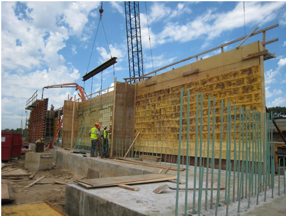
Figure 51. Photo. Erecting the reinforcing steel and forms for the construction of the CIP west abutment wall. Note the stamped texture on the forms for aesthetics of the inside wall face.
