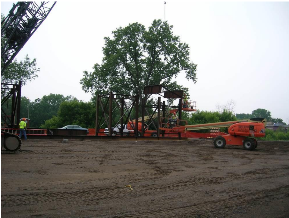
Figure 12. Photo. Medium-shot view of construction of the falsework at the bridge staging area to support bridge 62626 superstructure.
