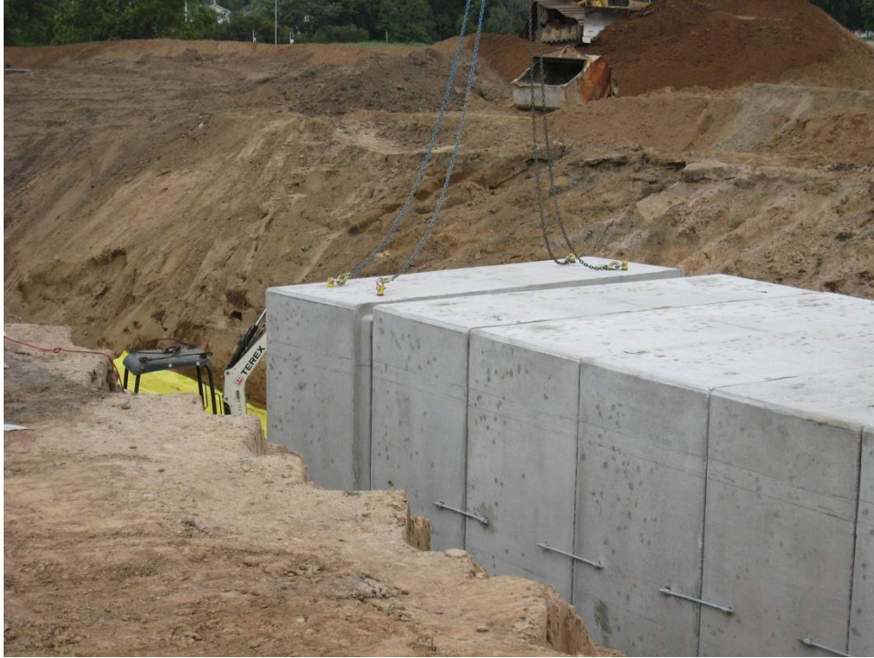
Figure 55. Photo. Placing the individual prefabricated sections for the box culvert bridge tunnel beneath Maryland Ave.
