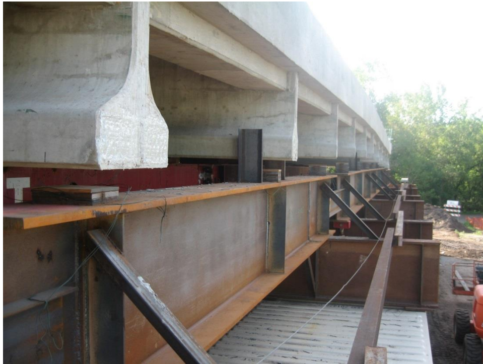
Figure 63. Photo. The superstructure span was first lifted off the bearing pads on top of the falsework.
