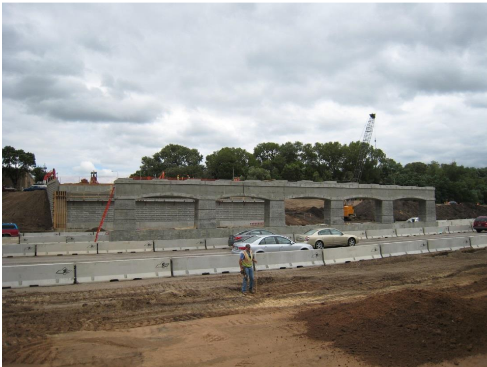
Figure 53. Photo. Medium-shot view of the completed midspan pier in the foreground and the east abutment wall in the background after removal of the forms.
