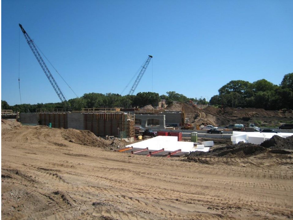
Figure 52. Photo. Long-shot view of the two abutments and the midspan pier after concrete placement.
