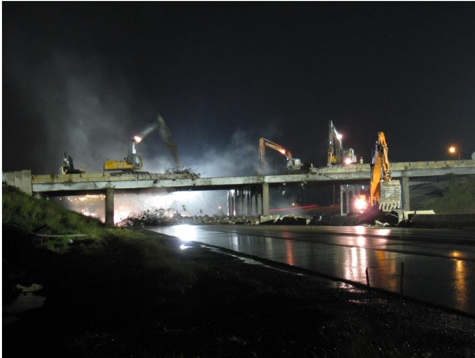
Figure 41. Photo. Demolishing Maryland Ave. bridge 6513 as seen from I-35E. The bridge was demolished over a weekend closure of I-35E, while traffic was diverted through the Maryland Ave. off- and on-ramps.
