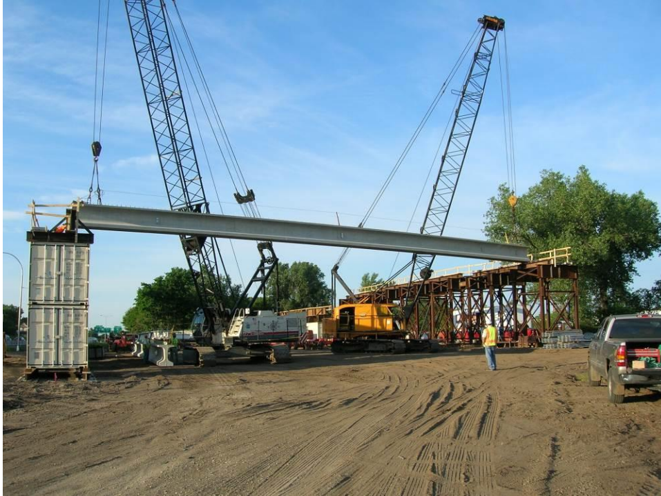
Figure 15. Photo. Two cranes were used to hoist each girder onto the falsework.
