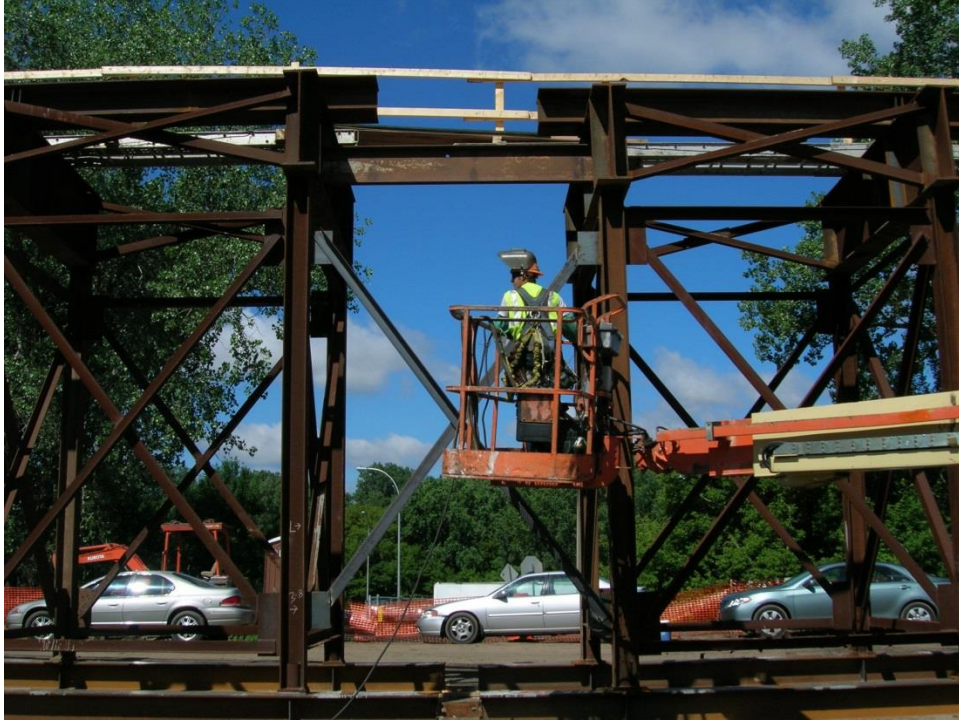
Figure 11. Photo. Close-up view of construction of the falsework at the bridge staging area to support bridge 62626 superstructure.
