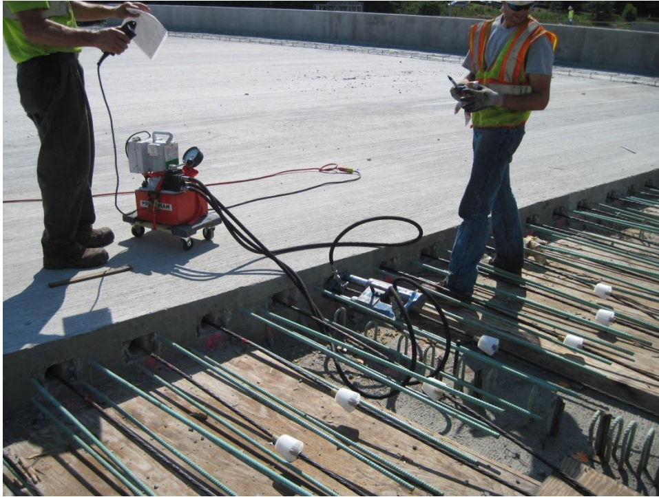
Figure 37. Photo. Stressing the post-tensioning cables to precompress the span prior to moving it using the SPMT.
