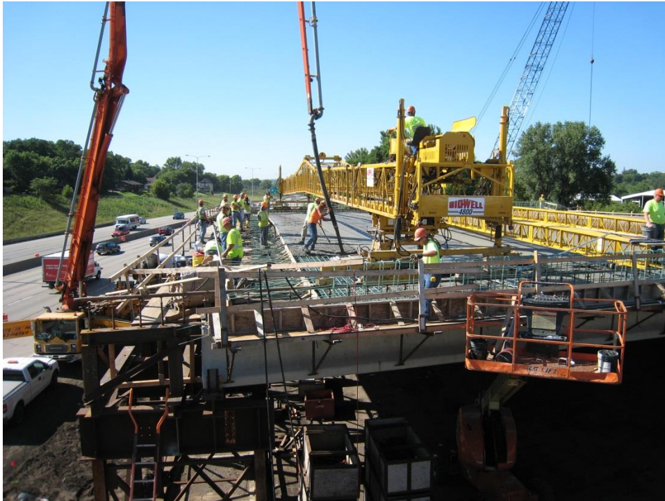
Figure 32. Photo. The fiber-reinforced concrete was pumped from the roadway below on to the prepared bridge deck surface and the paving was done using a Terex® Bid-Well 4800 roller paver.
