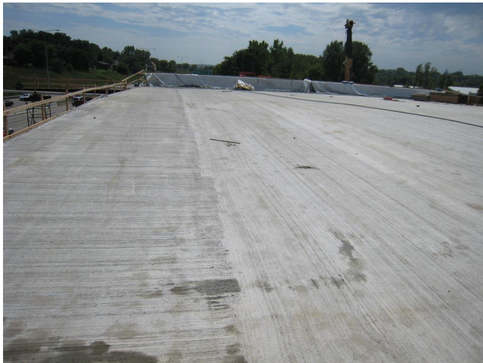
Figure 36. Photo. Finished and cured bridge deck surface after removal of the polyethylene sheets.
