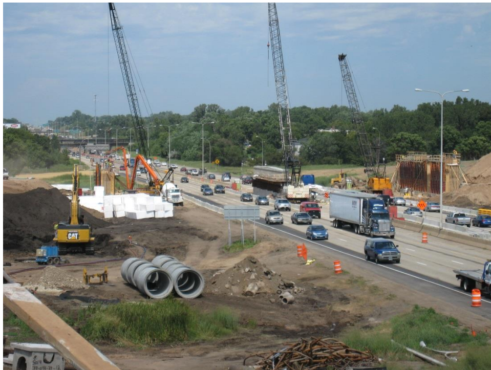
Figure 47. Photo. Long-shot view of the construction of the abutments and midspan pier with traffic lanes open on I-35E. This view is from the top of the new bridge 62626 concurrently being constructed alongside the roadway.
