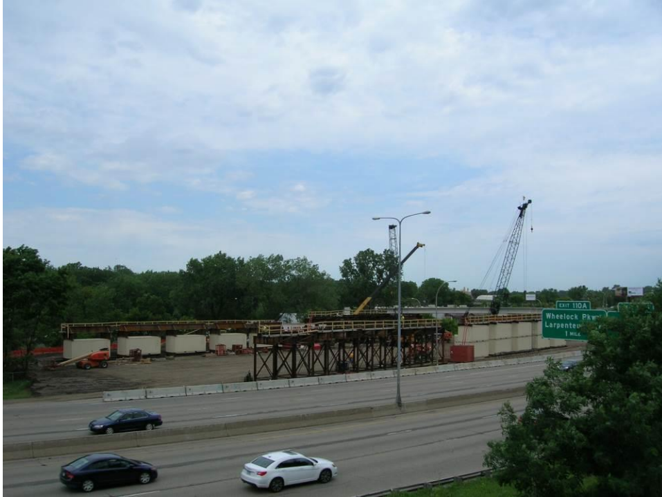
Figure 17. Photo. Long-shot view of hoisting girders onto the falsework at the bridge superstructure staging area.
