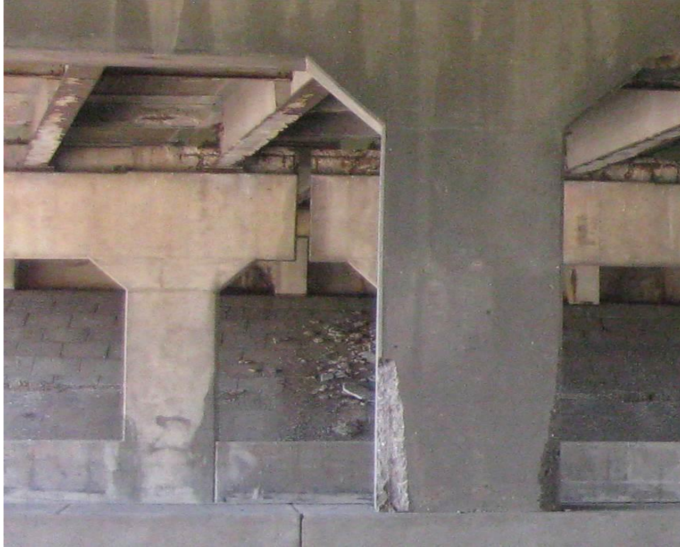
Figure 4. Photo. Fallen debris from end bent cap and column spalling on bridge 6513.
