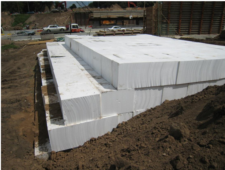
Figure 58. Photo. EPS-block geof foam was used for the west embankment fill to reduce bearing pressure on the subsoil to control settlement and minimize excavation.
