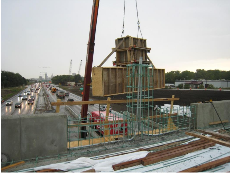
Figure 81. Photo. Setting the reinforcing steel and forms for the closure pour of the barrier wall after the closure pour of the 15-ft transverse joint opening between the two spans.
