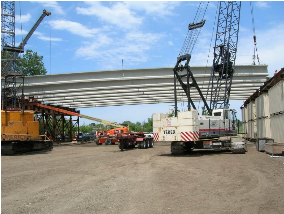
Figure 16. Photo. Hoisting girders onto the falsework at the bridge superstructure staging area.
