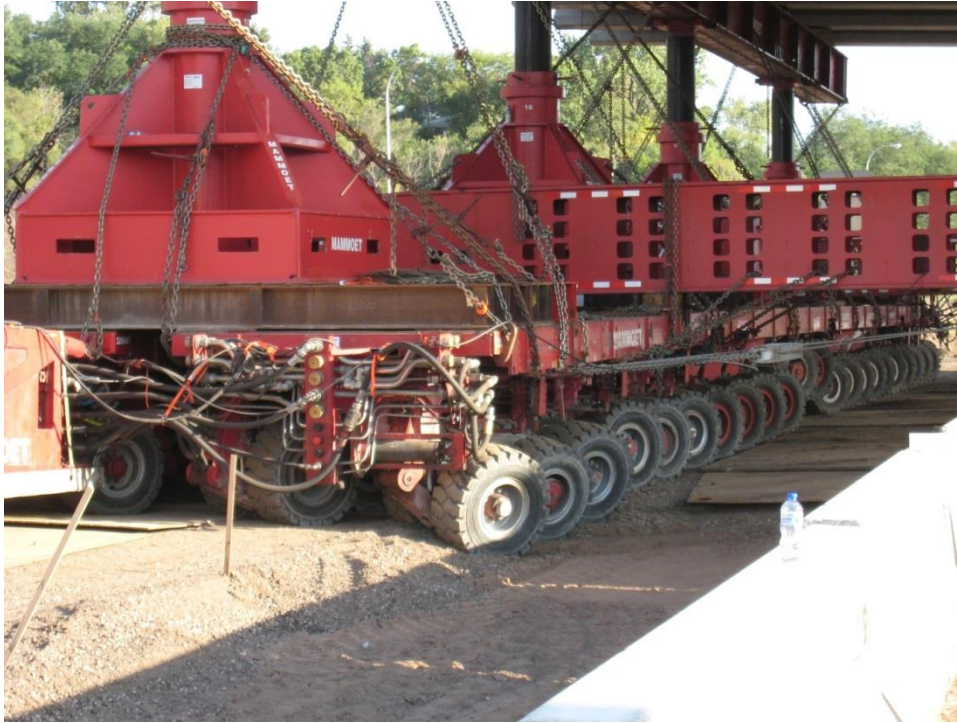
Figure 66. Photo. The SPMT easily handled the grade difference between the bridge staging area and I-35E during the move to the final location. All movements measured using the stringlines were within specifications.
