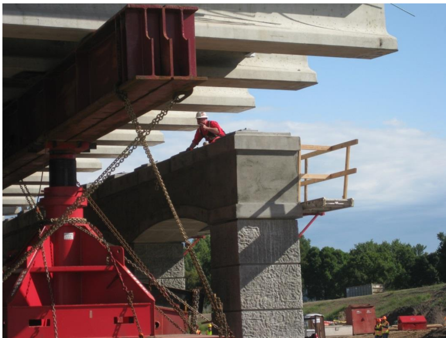
Figure 69. Photo. The vertical and horizontal positions of all girders of the span were carefully monitored from the pier to ensure that it was lowered uniformly so as to not excessively stress the girders, deck, and pier columns, which could potentially cause cracking or other distresses.
