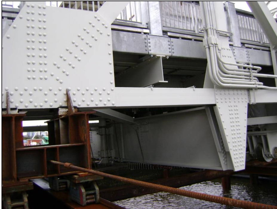
Figure 3. Closeup of the rivet head bolts.
