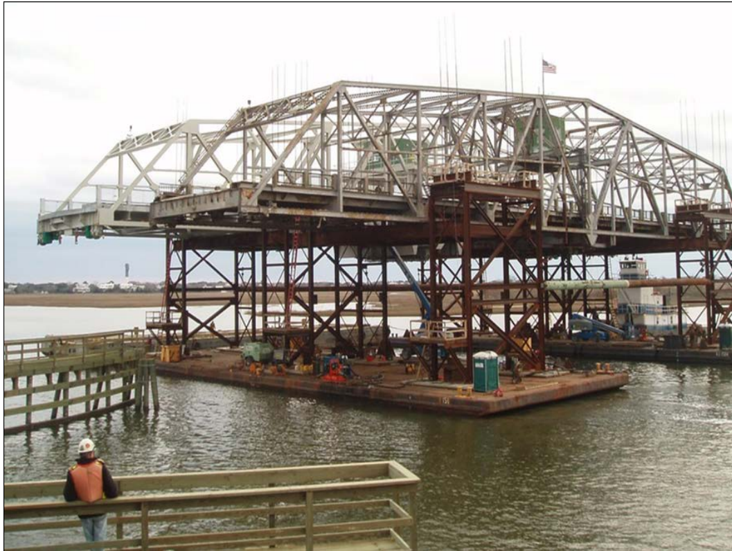
Figure 12. Existing and new swing spans shown side by side on supporting barges.
