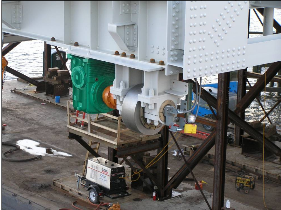
Figure 10. New swing span machinery.
